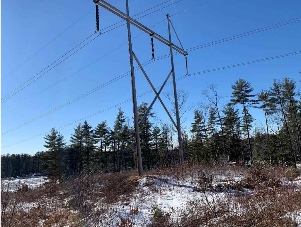
Photograph No. 19: Looking westerly at proposed pad location for 373 Structure 276 to be replaced.
