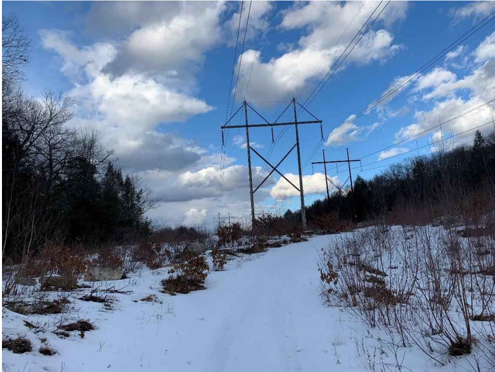
Photograph No. 7: Looking northerly at proposed access towards 373 Structure 299 to be replaced.
