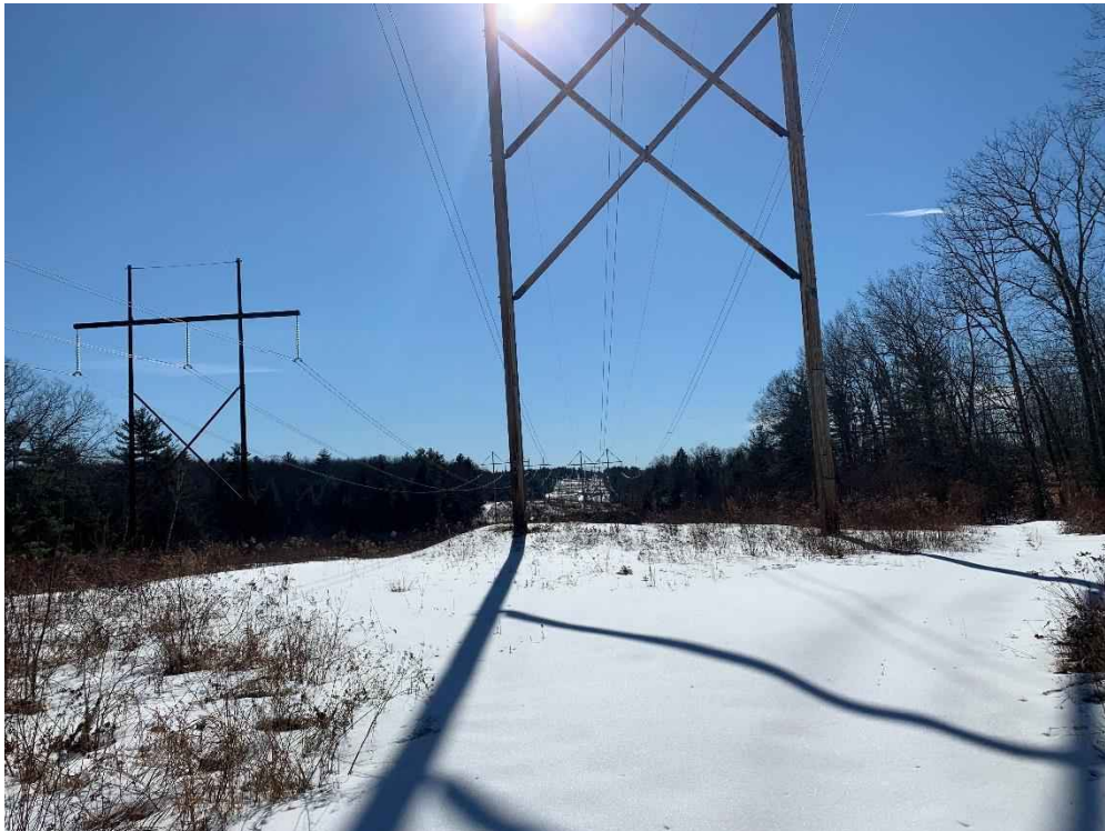
Photograph No. 10: Looking southerly at proposed access and work pad location for 373 Structure 296 to be replaced.
