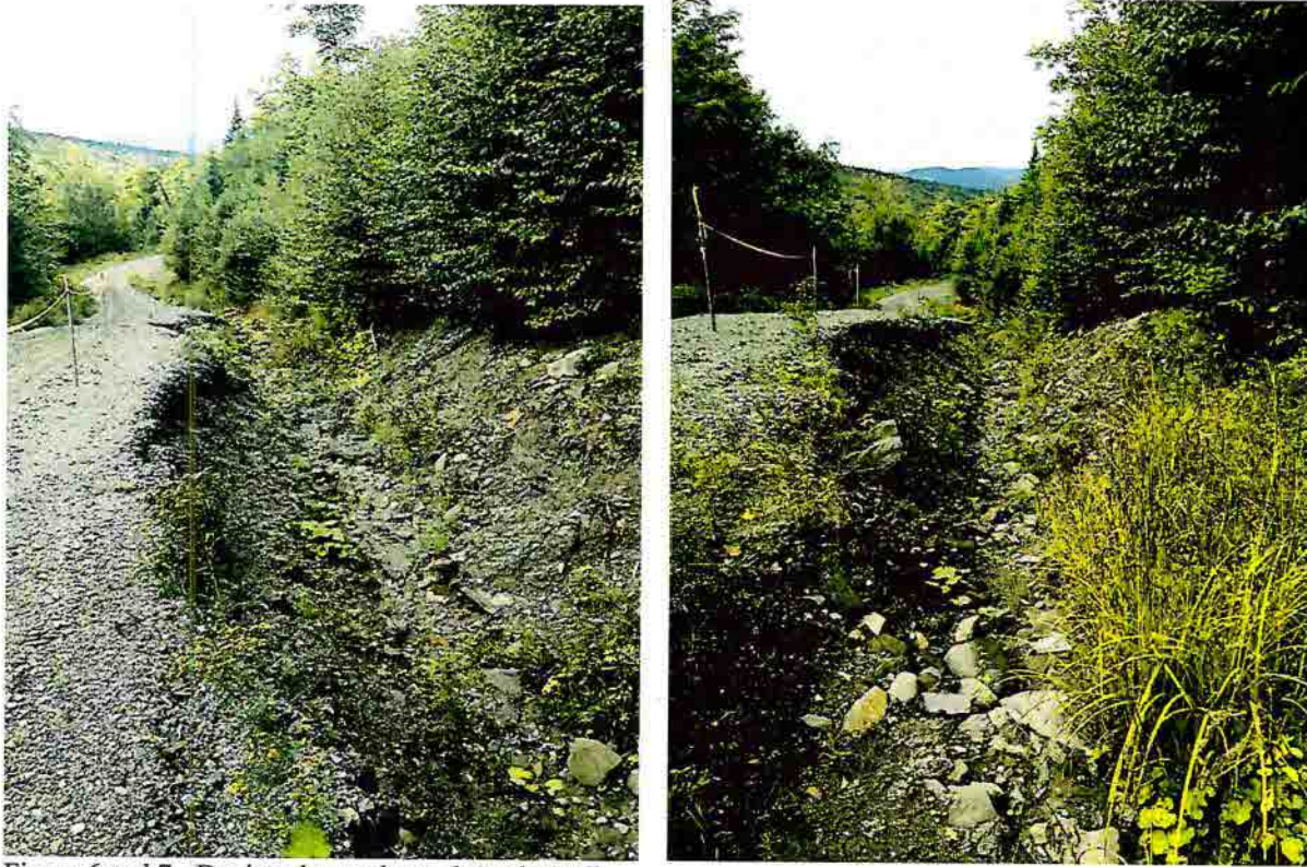
Figure 6 and 7- Depicts the washout along the trail.
