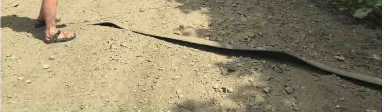
Ineffective Water Bar
