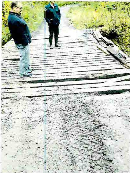
Figure 10- Depicts the repaired approach to the bridge, however, still shows the decking that needs replacing.
