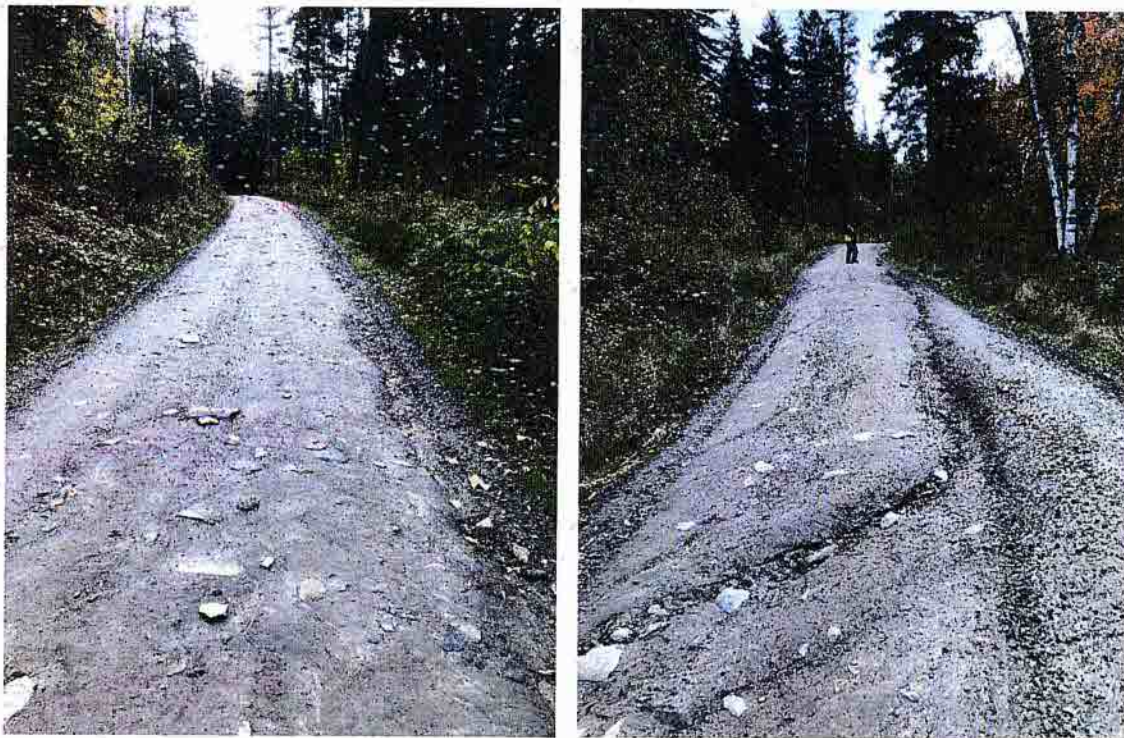
Figure 3- Shows condition of trail
