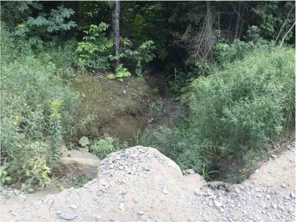
New Gravel covering Erosion
