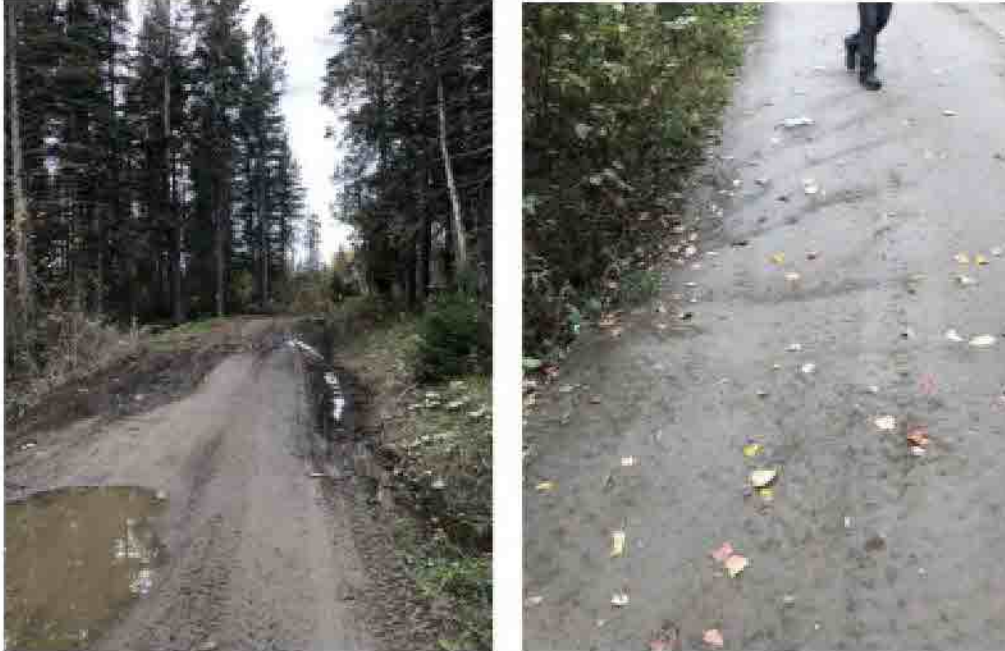
Figure 4- Mud on trail and ATV tracks in ditch and minor sedimentation on trail from water.
