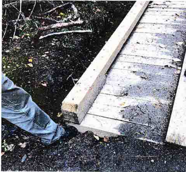
Figure 2- Minor sediment washing on edge of bridge
