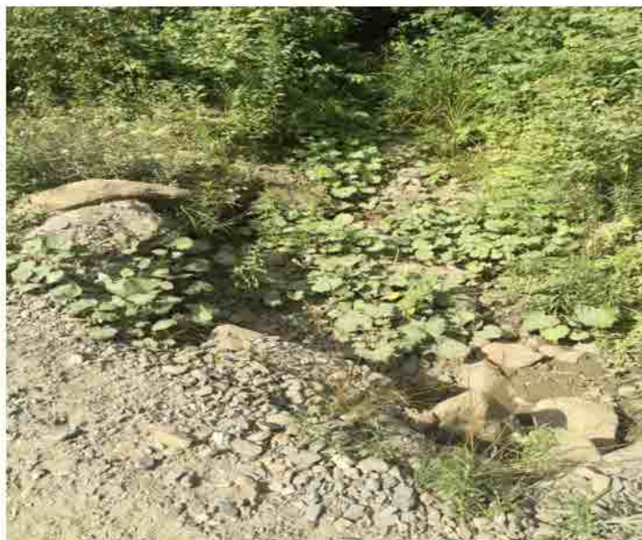
Drainage ditch with erosion and dust
