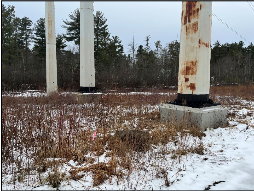
Photo 11: View of proposed timber matting location near Structure 187 off Cate Road in Deerfield.
