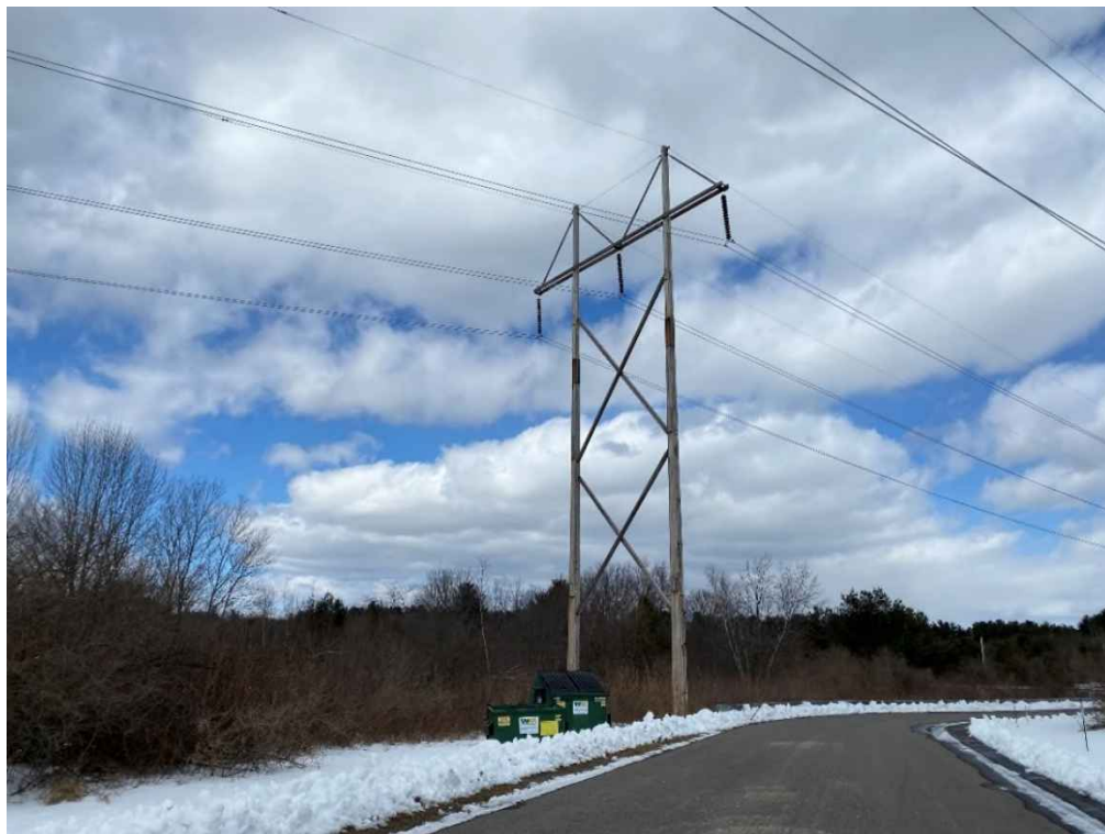
Photograph No. 6: Looking at proposed work pad location adjacent for Structure 61 of the 380 Line from Driveway A504.
