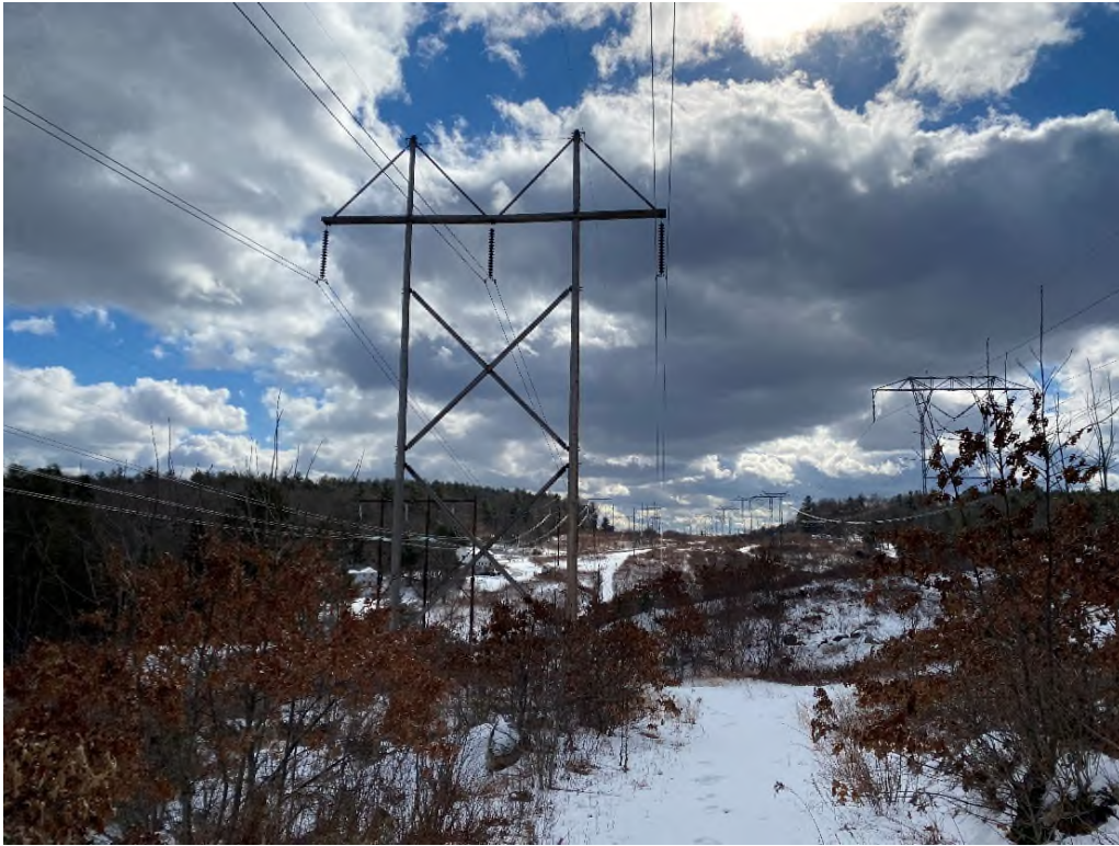
Photograph No. 17: Looking at proposed access and work pad location for Structure 80 of the 326 Line.
