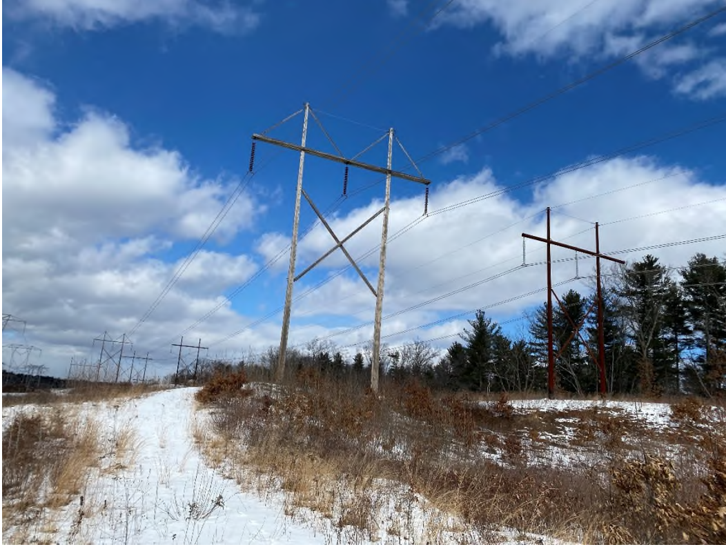
Photograph No. 13: Looking at work pad location for Structure 72 of the 326 Line.
