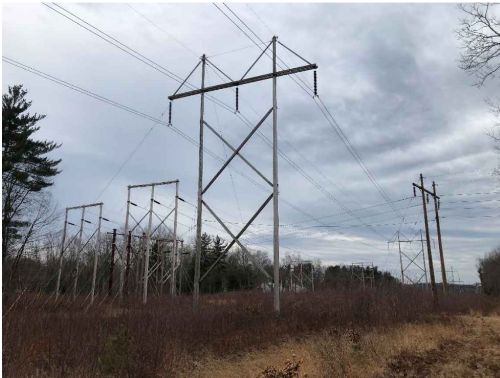
Photograph No. 2: Looking at proposed access and work pad location adjacent to Structure 85 of the 380 Line.
