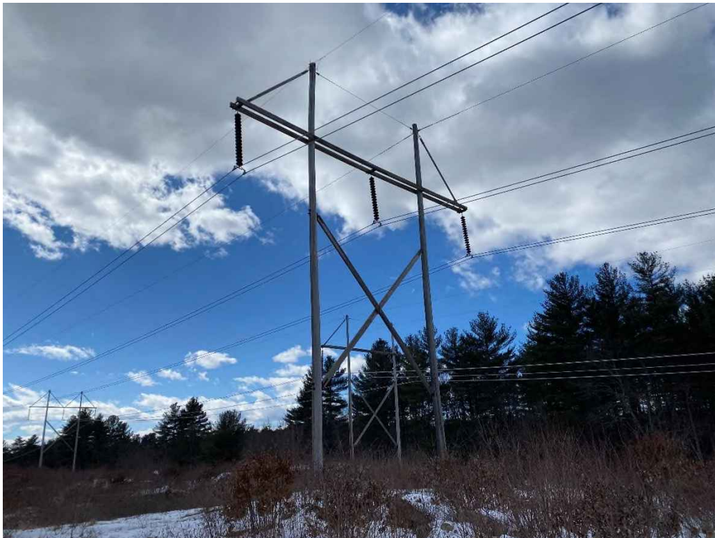
Photograph No. 26: Looking at proposed work pad location adjacent to Structure 49 of the 326 Line.
