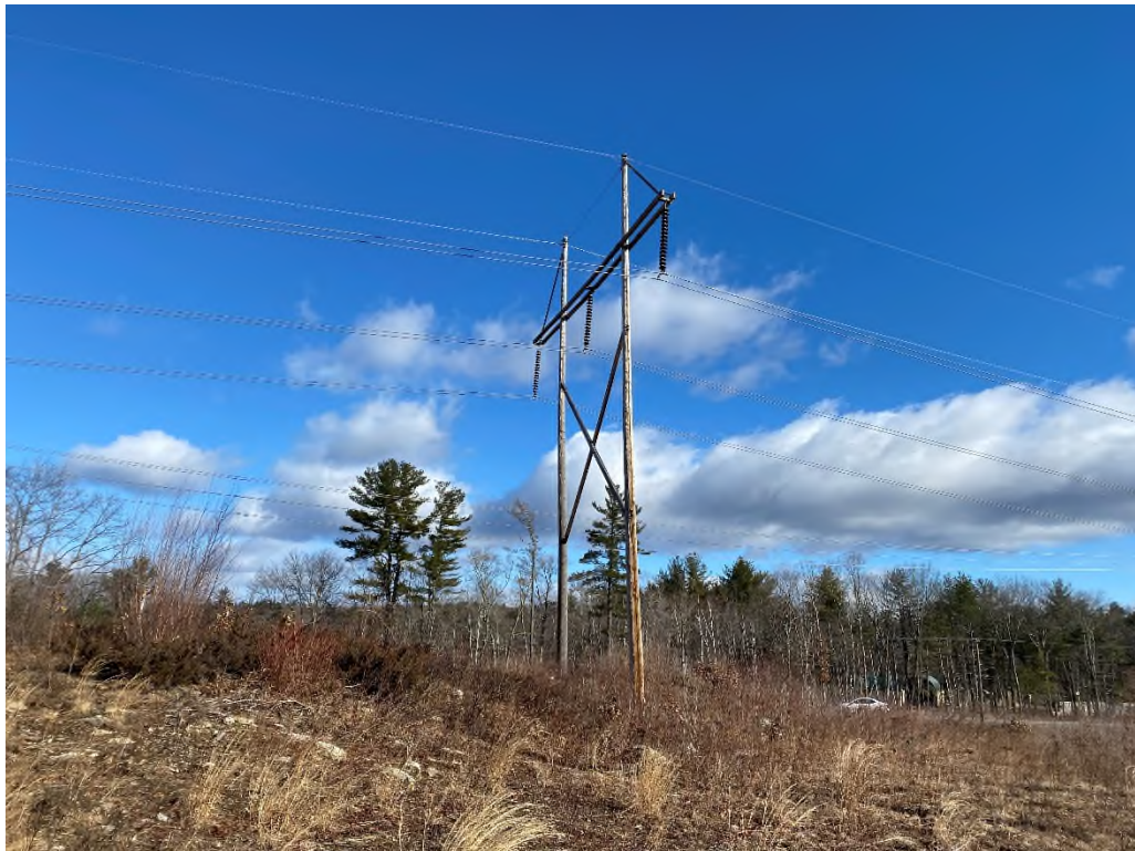
Photograph No. 42: Looking at proposed access and work pad location for Structure 6 of the 326 Line.
