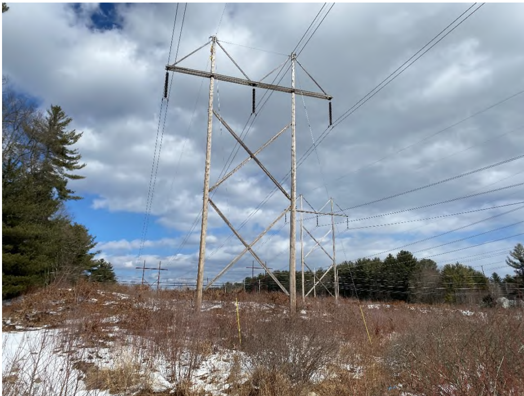
Photograph No. 8: Looking at proposed access and work pad location adjacent to Structure 55 of the 380 Line.
