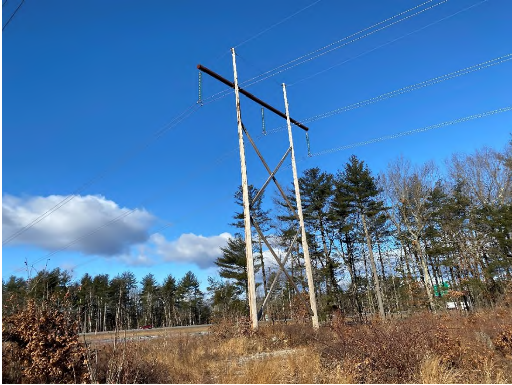
Photograph No. 35: Looking at proposed access and work pad location adjacent to Structure 12 of the 380 Line.
