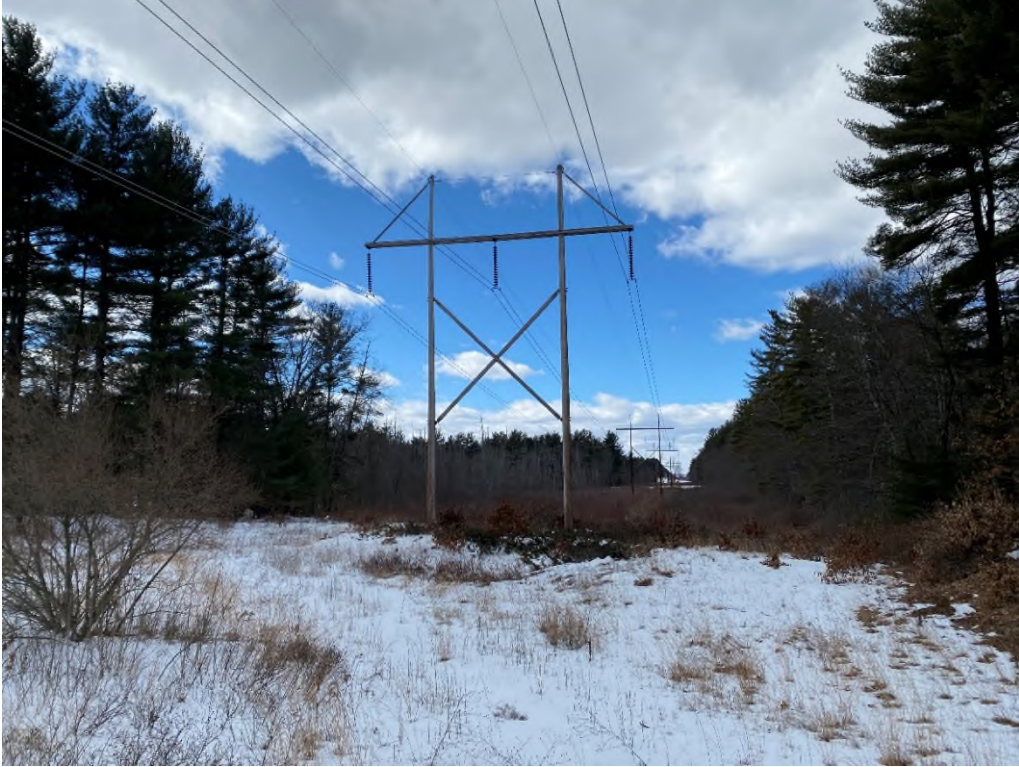
Photograph No. 3: Looking at proposed access and work pad location for Structure 66 of the 380 Line.
