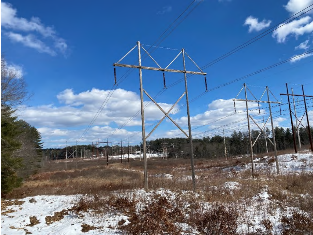
Photograph No. 27: Looking at proposed access and work pad location adjacent to Structure 29 of the 380 Line.
