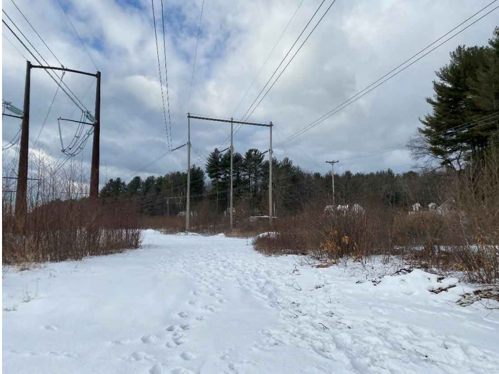
Photograph No. 23: Looking at proposed access and work pad location for Structure 155 of the 326 Line from River Road.
