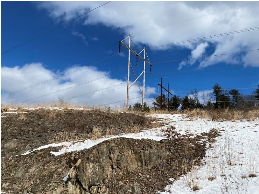
Photograph No. 14: Looking at proposed access adjacent to Structure 72 of the 326 Line.
