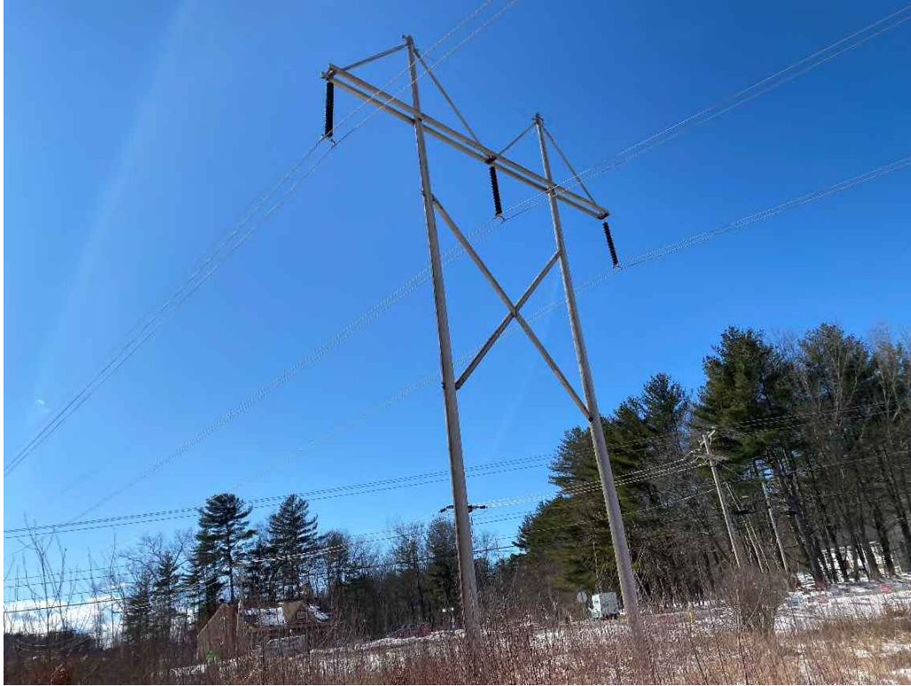
Photograph No. 29: Looking at proposed work pad location adjacent to Structure 25 of the 380 Line.
