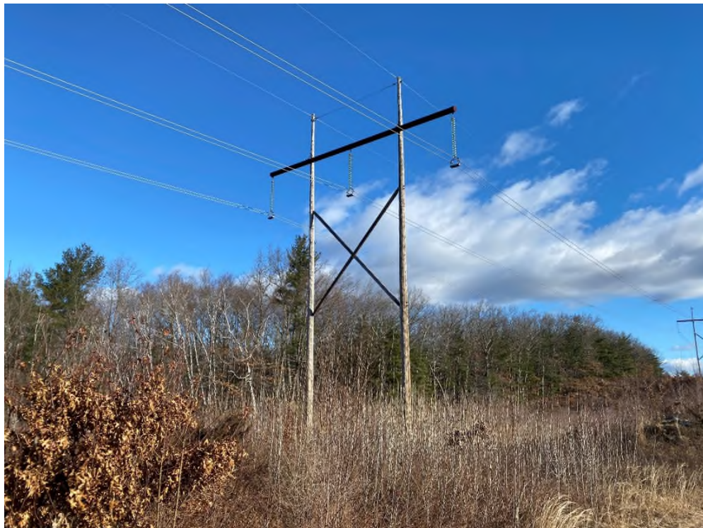
Photograph No. 36: Looking at proposed access and work pad location adjacent to Structure 11 of the 380 Line.
