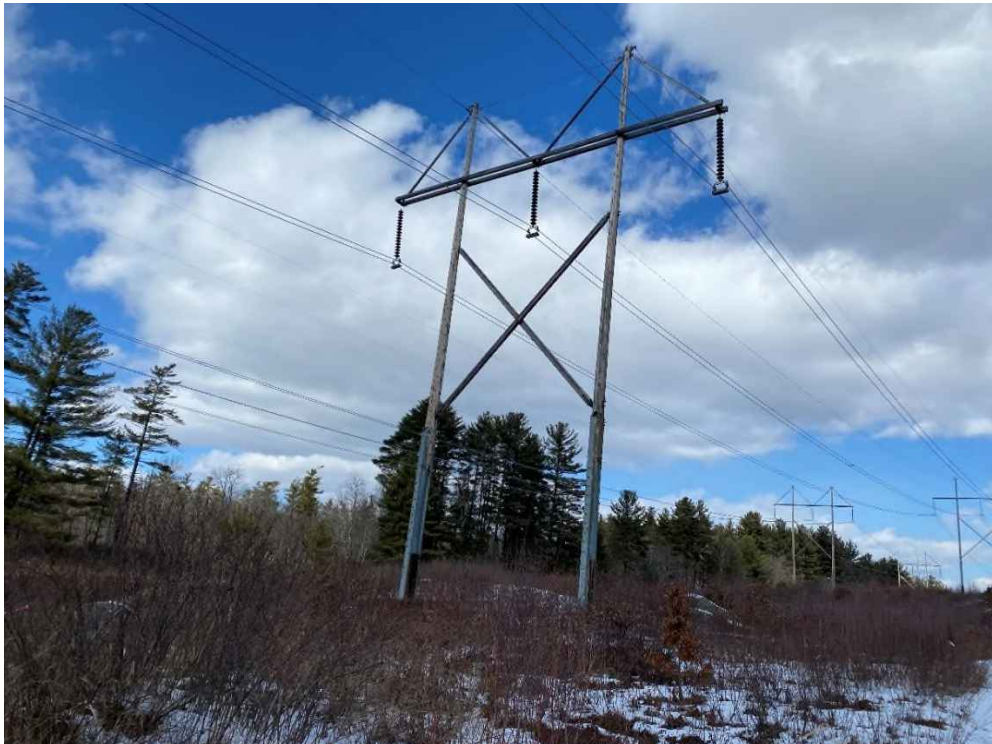
Photograph No. 24: Looking at proposed access and work pad location adjacent to Structure 51 of the 326 Line.
