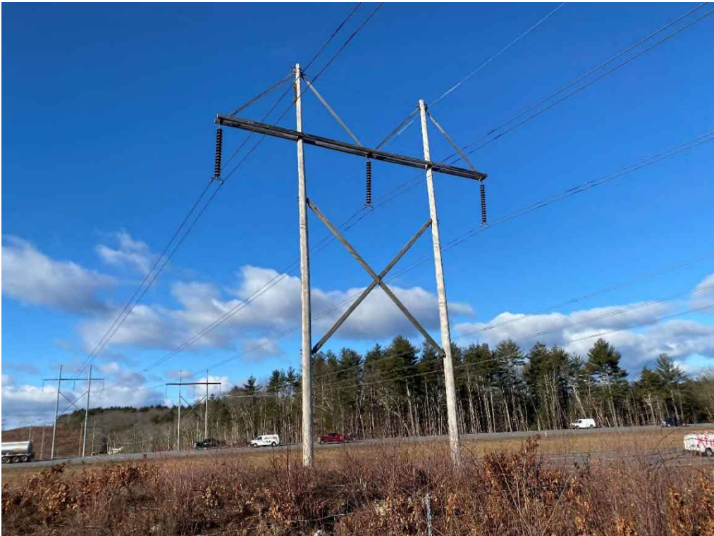
Photograph No. 34: Looking at proposed access and work pad location adjacent to Structure 13 of the 326 Line.
