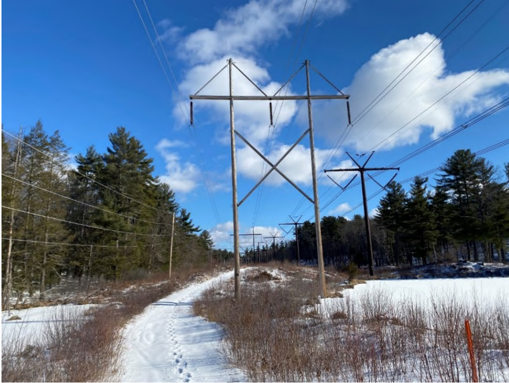
Photograph No. 19: Looking at proposed access and work pad location for Structure 123 of the 326 Line.
