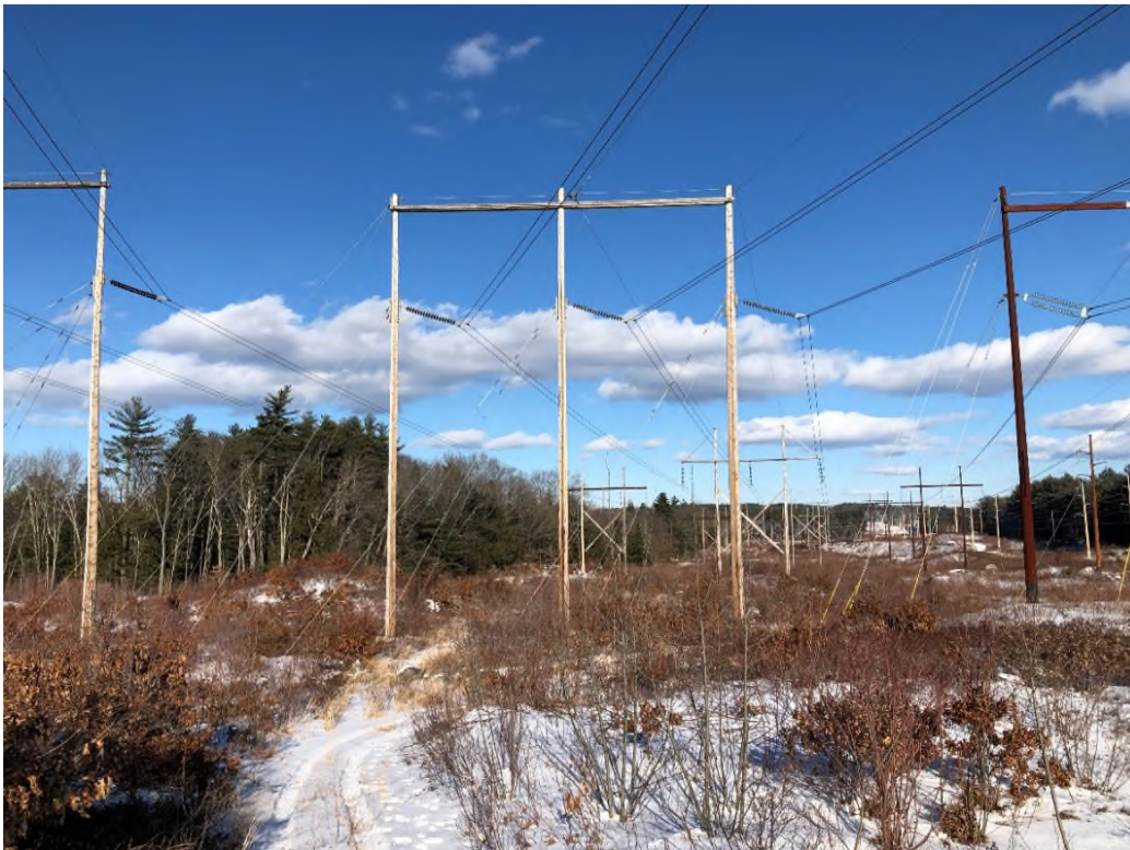
Photograph No. 38: Looking at proposed access and work pad location adjacent to Structure 10 of the 326 Line.
