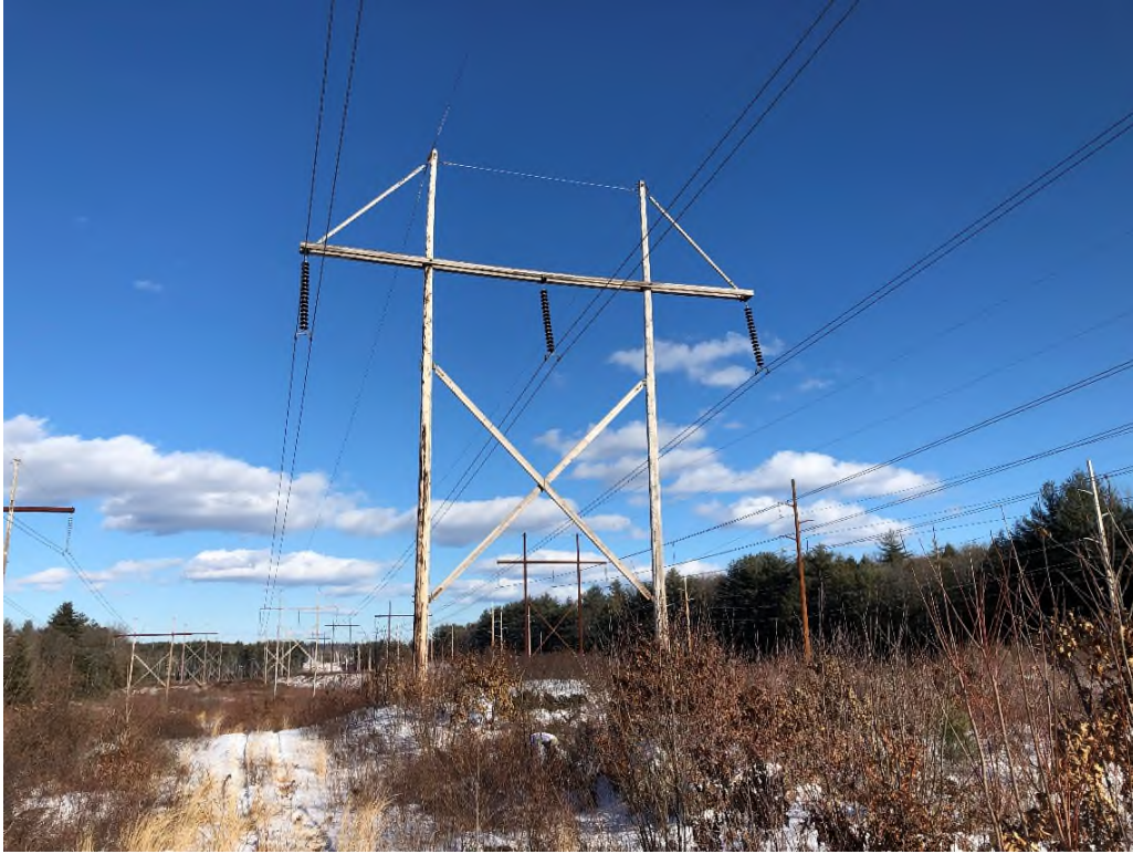
Photograph No. 39: Looking at proposed access and work pad location for Structure 9 of the 326 Line.
