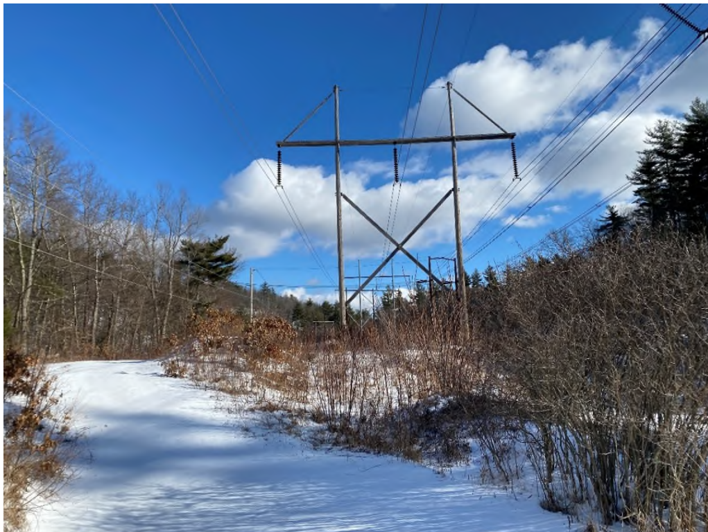
Photograph No. 18: Looking at proposed work pad location for Structure 121 of the 326 Line.
