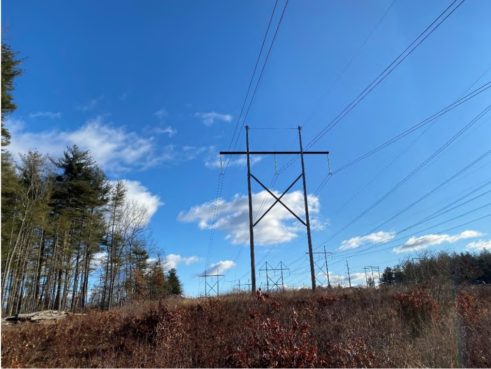
Photograph No. 33: Looking at proposed access and work pad location to Structure 13 of the 380 Line.
