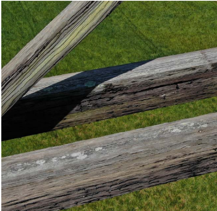
Cross Arm Damage – Line 3754
