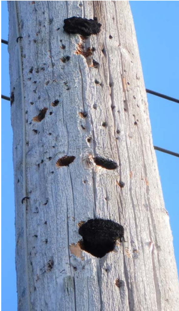
Woodpecker Damage – Line 387
