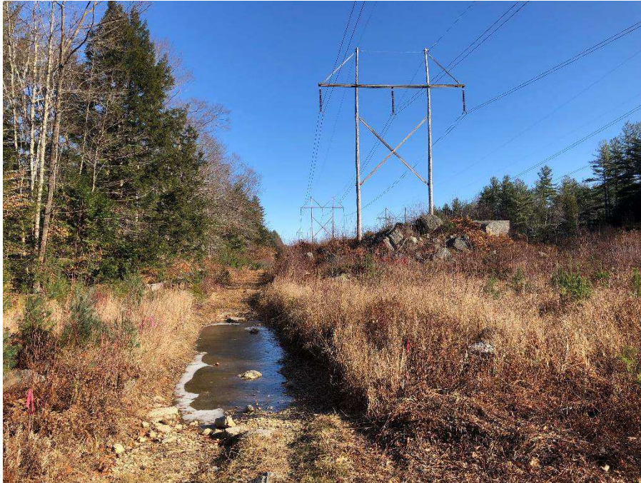
Photograph No. 7: Looking northwesterly at proposed structure replacement 385 structure 157 with proposed access route in Deerfield.
