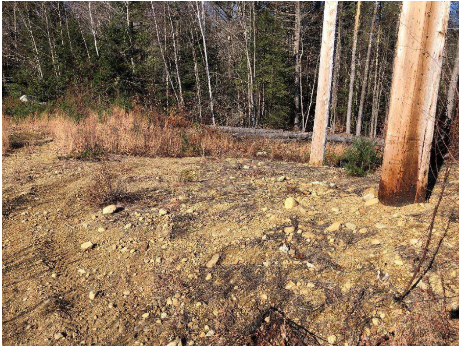
Photograph No. 19: Looking northwesterly at proposed structure replacement 385 structure 154 work pad in Deerfield.
