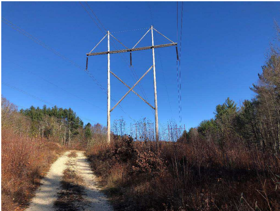
Photograph No. 34: Looking northeasterly at proposed existing access route towards 391 structure 150 in Northwood.
