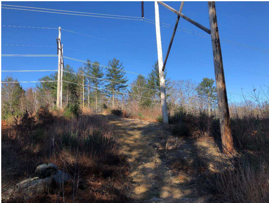
Photograph No. 18: Looking northwesterly at proposed structure replacement 385 structure 154 (left) and 391 structure 158 (right) with proposed access in-between the two structures in Deerfield.
