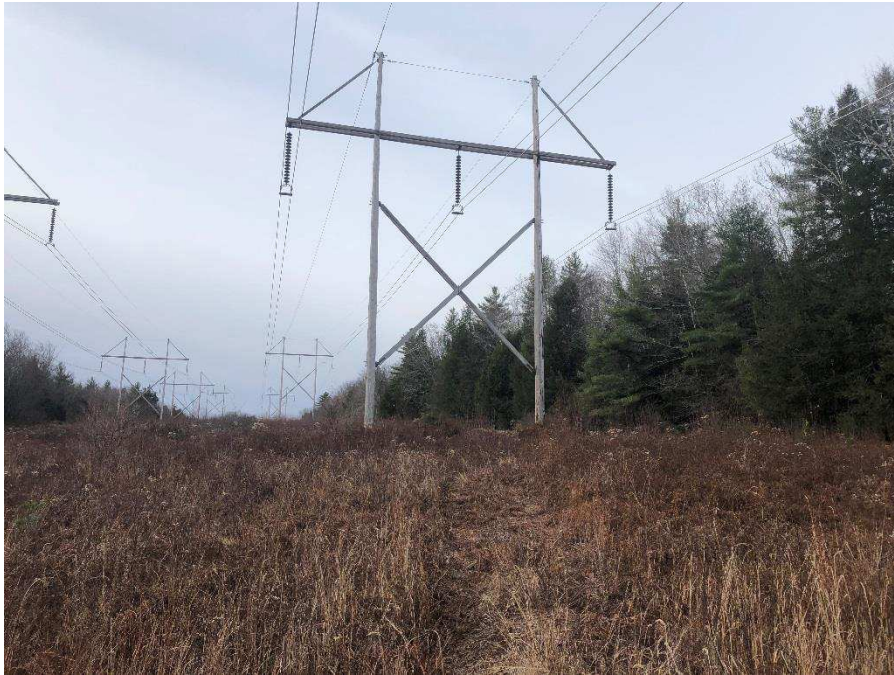
Photograph No. 51: Looking northeasterly at proposed work pad location adjacent to 385 Line Structure 90 Strafford.
