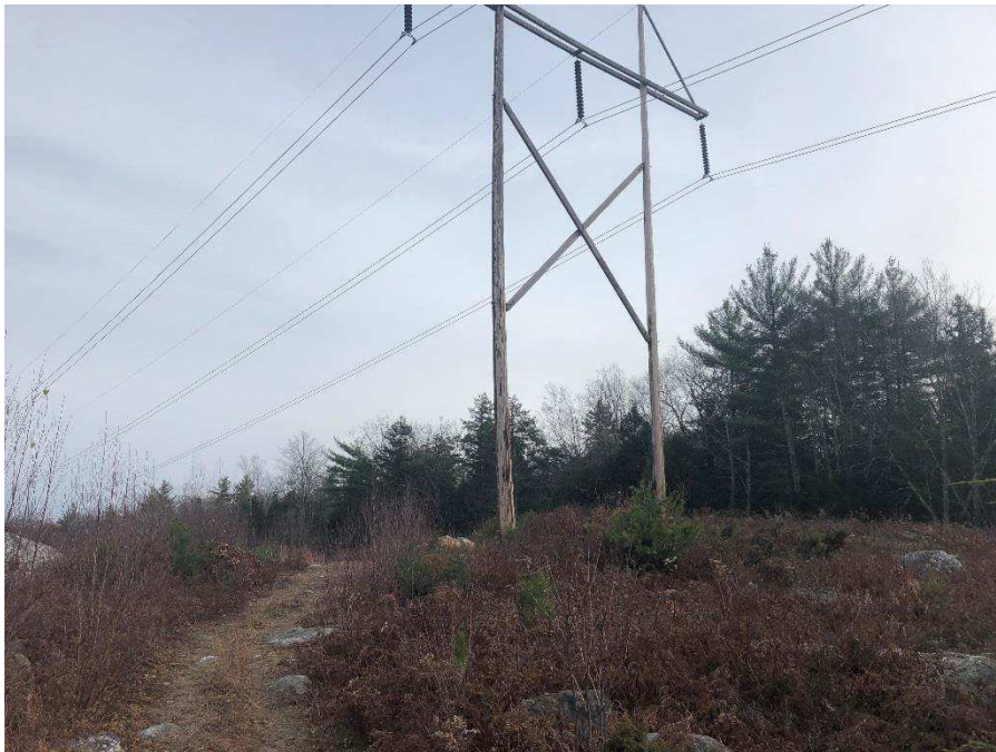
Photograph No. 46: Looking easterly at proposed work pad location adjacent to 391 Line Structure 97 Strafford.
