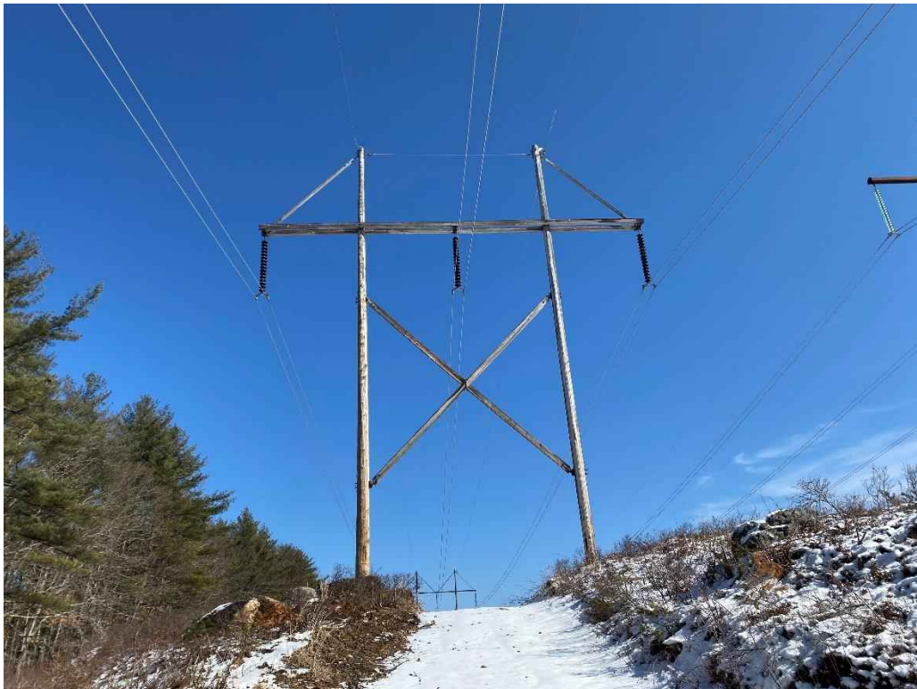
Photograph No. 44: View of proposed access and work pad location for 385 Line Structure 78.
