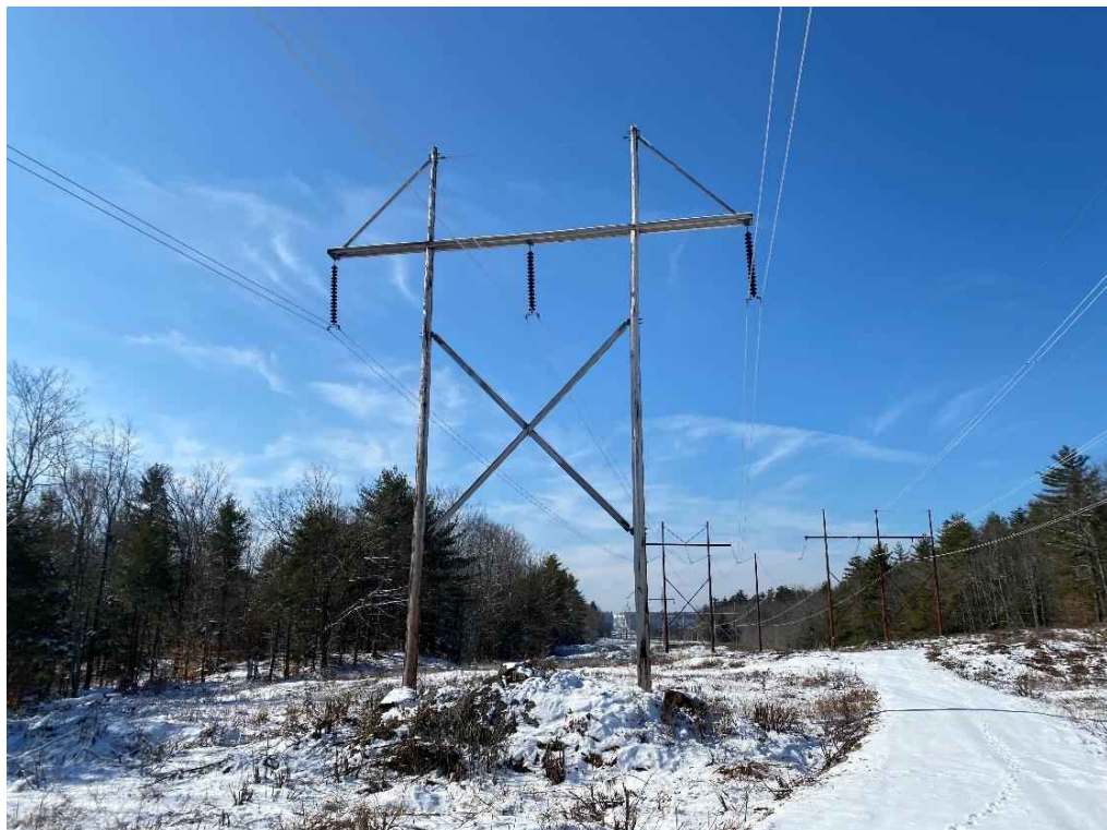
Photograph No. 54: View of proposed access and work pad location for 391 Line Structure 73.
