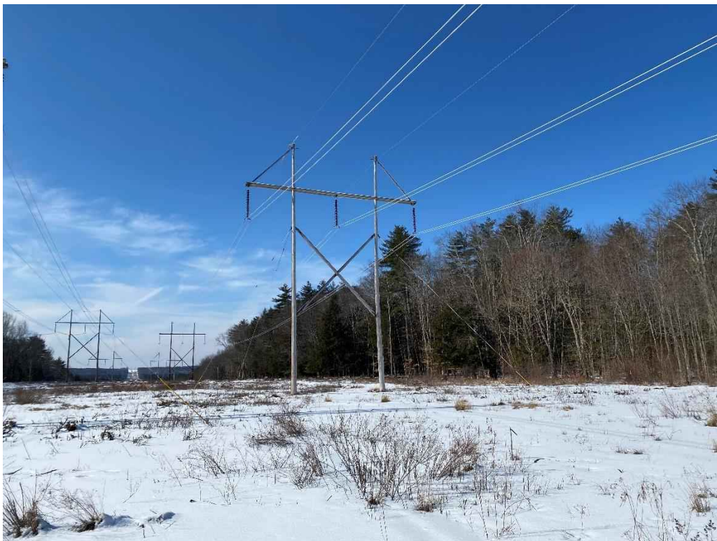
Photograph No. 50: View of proposed access and work pad location adjacent for 385 Line Structure 69.
