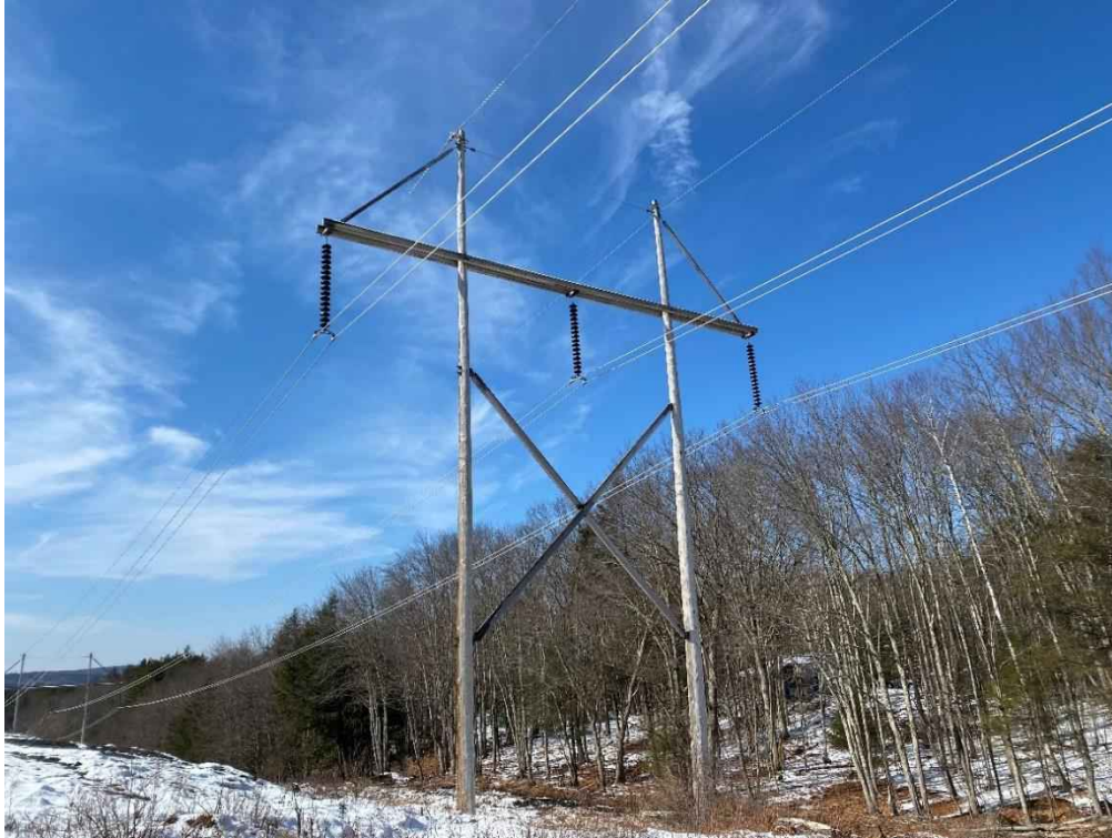
Photograph No. 47: View of proposed access and work pad location for 391 Line Structure 71.
