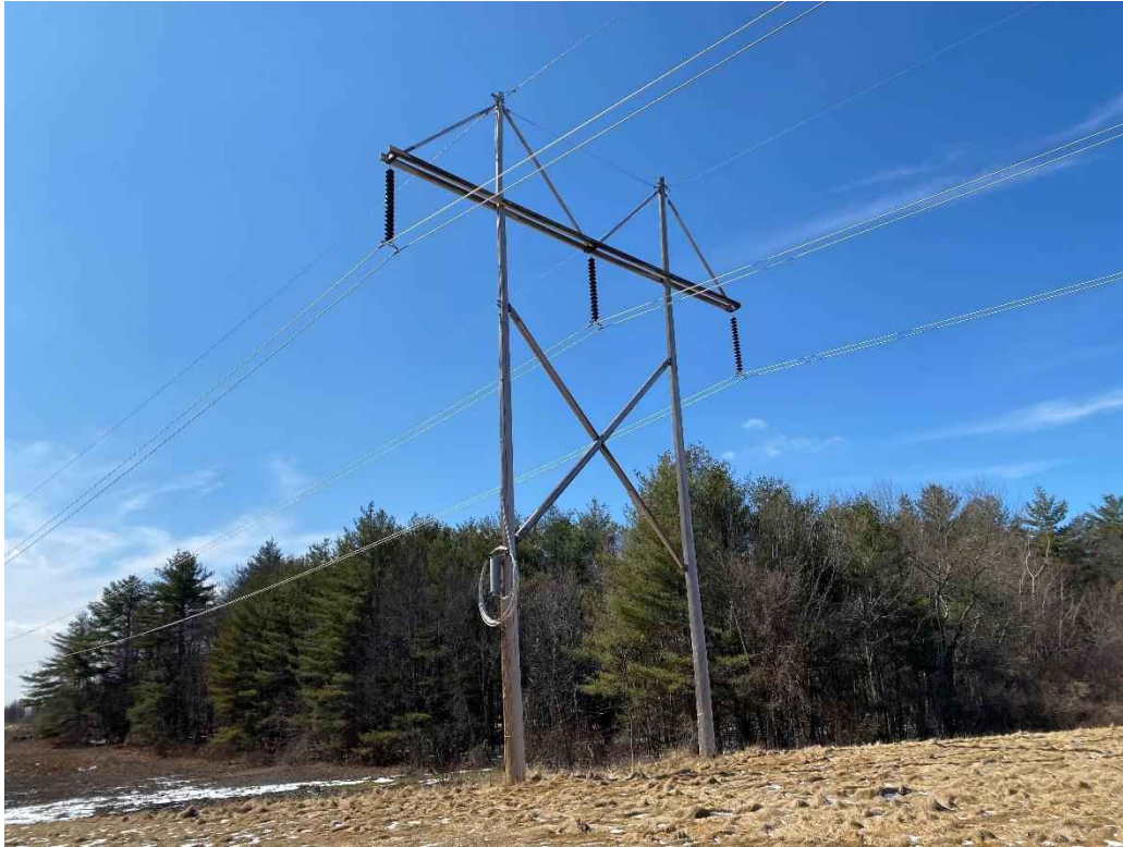
Photograph No. 31: View of proposed access and work pad location adjacent to 385 Line Structure 144.
