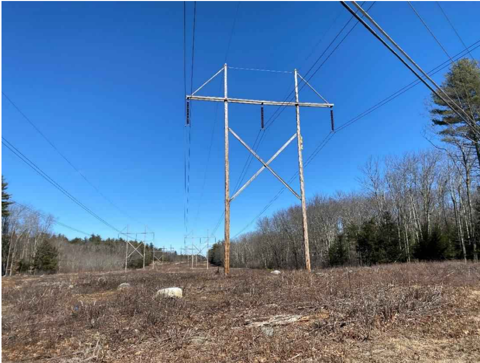
Photograph No. 49: View of proposed access and work pad location for 391 Line Structure 77.
