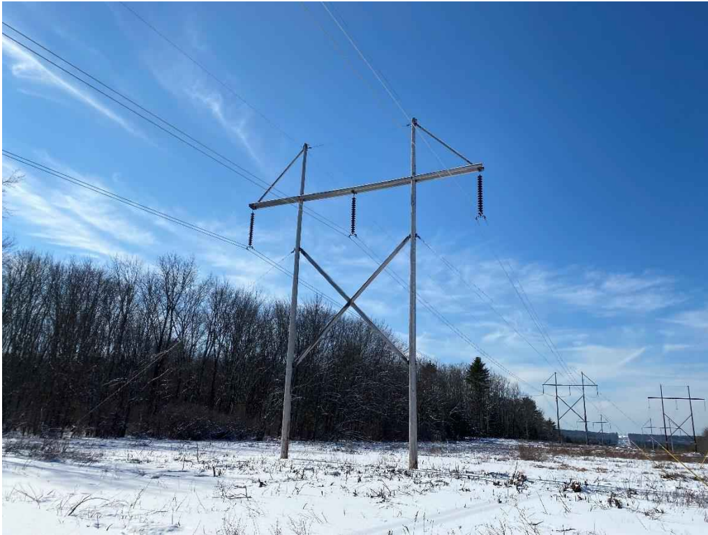
Photograph No. 51: View of proposed access and work pad location for 391 Line Structure 76.
