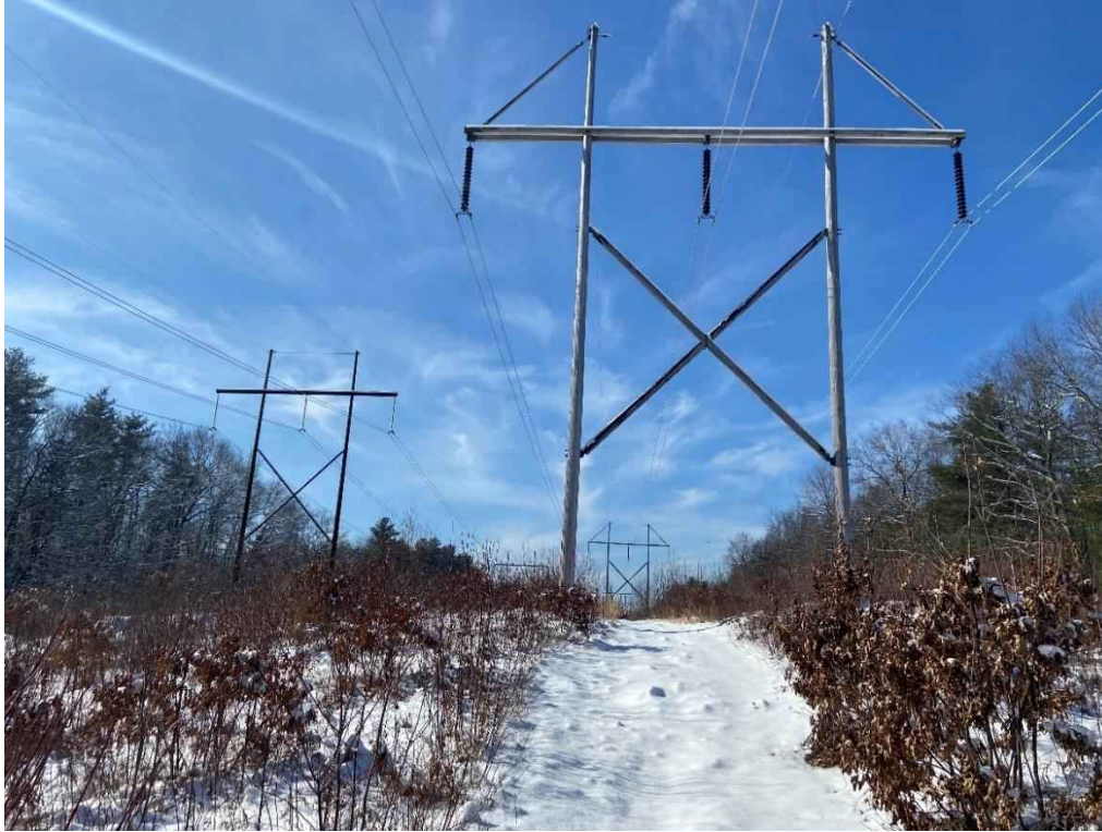
Photograph No. 5: View of proposed access and work pad location for 373 Line Structure 317.
