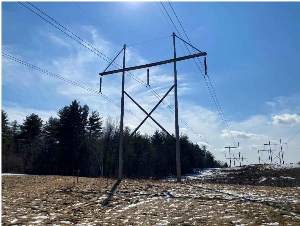
Photograph No. 30: View of proposed access and work pad location for 373 Line Structure 147.
