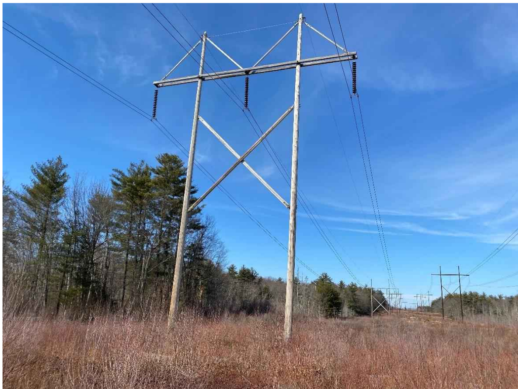
Photograph No. 20: View of proposed access and work pad location for 373 Line Structure 256.
