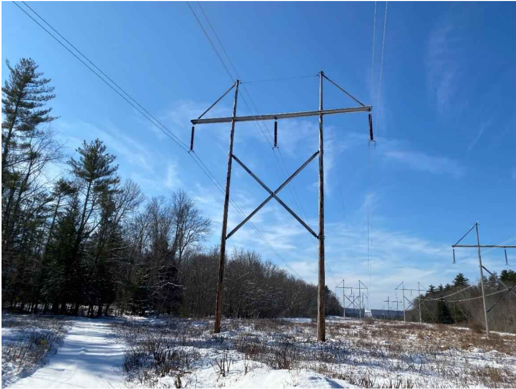
Photograph No. 53: View of proposed access and work pad location for 391 Line Structure 75.
