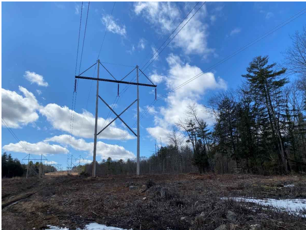
Photograph No. 64: View of proposed access and work pad location for 385 Line Structure 24.
