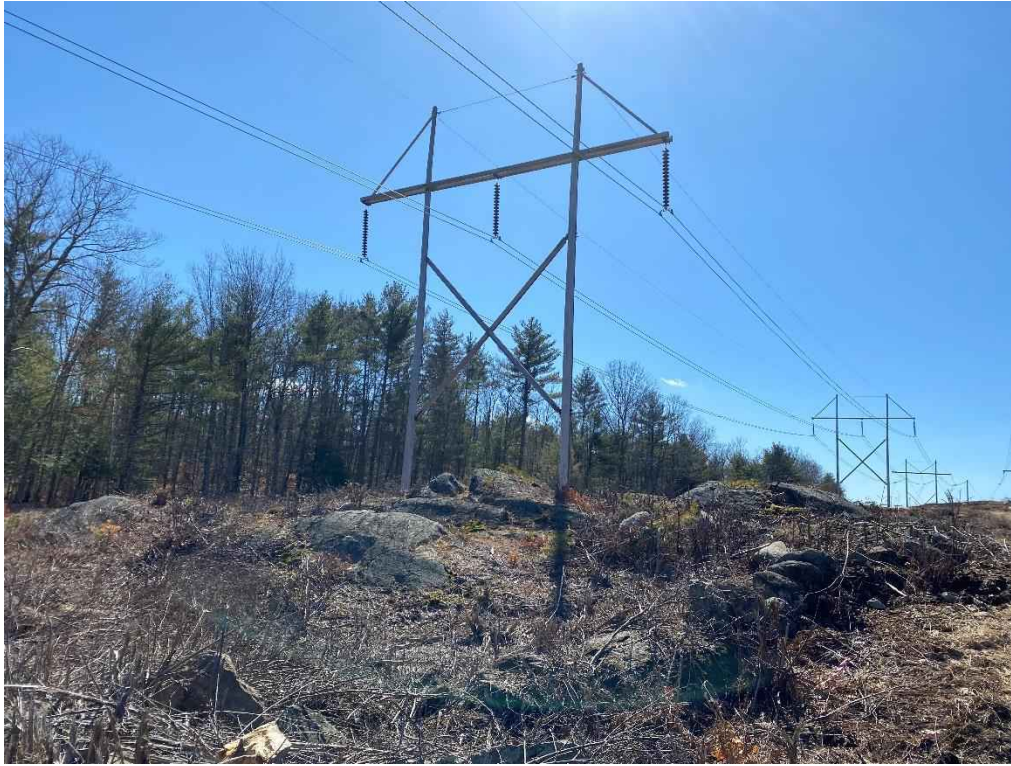
Photograph No. 55: View of proposed access and work pad location for 391 Line Structure 72.
