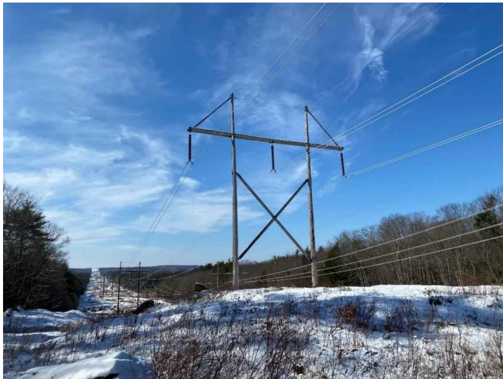
Photograph No. 46: View of proposed access and work pad location for 385 Line Structure 72.
