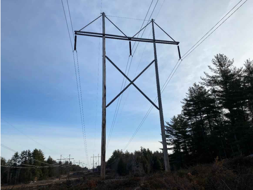
Photograph No. 29: View of proposed access and work pad location for 391 Line Structure 163.
