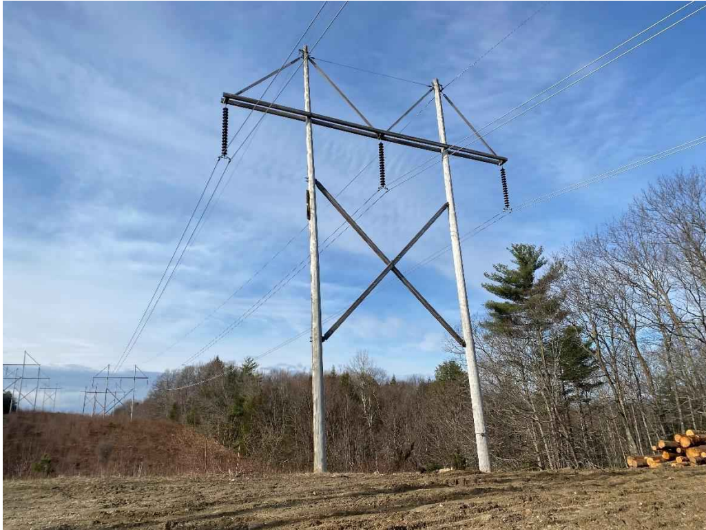
Photograph No. 27: View of proposed access and work pad location adjacent to 373 Line Structure 186.
