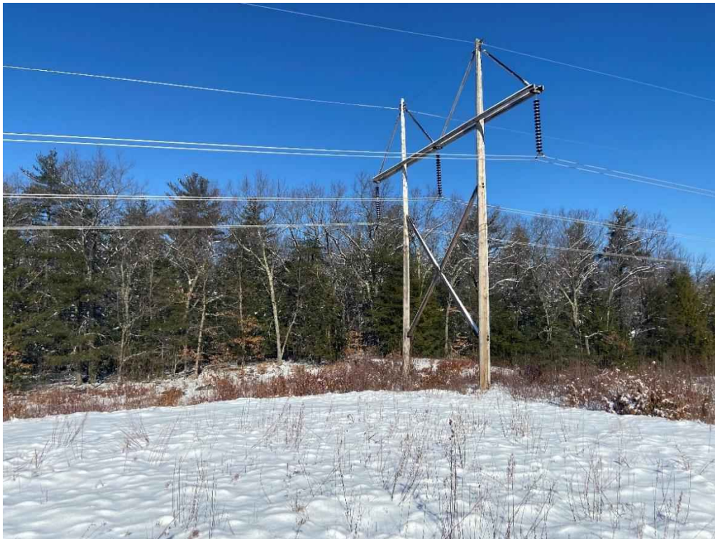
Photograph No. 6: View of proposed access and work pad location adjacent to 373 Line Structure 316.
