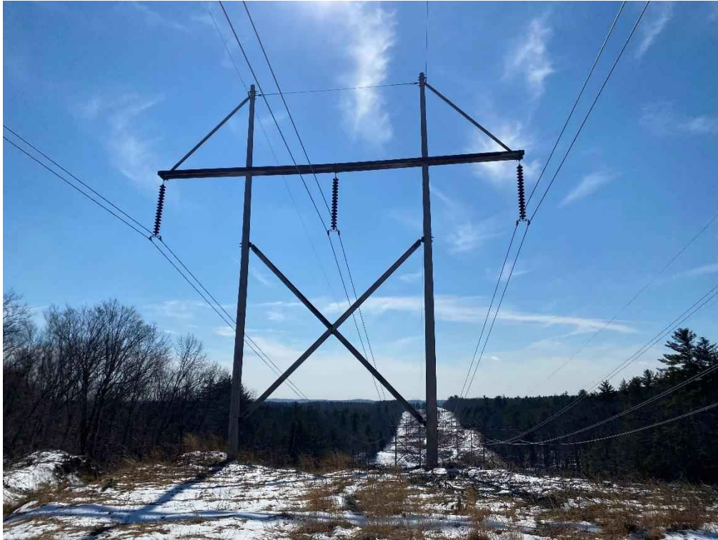
Photograph No. 39: View of proposed access and work pad location for 391 Line Structure 130.
