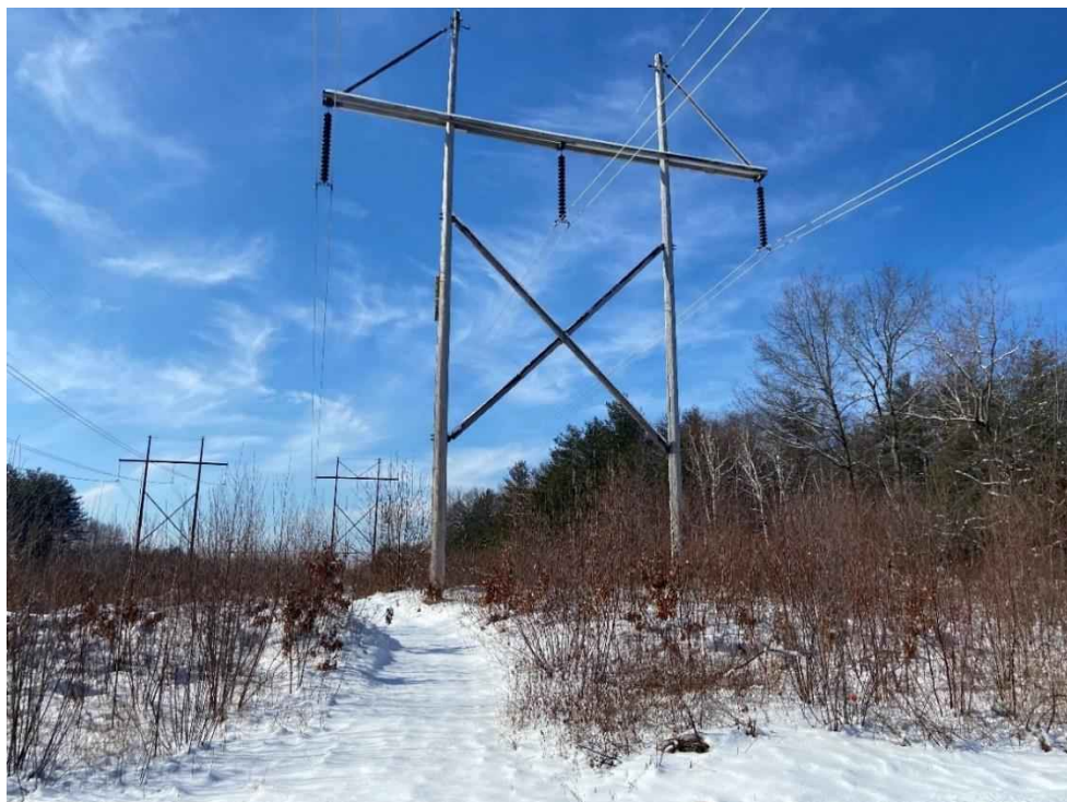
Photograph No. 2: View of proposed access and work pad location for 373 Line Structure 320.
