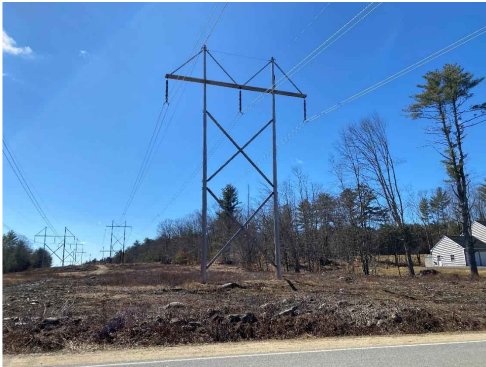
Photograph No. 56: View of proposed access and work pad location to 385 Line Structure 65 from Second Crown Point Road.
