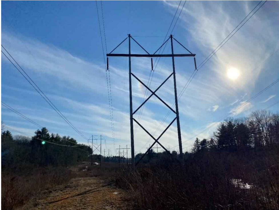
Photograph No. 1: View of proposed access and work pad location from Route 28 to 391 Line Line, Structure 326.
