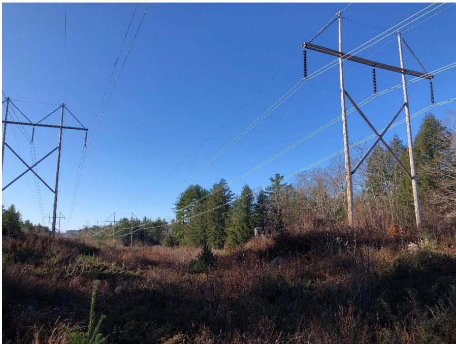
Photograph No. 8: Looking southwesteryly at proposed structure replacement 385 structure 157 on right in Deerfield.
