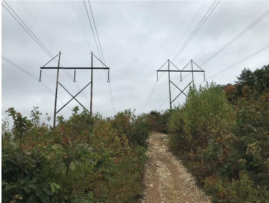
Photograph No. 3: Looking northerly at proposed access route toward 391 Structure 278 in Chester.
