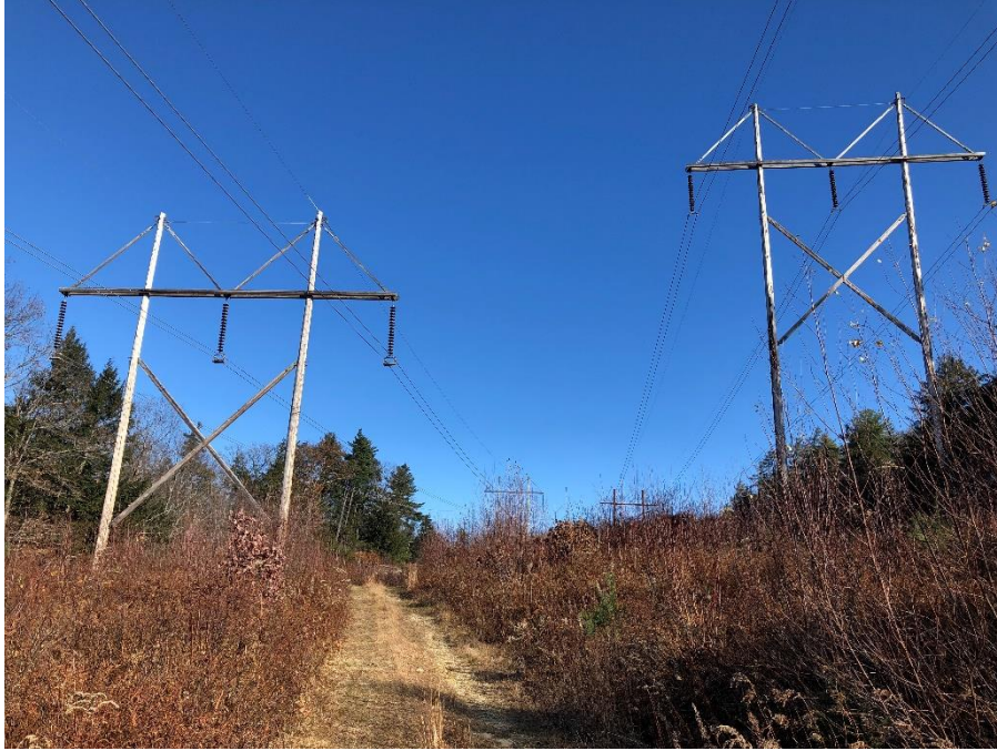
Photograph No. 27: Looking northeasterly at proposed structure replacement 385 structure 151 (left) and 391 structure 155 (right) with proposed access route between structures in Deerfield.
