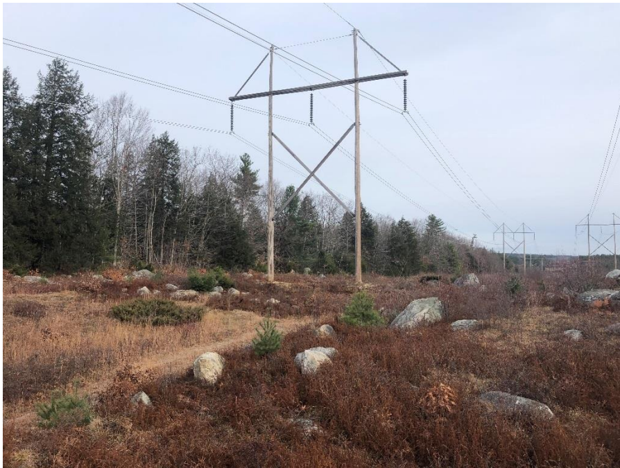
Photograph No. 44: Looking northeasterly at proposed work pad location adjacent to 385 Line Structure 93 Strafford.
