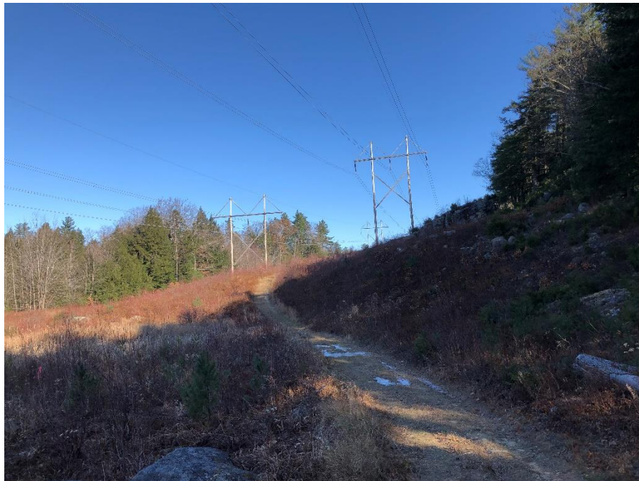
Photograph No. 26: Looking northerly at proposed access route between structures 156 & 155 on the 391 line in Deerfield.
