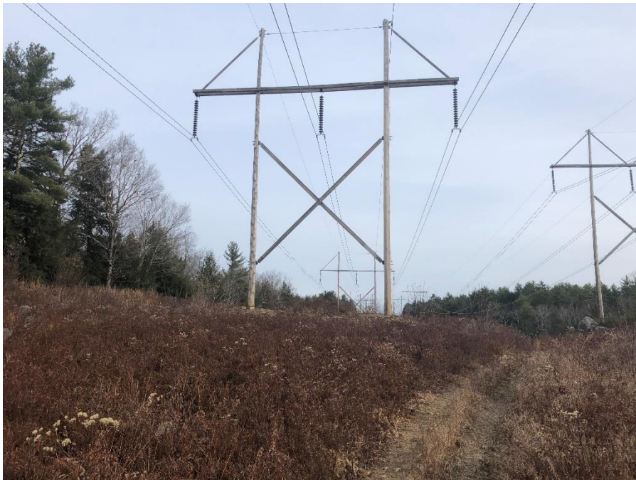
Photograph No. 54: Looking northeasterly at proposed work pad location adjacent to 385 Line Structure 89 Strafford.
