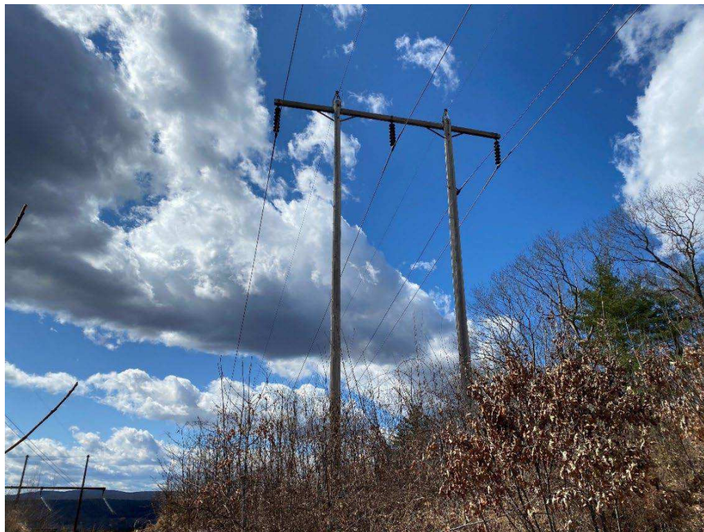
Photograph No. 12: Looking at proposed access and work pad location adjacent to N186 Structure 245.
