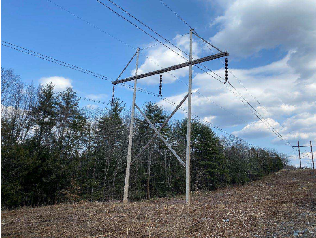
Photograph No. 17: Looking at proposed access and work pad location adjacent to 379 Structure 546.
