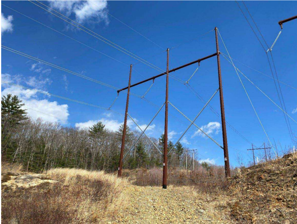
Photograph No. 11: Looking at proposed access and work pad location for 379 Structure 581.
