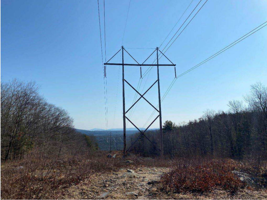
Photograph No. 31: Looking at proposed access and work pad location for 379 Structure 454.
