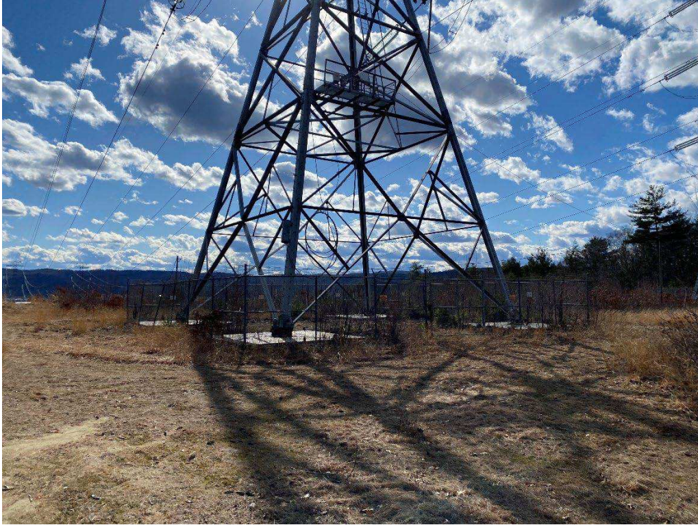
Photograph No. 1: Looking at proposed access and work pad location for N186 Structure 261.
