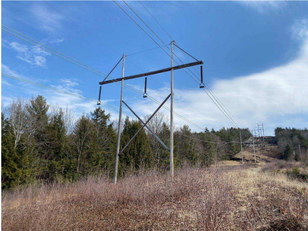
Photograph No. 27: Looking at proposed access and work pad location for 379 Structure 478.
