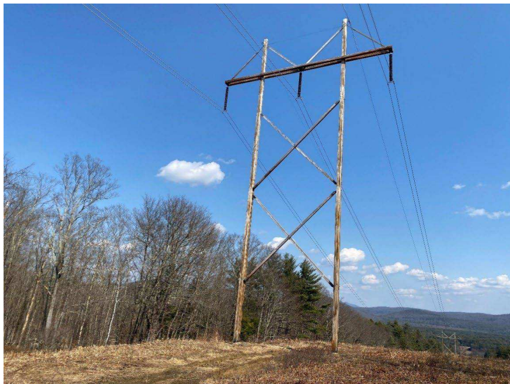
Photograph No. 20: Looking at proposed access and work pad location for 379 Structure 541.
