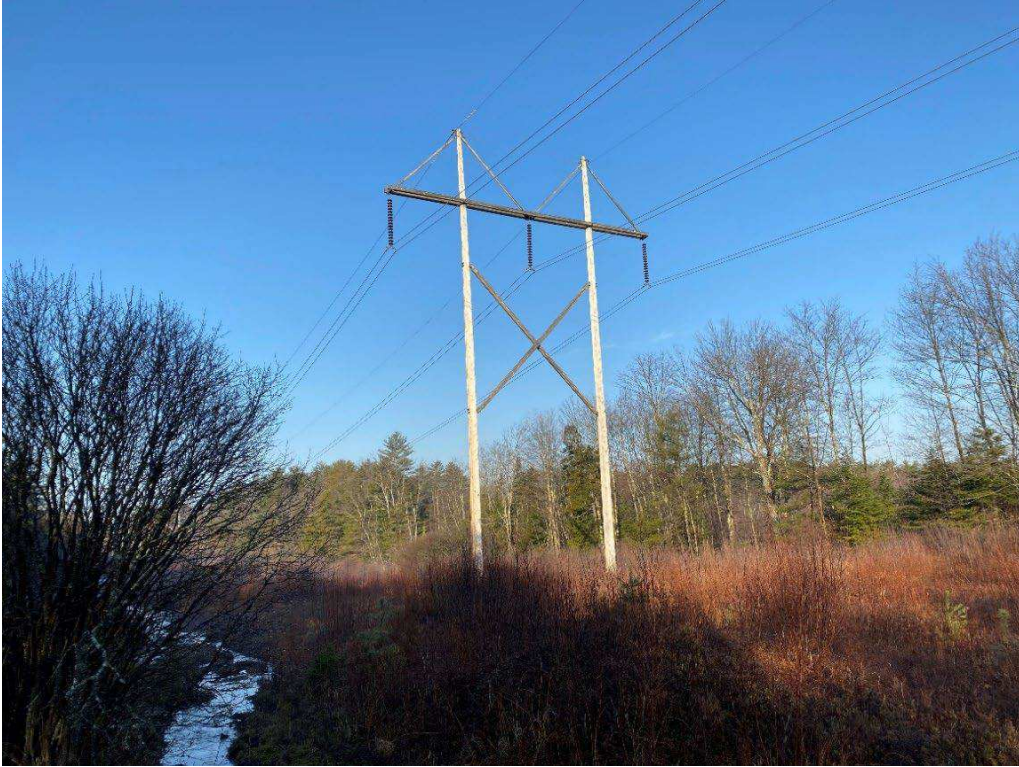
Photograph No. 37: Looking at proposed access and work pad location for 379 Structure 437.
