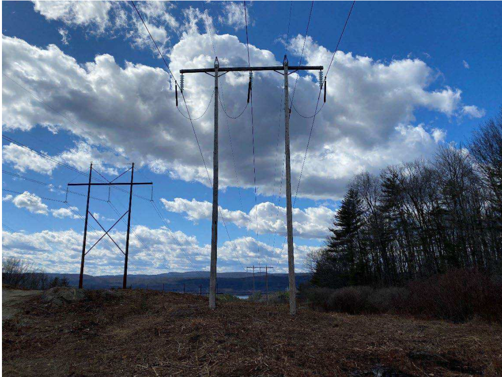
Photograph No. 13: Looking at proposed access and work pad location for N186 Structure 244.
