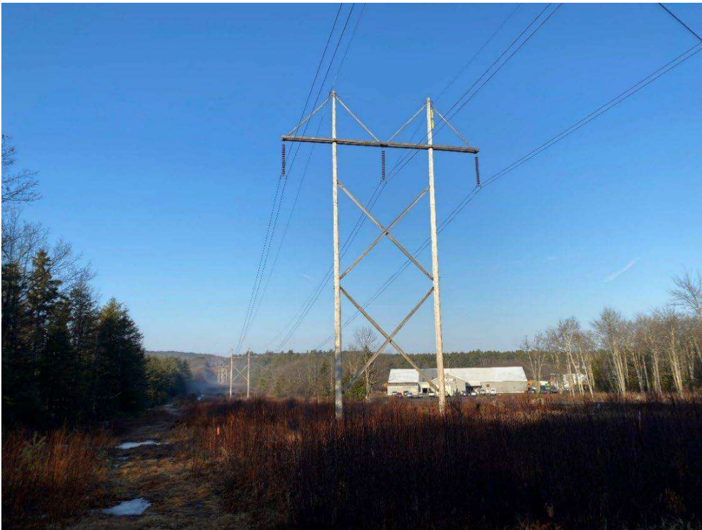
Photograph No. 38: Looking at proposed work pad location adjacent to 379 Structure 436 from NH Route 12 North.
