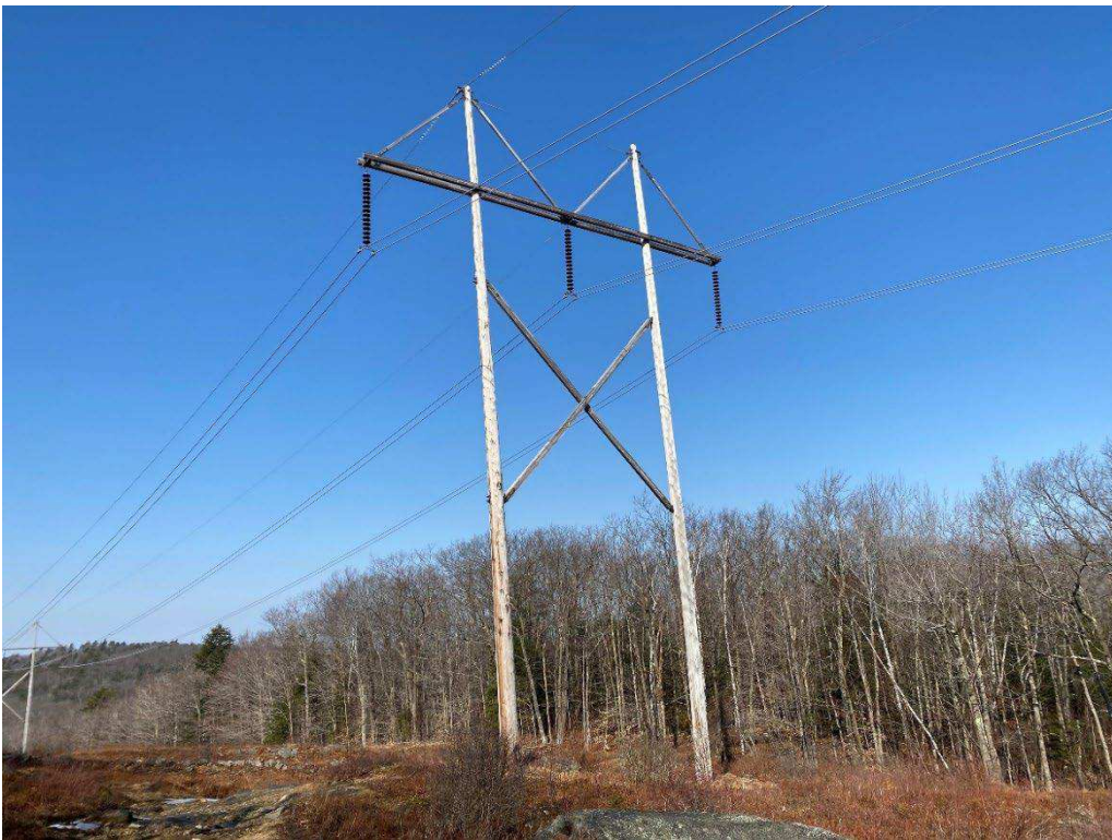
Photograph No. 30: Looking at proposed access and work pad location for 379 Structure 455.
