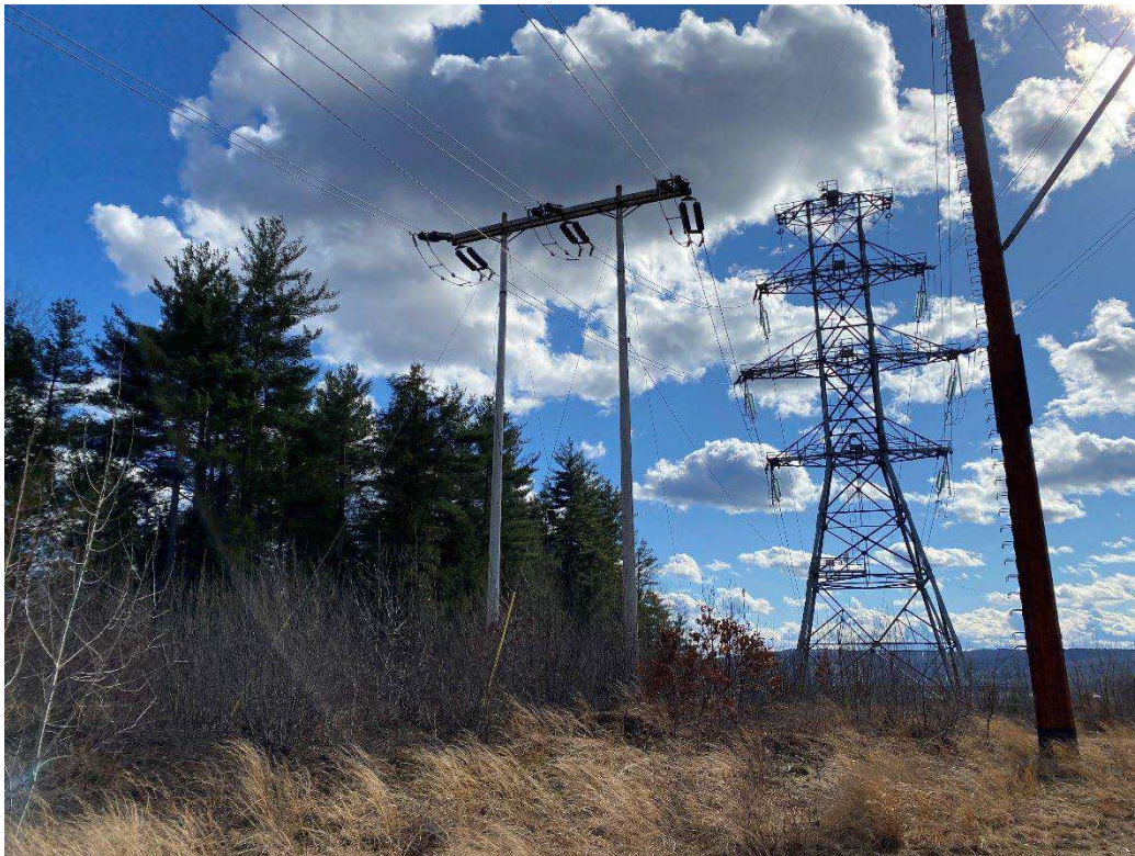
Photograph No. 2: Looking at proposed access and work pad location for N186 Structure 260.
