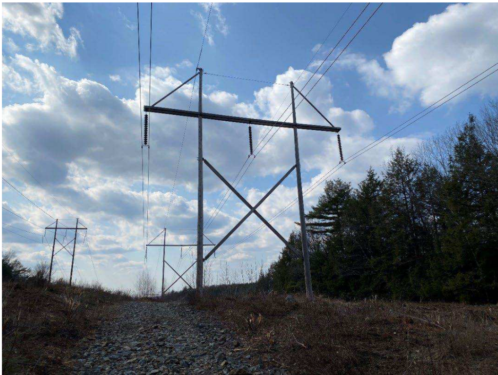
Photograph No. 16: Looking at proposed access and work pad location for 379 Structure 547.
