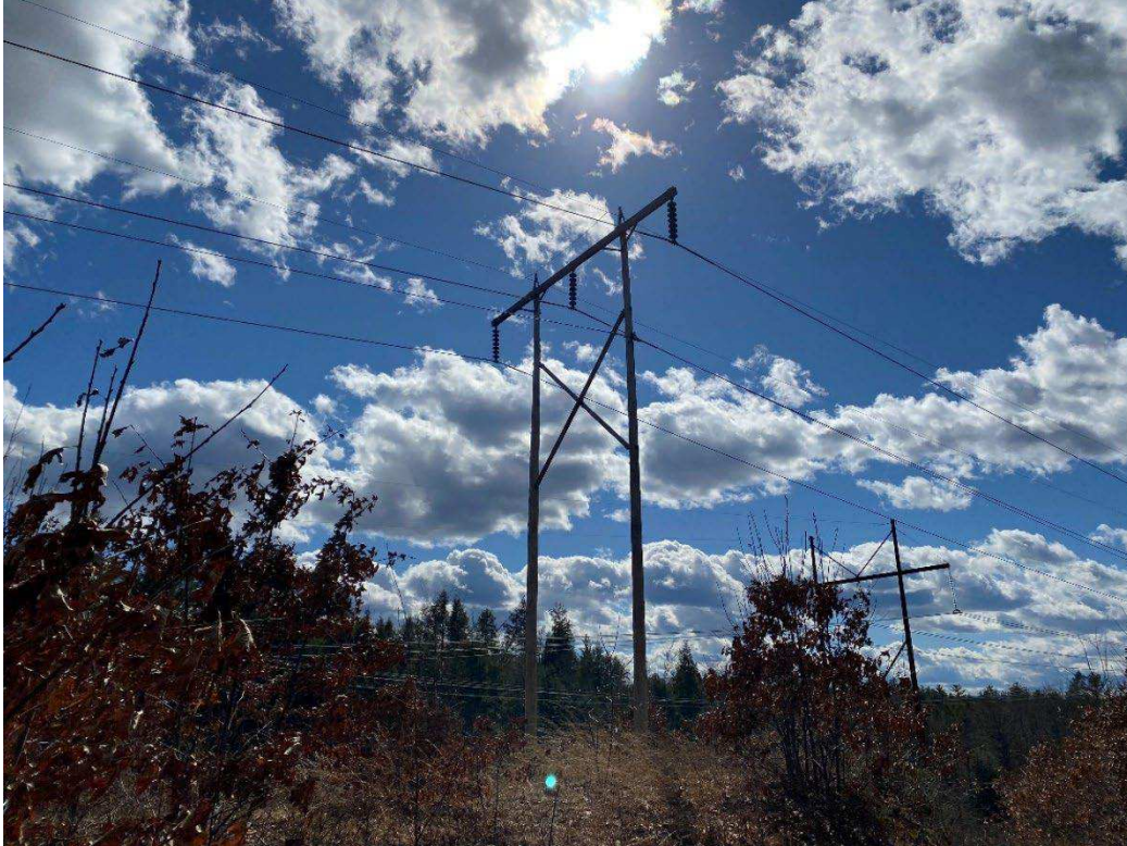
Photograph No. 7: Looking at proposed access and work pad location adjacent to N186 Structure 249.
