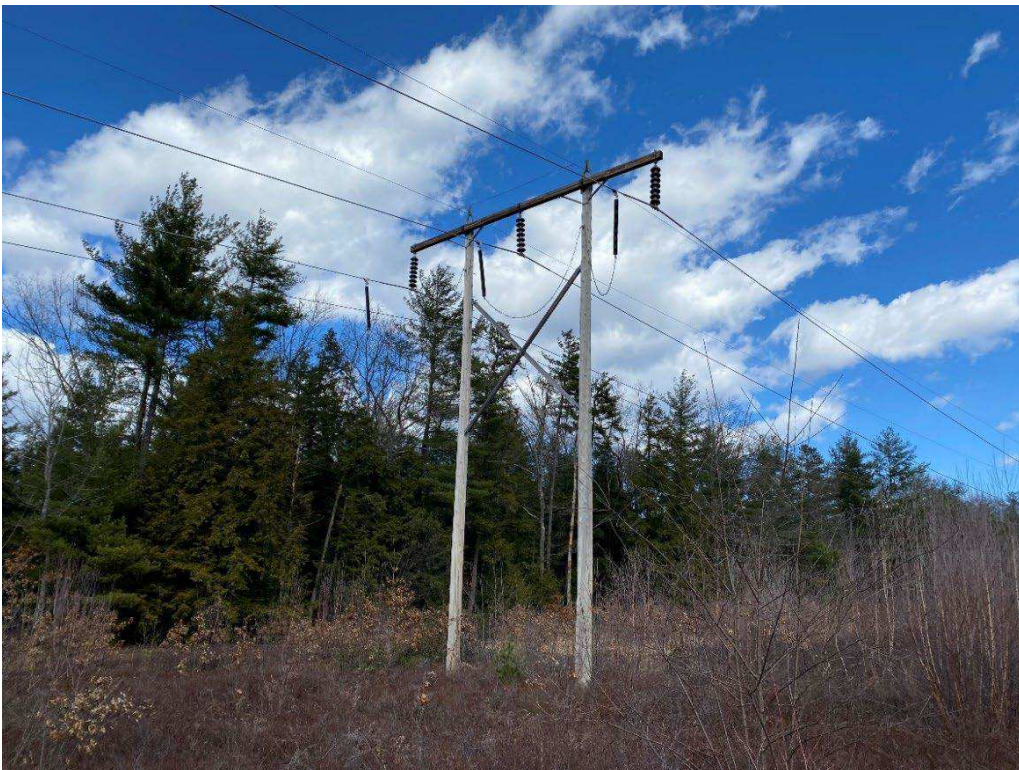
Photograph No. 6: Looking at proposed work pad location adjacent to N186 Structure 254.
