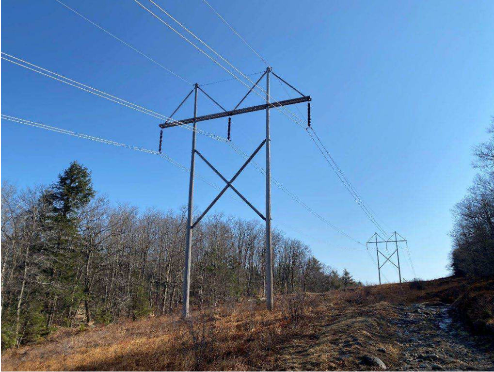
Photograph No. 29: Looking at proposed access and work pad location for 379 Structure 456.
