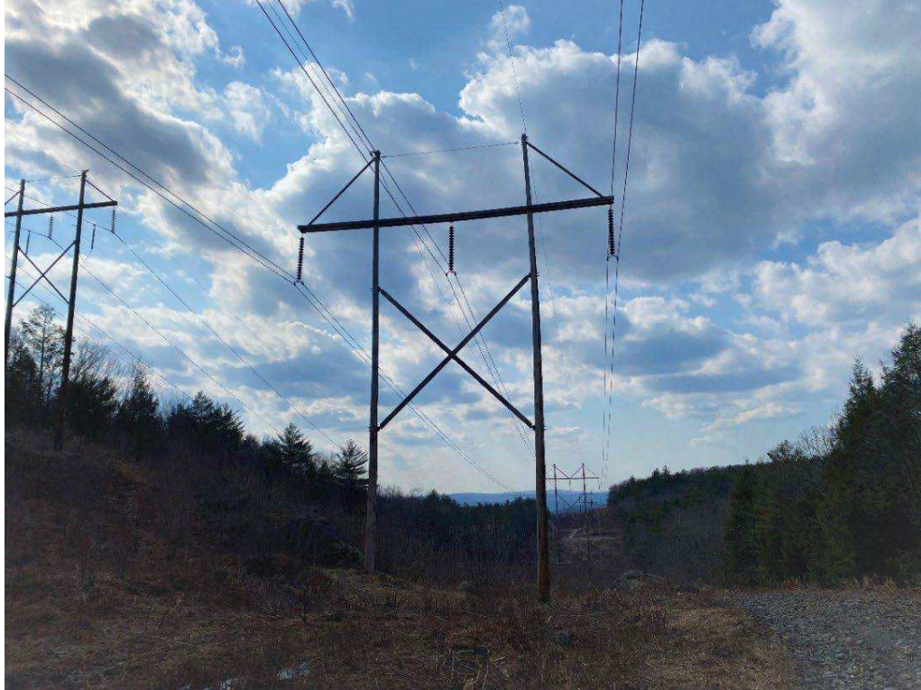
Photograph No. 15: Looking at proposed access and work pad location for 379 Structure 548.
