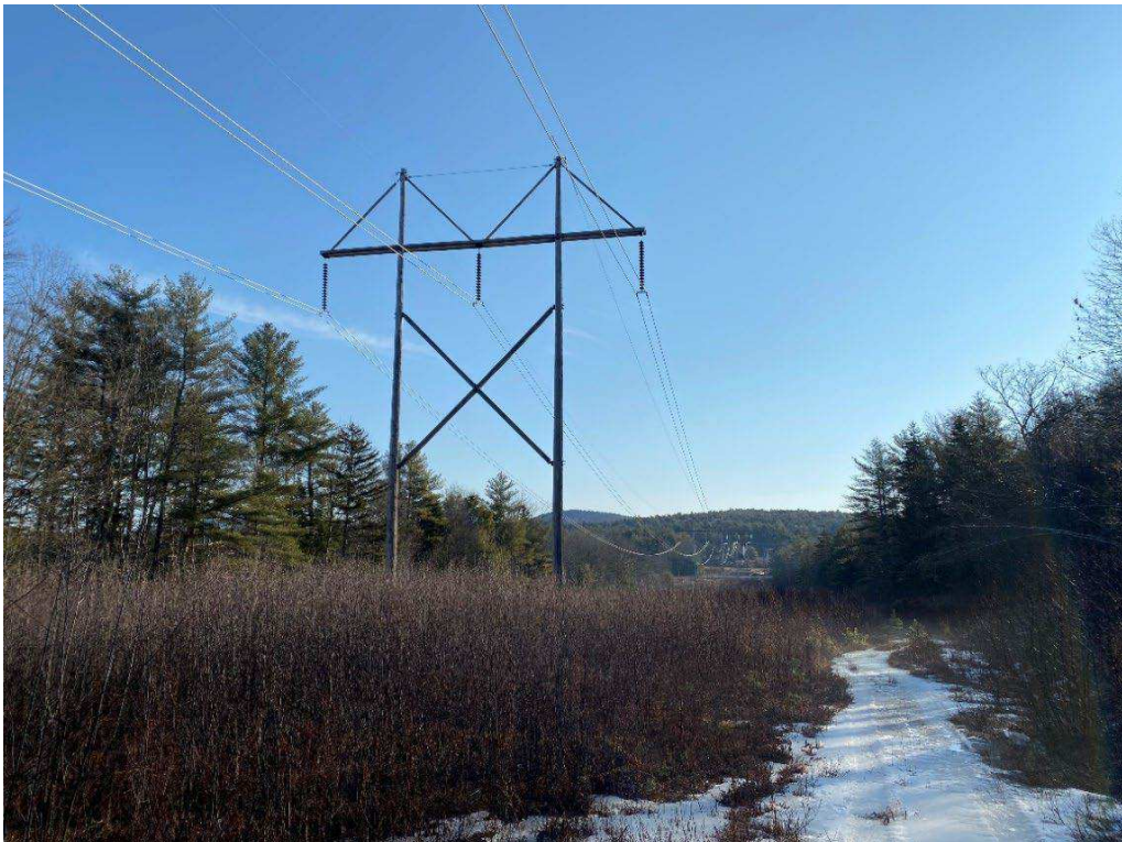
Photograph No. 36: Looking at proposed access and work pad location adjacent to 379 Structure 438.
