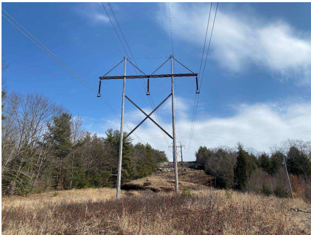
Photograph No. 28: Looking at proposed access and work pad location for 379 Structure 477.
