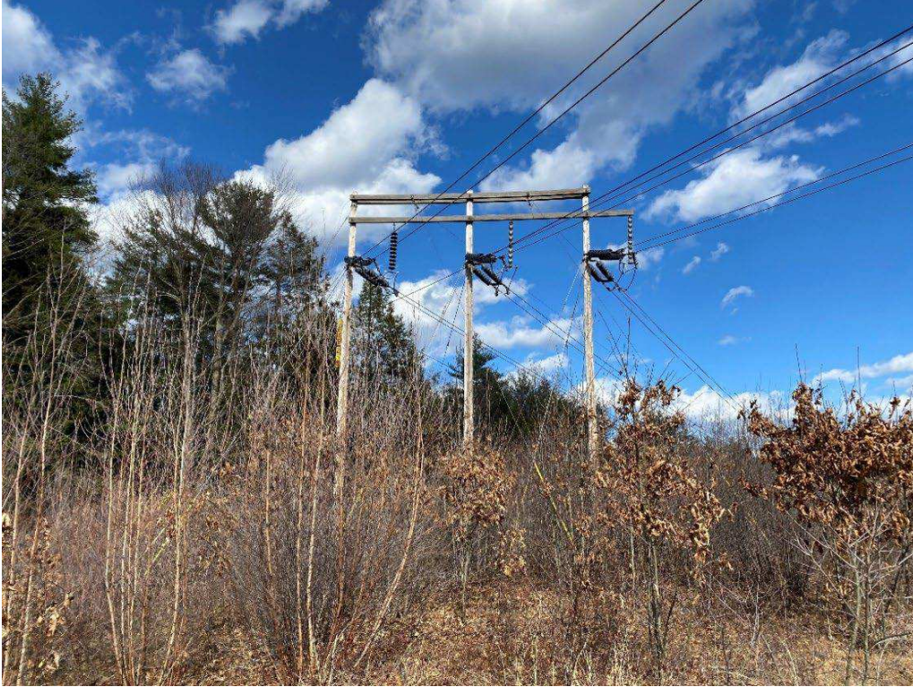
Photograph No. 3: Looking at proposed access and work pad location for N186 Structure 259.
