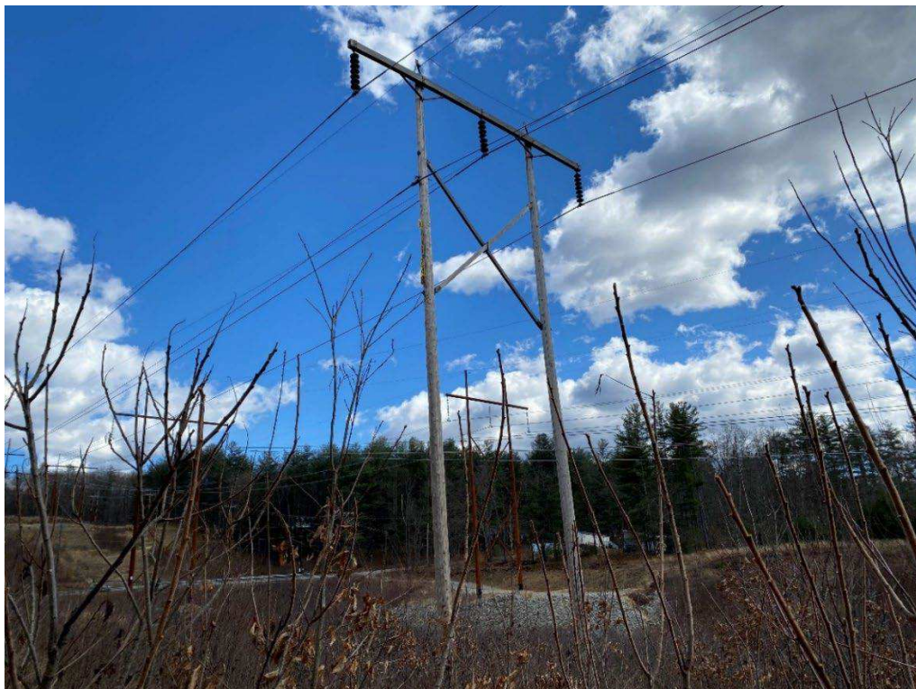
Photograph No. 8: Looking at proposed access and work pad location for N186 Structure 248.
