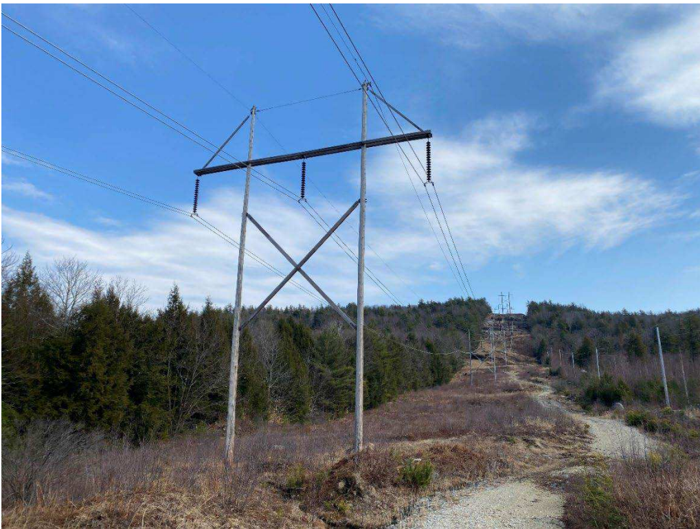
Photograph No. 26: Looking at proposed access and work pad location for 379 Structure 479.
