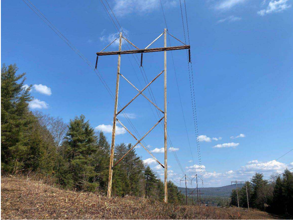
Photograph No. 21: Looking at proposed access and work pad location for 379 Structure 540.
