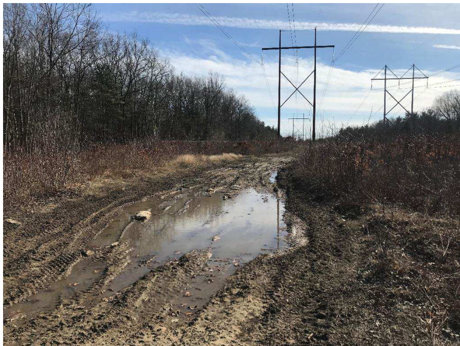
Photograph No. 2: Looking southwesterly at access to be improved towards 373 Structure 314 in Chester.
