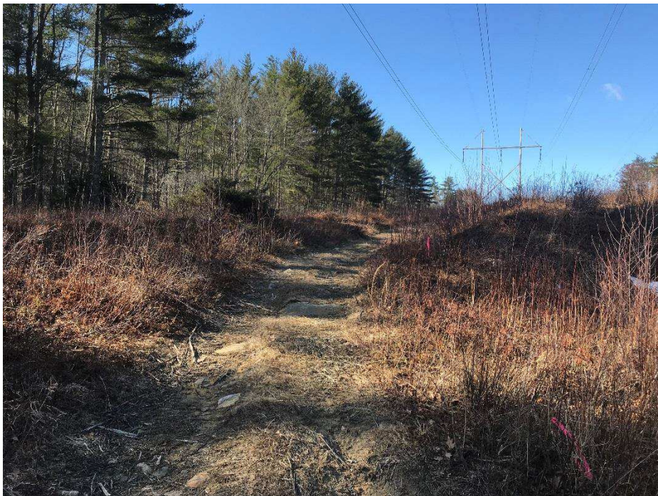
Photograph No. 18: Looking southwesterly toward 391 Structure 57 along existing access to be improved in Rochester.
