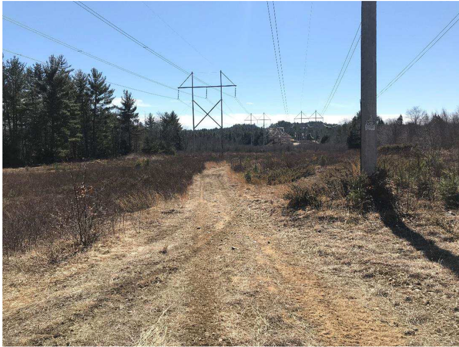
Photograph No. 9: Looking southerly toward 391 Structure 218 along existing access to be improved in Deerfield.
