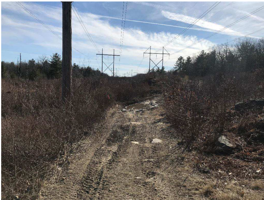
Photograph No. 4: Looking southwesterly at access to be improved by 391 Structure 306 in Chester.
