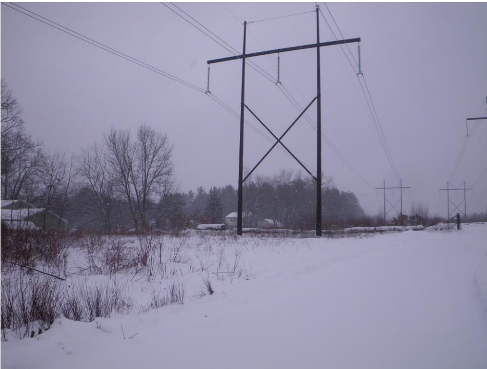
Photo 2 looking south southwest at pole 314, Ledgewood Dr in in the background.
