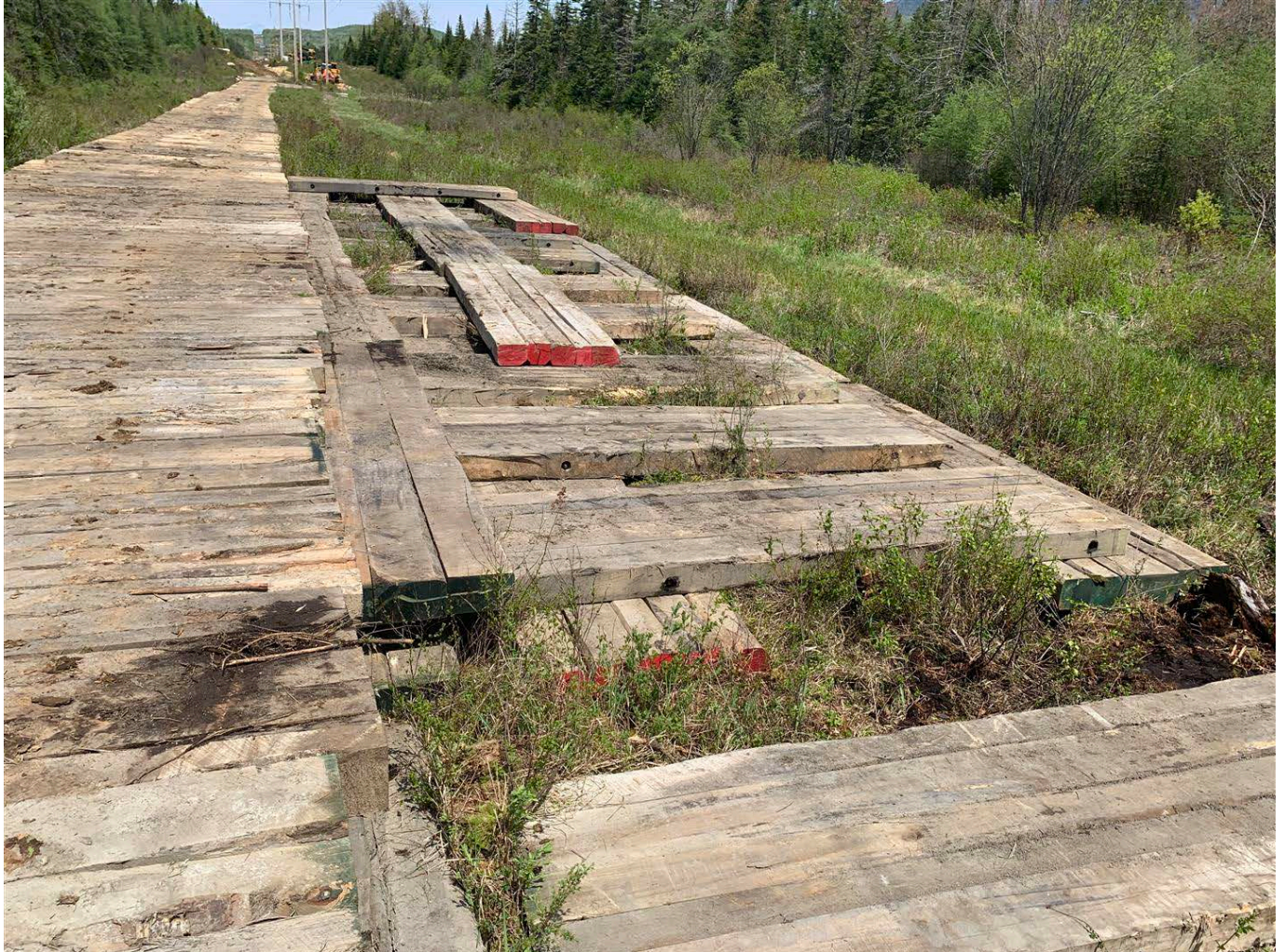
Photo 1: Example of wetland work pad creation using multiple layers of matting to elevate work surfaces and reduce ground pressure and compaction.
