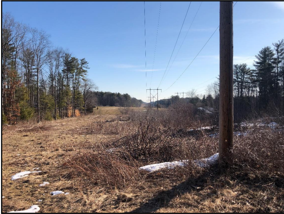
Photo 7: View east along transmission line ROW at the base of Structure 114 with Structure 113 in the background.
