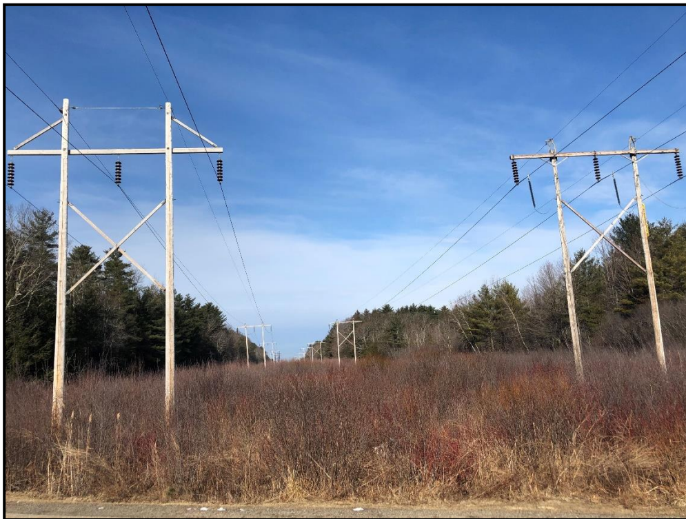
Photo 6: View west along transmission line ROW of Structures 108 and 125 from Muirfield Drive.
