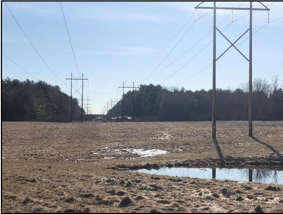
Photo 5: View east along transmission line ROW of Structure 118 with Structures 134 and 117 in the background.
