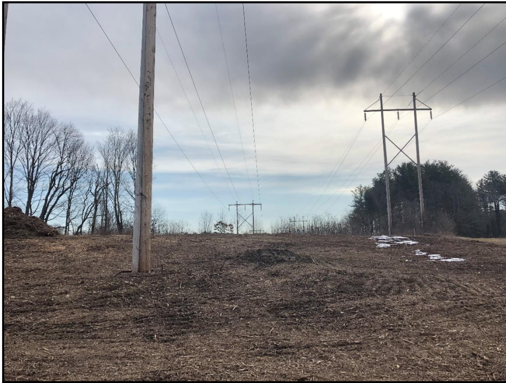
Photo 3: View east along transmission line ROW at the base of Structure 124 with Structures 124 and 141 in the background.
