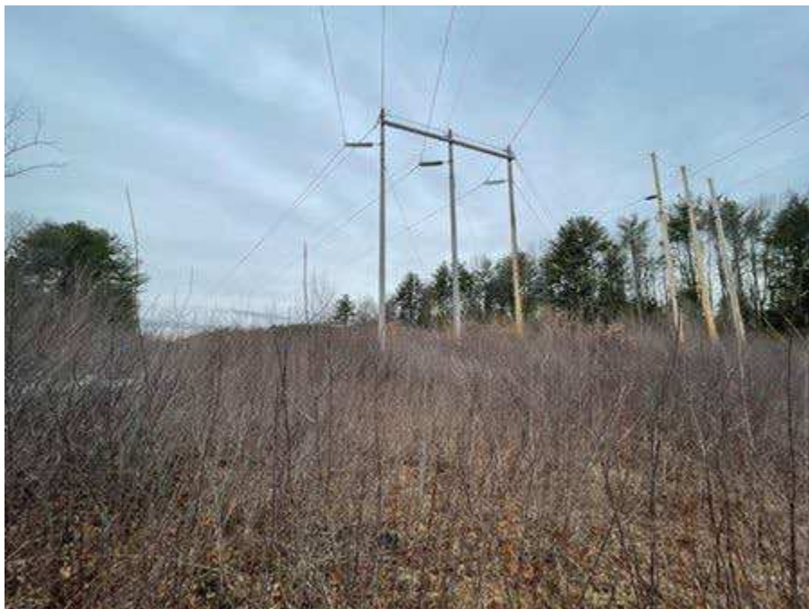
Photo 6. Str. 142 (H141 line) future work area, viewing northwest.
