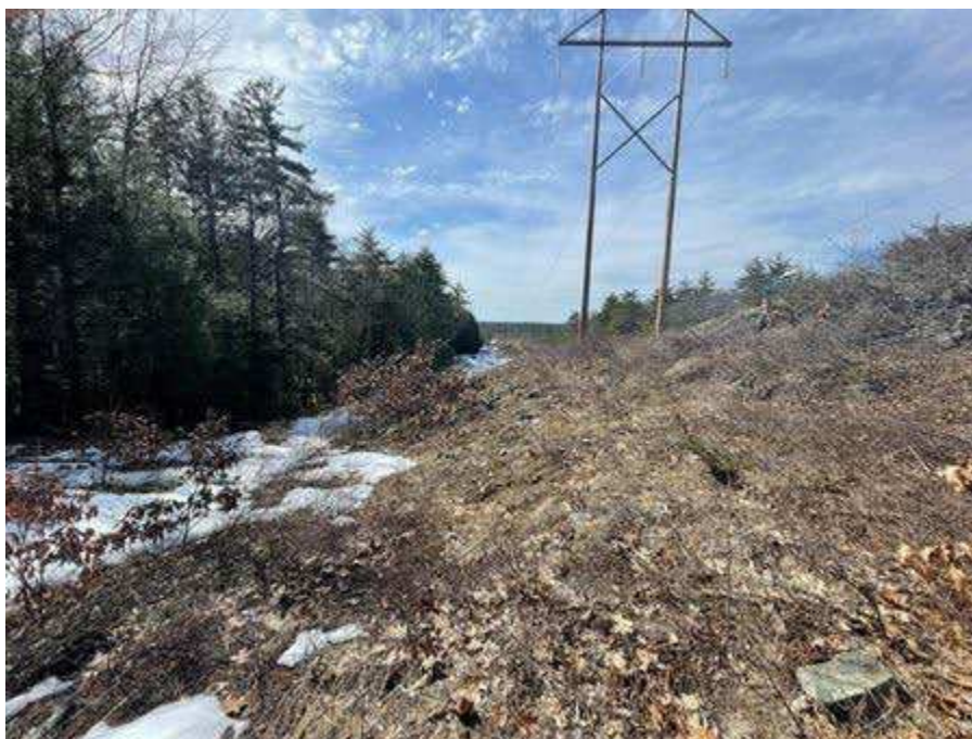
Photo 44. Proposed access road to immediate left of Str. 159, H141 line, viewing west. Existing trail with steep grade to far left.
