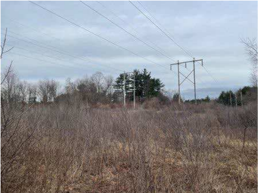
Photo 3. Proposed access route between Newfields Road and Str. 141 (H141 line), viewing west.
