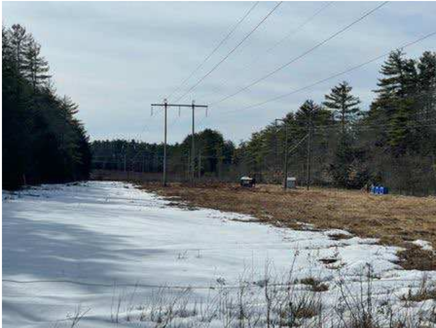
Photo 51. Proposed access route between existing improved road off Beechhill Road and Strs. 163 (H141 line) and 183 (A126 line), viewing west. Please note, ability to thoroughly photograph access routes and future work areas for Strs. 163-164 (H141 line) and 183-184 (A126 line) due to electric fence on property.
