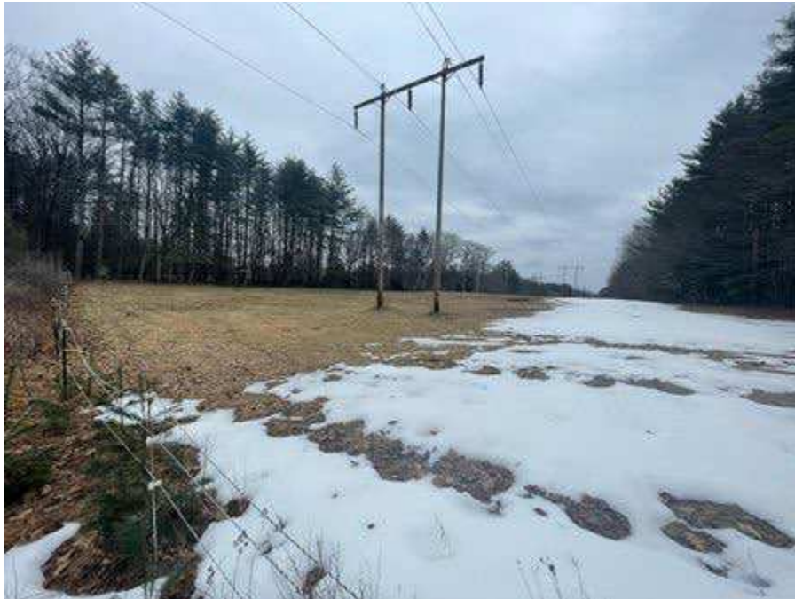
Photo 89. Str. 213 (H141 line) future work area, viewing northeast. Please note, private electric fence blocking further entry visible in bottom left of photo.
