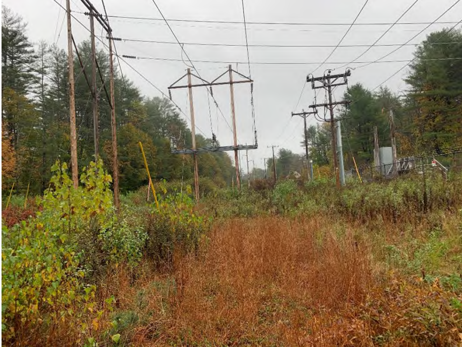
Photograph No. 49: Looking northeasterly at proposed pad location at Structures 70, 70A, 70B, & 71.
