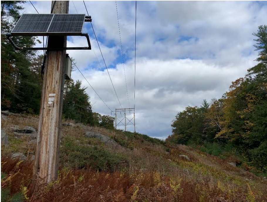
Photograph No. 20: Looking northerly at proposed access and pad location for Structure 38.
