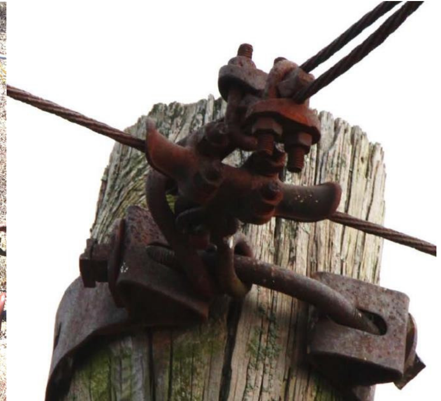
Line 1756 Rusting and Pitting on Shield wire & Hardware
