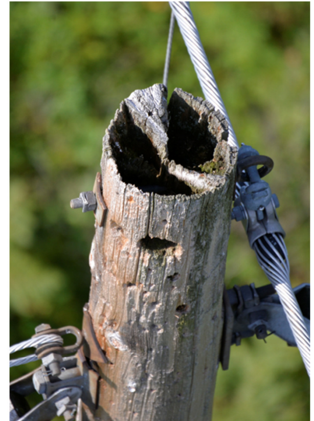
Line 1161 Str 40079 Deep Pole Top Rot
