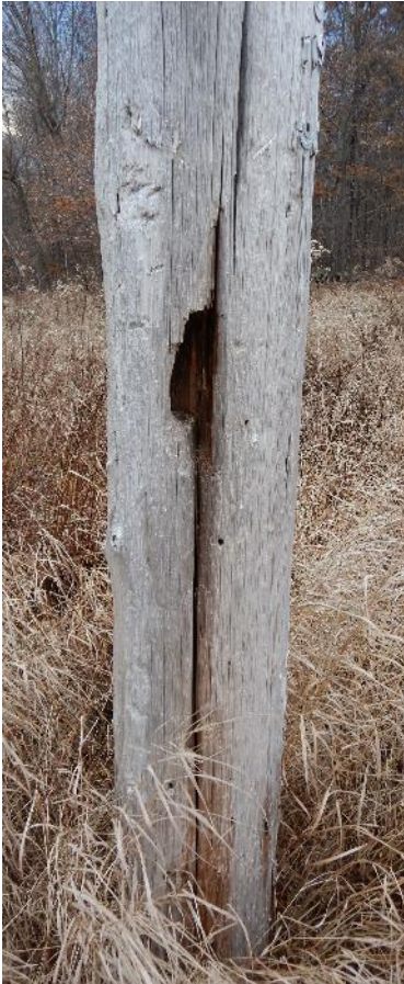
Line K174 Str 119 Pole Base Splitting
