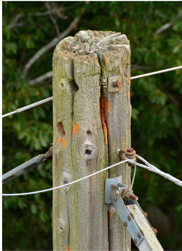
Line 1080 Str 6351 Pole Crack & Woodpecker Holes
