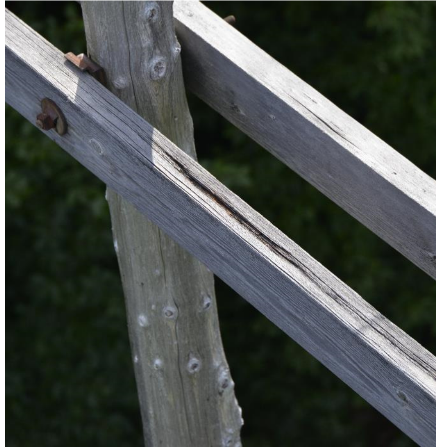
Line 1421 Str 32008 Cross Arm Splitting
