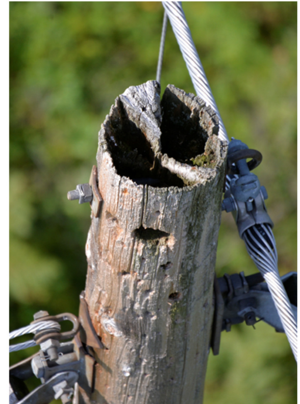
Line 1161 Str 40079 Deep Pole Top Rot
