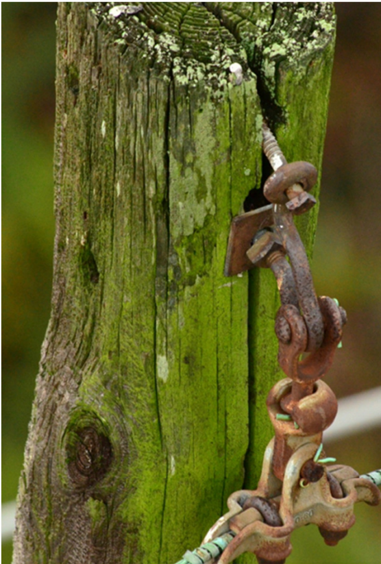
Line 1000 Str 7619 Pole Crack
