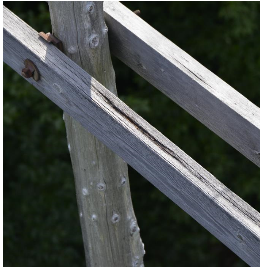
Line 1421 Str 32008 Cross Arm Splitting
