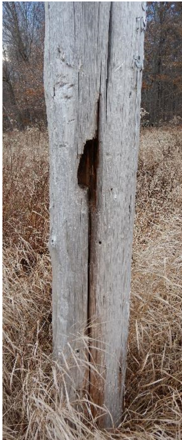
Line K174 Str 119 Pole Base Splitting
