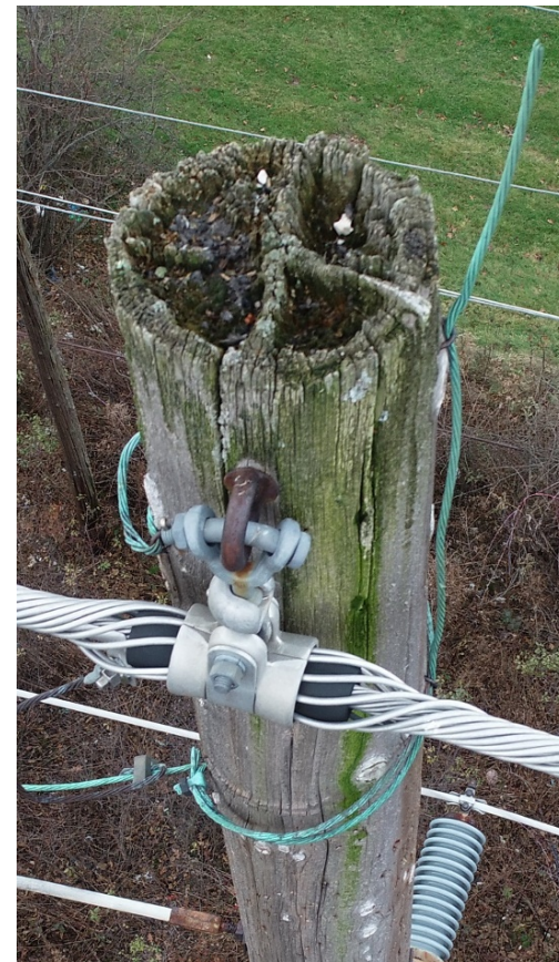
Split Pole Top, Cracks, Decay – Line 1751, Structure #3-363
