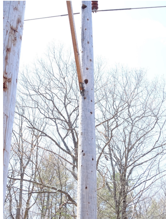
Woodpecker Damage – Line D121, Structure #77
