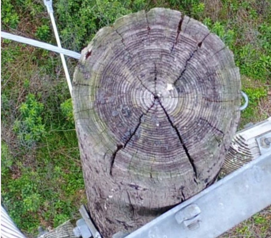
Pole Top Split – Line 456-522, Structure #2
