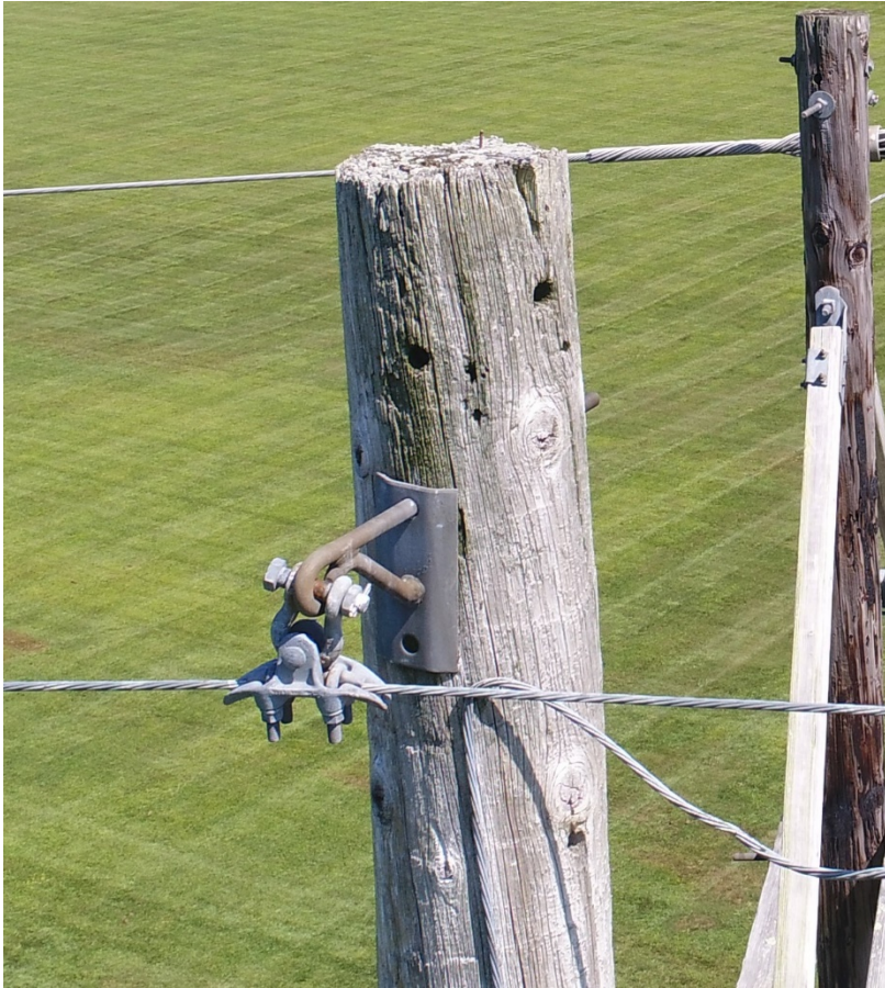
Woodpecker Damage – Line 240-510, Structure #185
