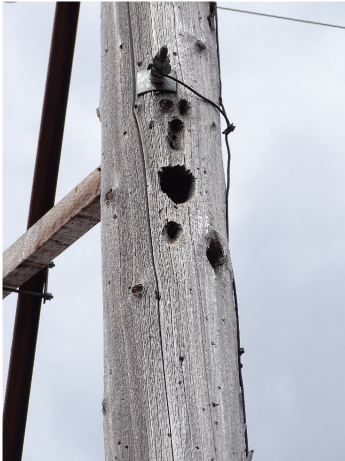
Woodpecker Damage – Line D121, Structure #46
