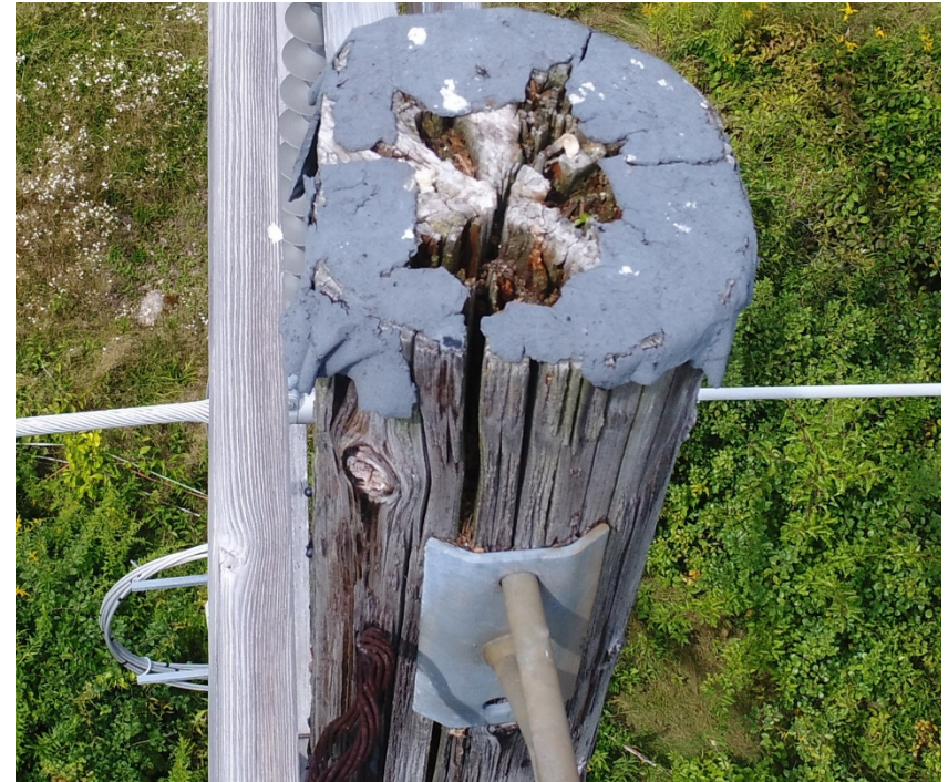
Pole Top Rot – Line 240-510, Structure #197
