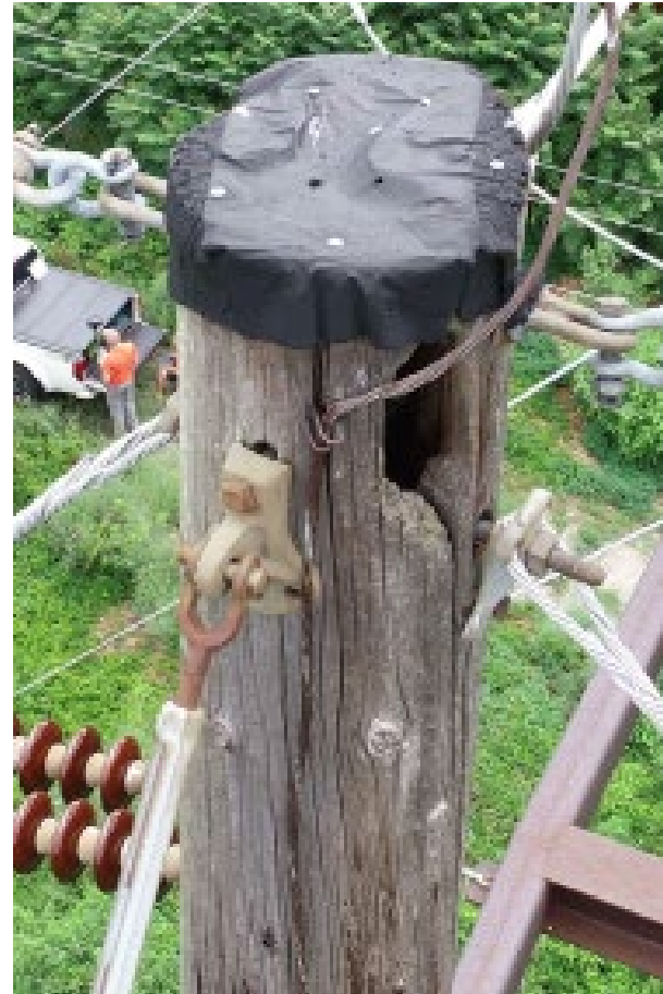
Woodpecker Damage – Line 342-603, Structure #101
