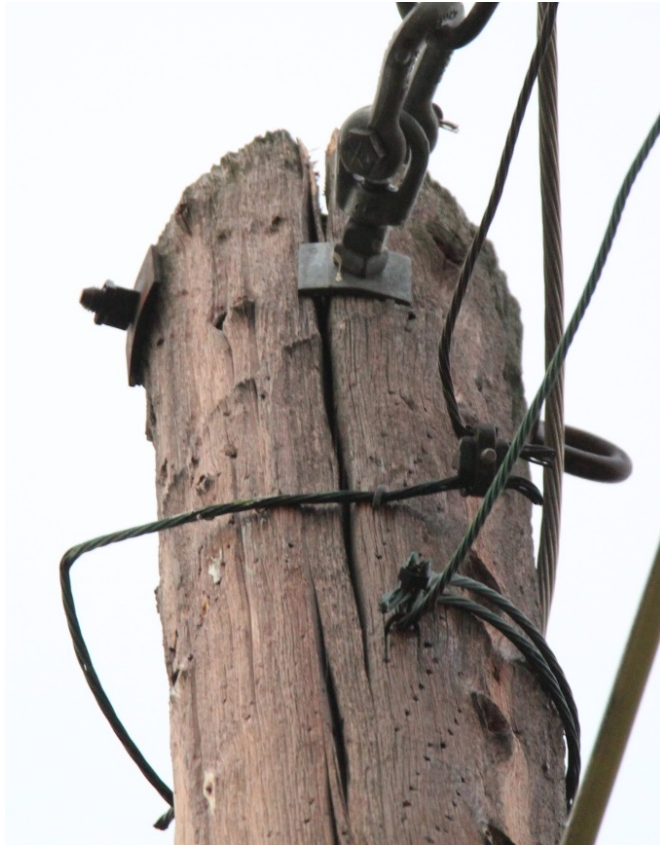
Split Pole Top, Cracks, Decay – Line 1751, Structure #3-331
