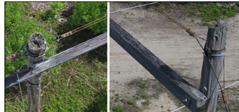
E115 Structure #160 – Split pole tops, crossarm rot, shell rot, cracks
