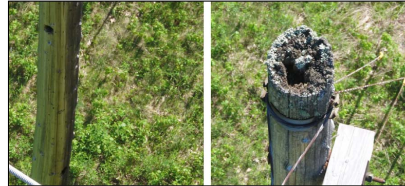
A111 Structure #64 – Split pole tops, woodpecker damage, cracks
