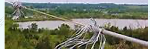
Figure A-75. Damaged conductor following the 2013 tornado.
