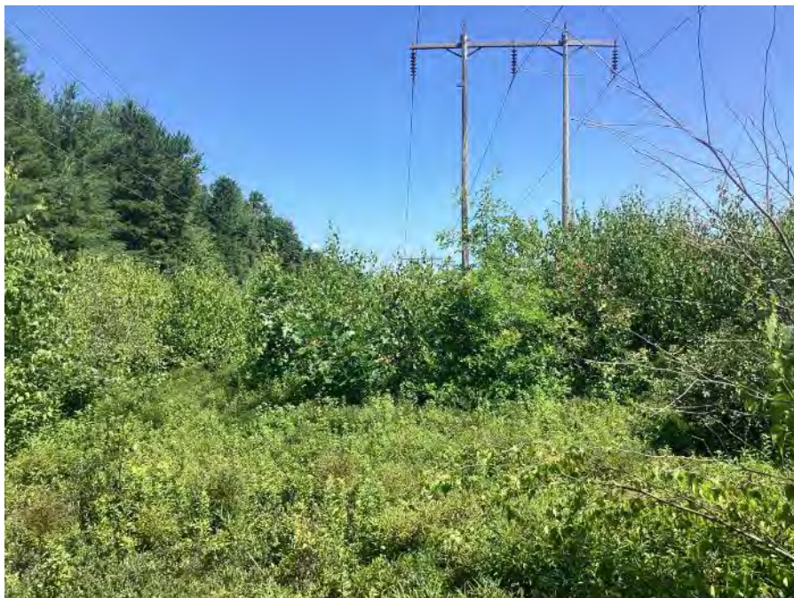
Photo 8. Louden Road to Soucook River Segment: shrub-dominated ROW, view to the north at structure 95. Stantec. July 19, 2022.
