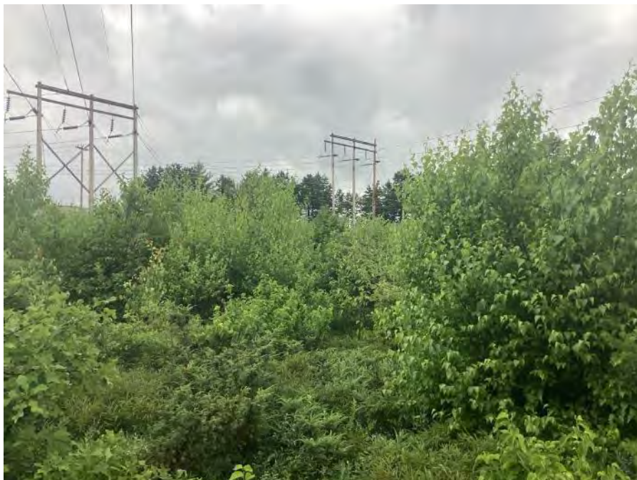
Photo 10. Louden Road to Soucook River Segment: shrub-dominated ROW, view to the south to structure 89. Stantec. July 18, 2022.
