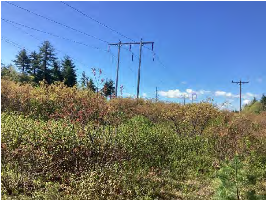
Photo 20. Soucook River to Pembroke Street Segment: scrub oak-dominated ROW near structure 72, view to the south. Stantec. May 17, 2022.
