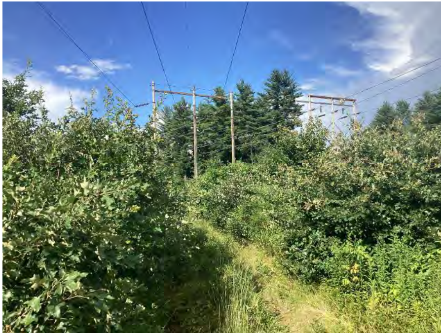
Photo 36. Soucook River to Pembroke Street Segment: scrub oak-dominated ROW near structure 60, view to the northeast. Stantec. July 21, 2022.
