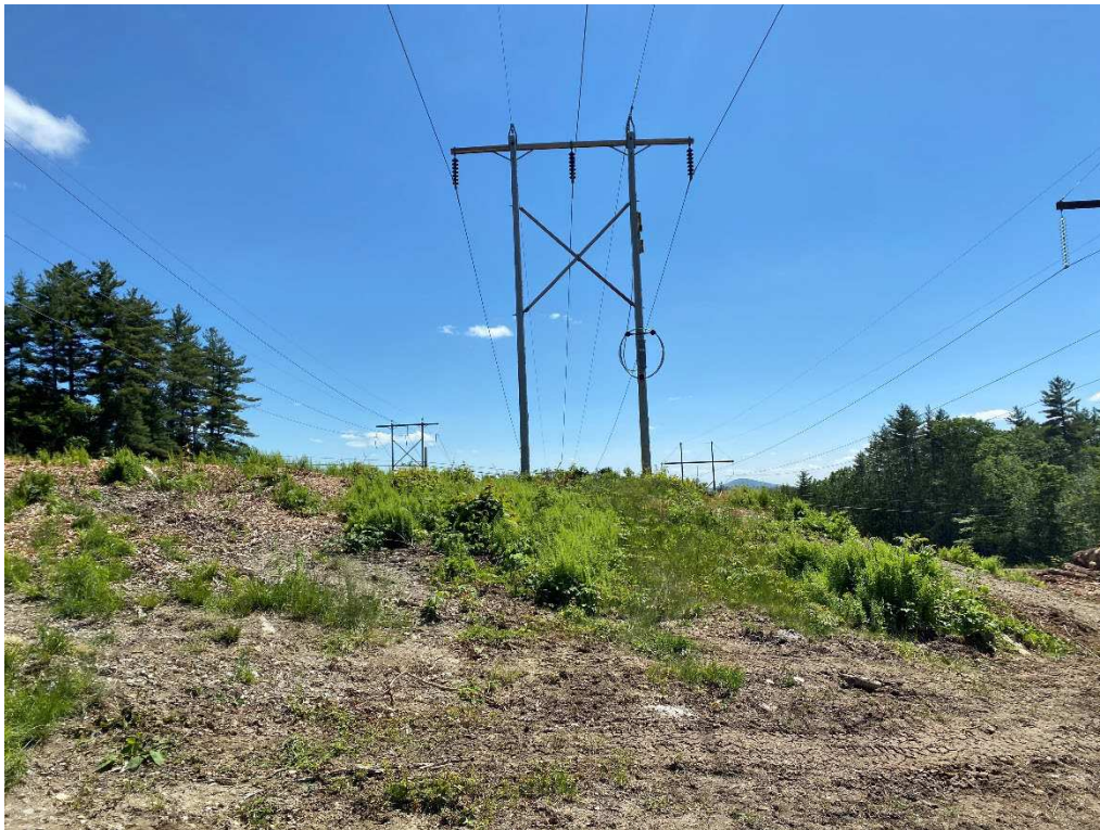
Photograph No. 50: Looking at proposed access and work pad location for C196 Structure 74.
