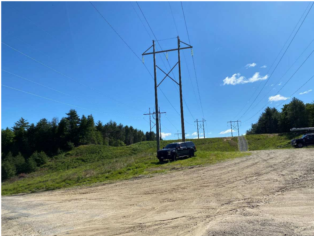
Photograph No. 74: Looking at proposed access and work pad location for C196 Structure 38.
