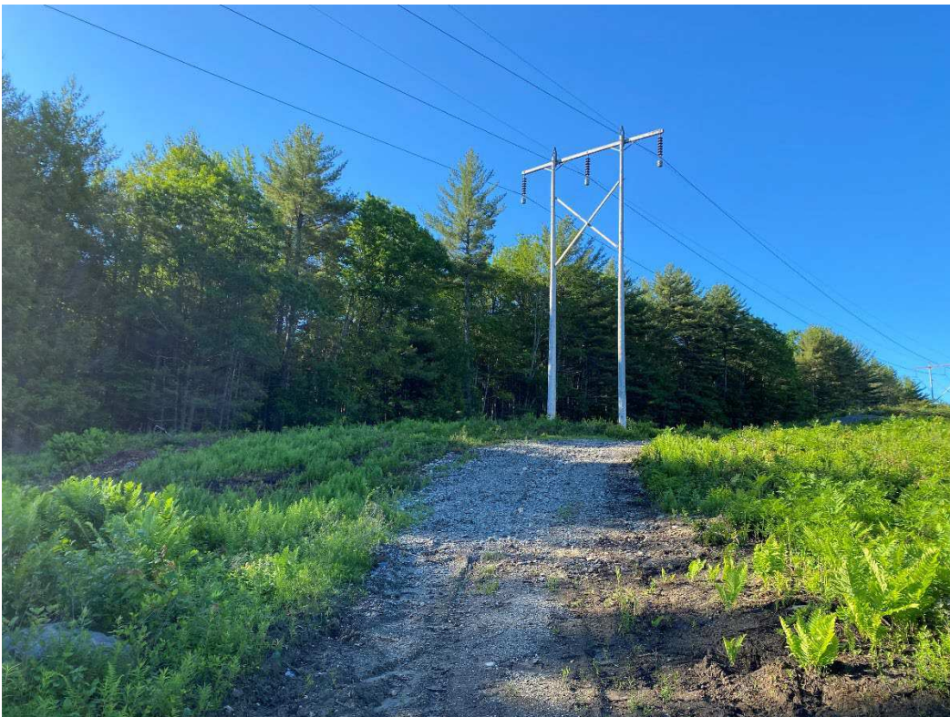
Photograph No. 64: Looking at proposed access and work pad location for Q171 Structure 63.
