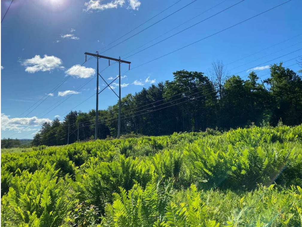
Photograph No. 67: Looking at proposed access and work pad location for C196 Structure 49.
