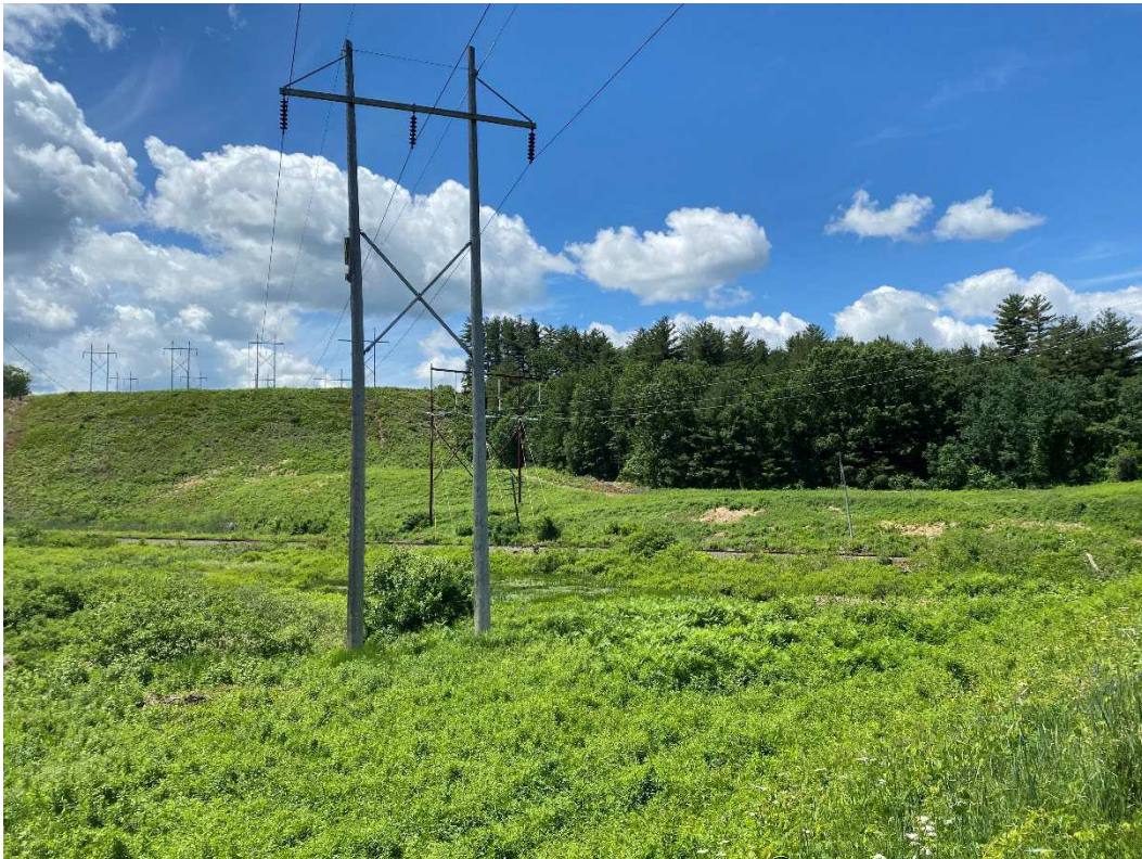
Photograph No. 84: Looking at proposed access and work pad location for C196 Structure 4.
