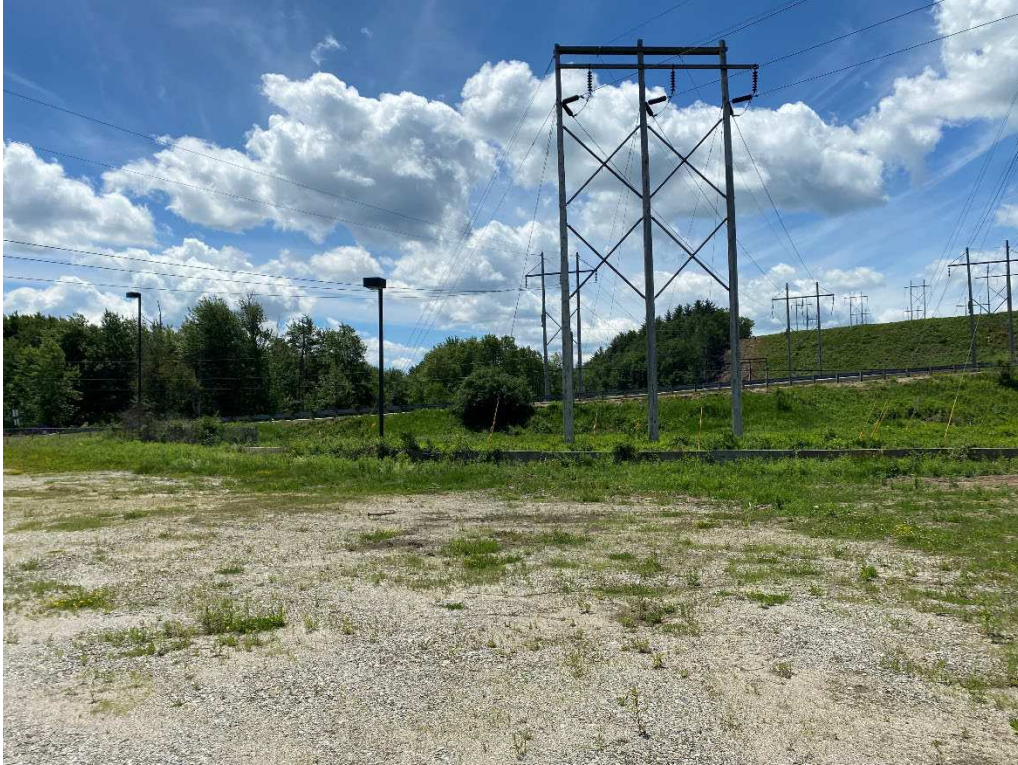
Photograph No. 85: Looking at proposed access and work pad location for Q171 Structure 3.
