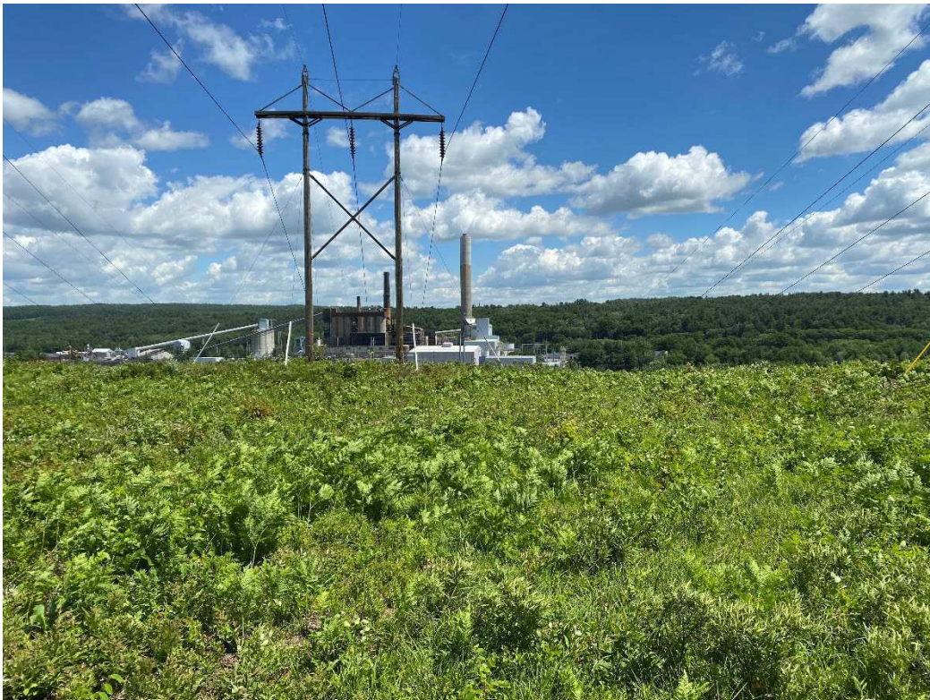
Photograph No. 82: Looking at proposed access and work pad location for Q171 Structure 5.
