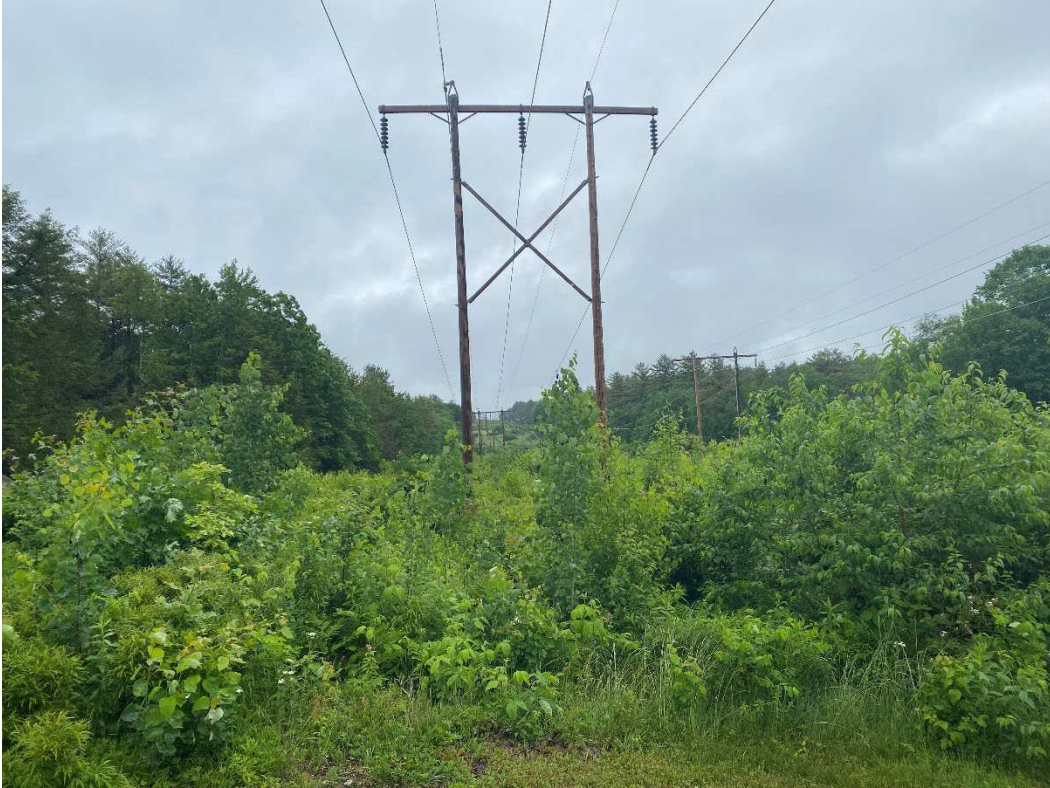
Photograph No. 21: Looking at proposed access and work pad location for C196 Structure 125.
