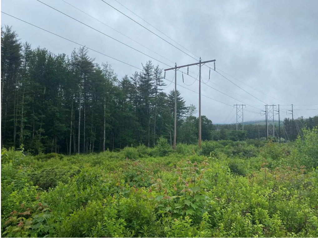
Photograph No. 5: Looking at proposed access and work pad location for Q171 Structure 137.
