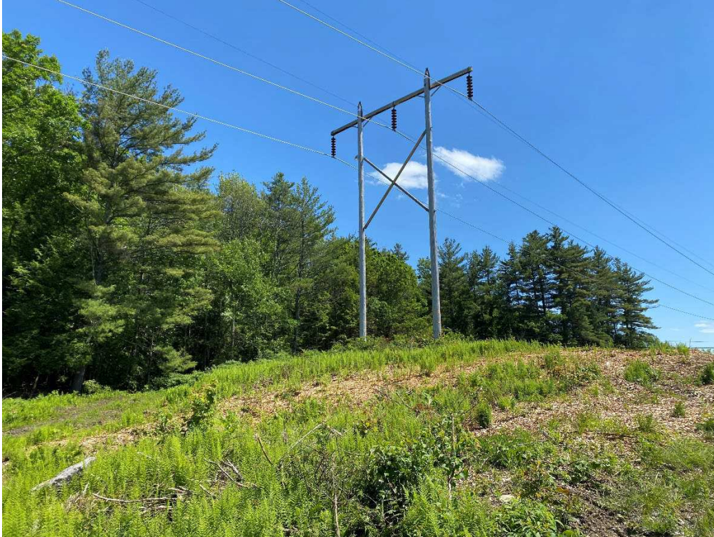
Photograph No. 51: Looking at proposed access and work pad location for Q171 Structure 73.
