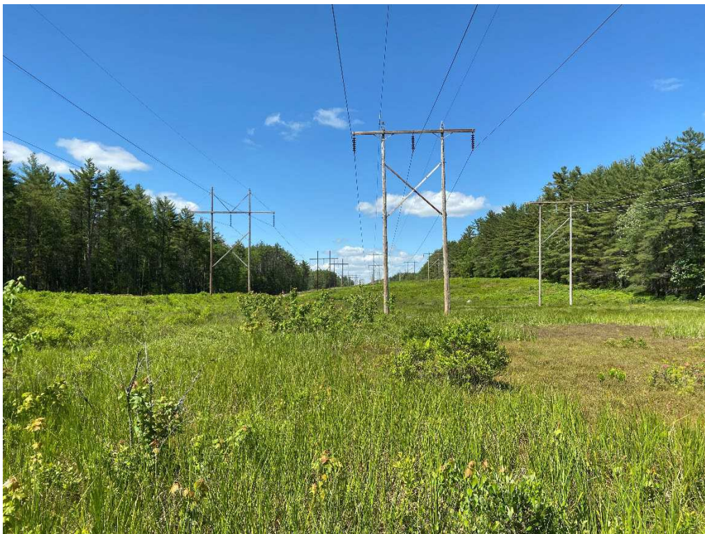
Photograph No. 58: Looking at proposed access and work pad location for C196 Structure 68 (center).
