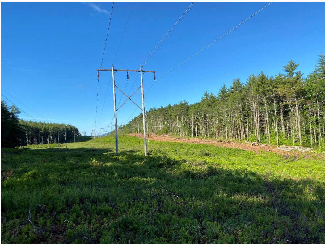
Photograph No. 60: Looking at proposed access and work pad location for C196 Structure 67.
