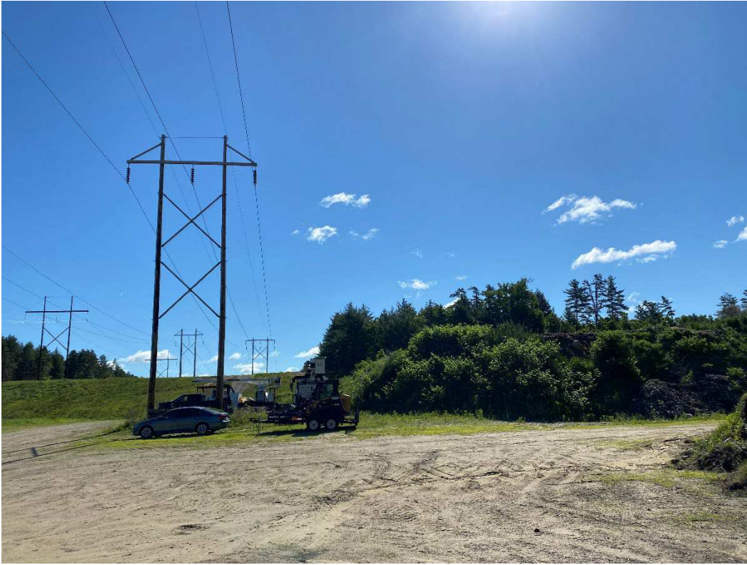
Photograph No. 73: Looking at proposed access and work pad location for Q171 Structure 39.
