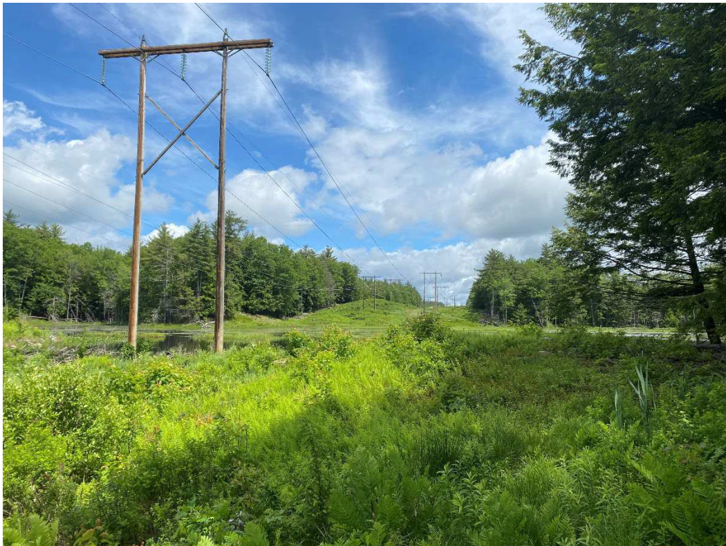
Photograph No. 44: Looking at proposed access and work pad location for Q171 Structure 87.
