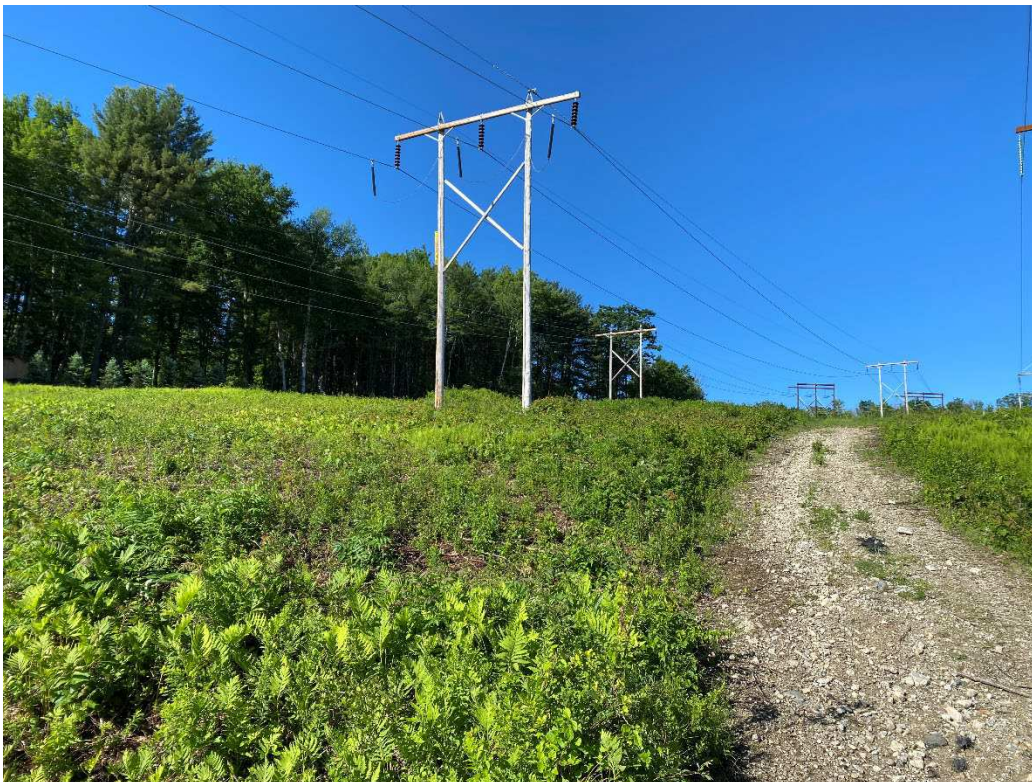
Photograph No. 68: Looking at proposed access and work pad location for C196 Structure 48.
