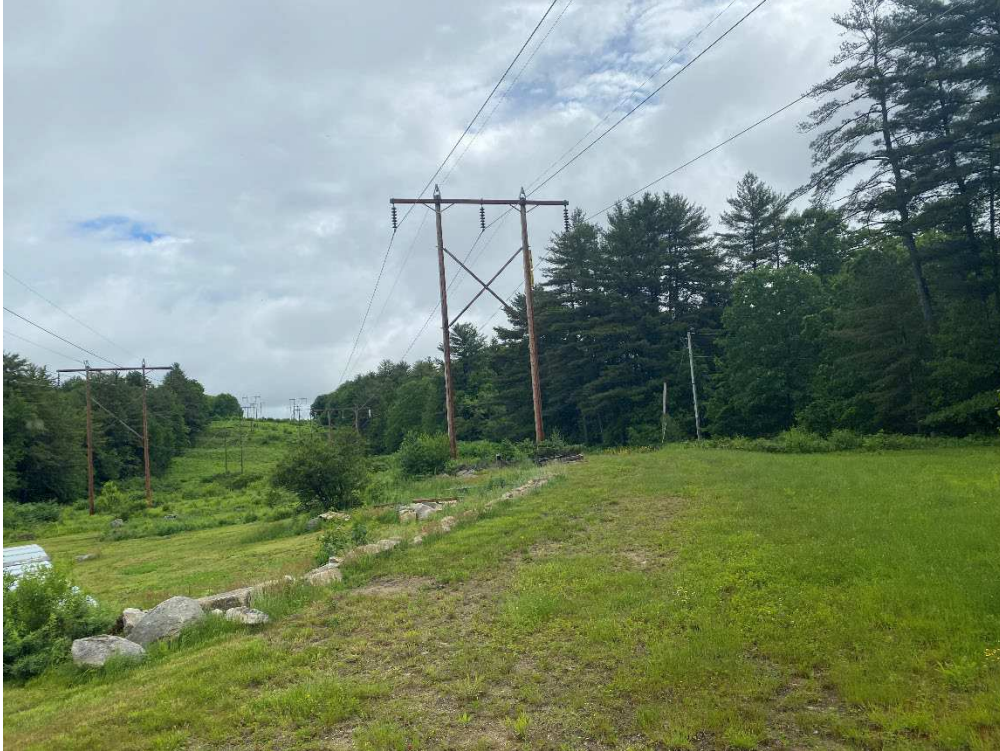
Photograph No. 27: Looking at proposed access and work pad location for Q171 Structure 111.
