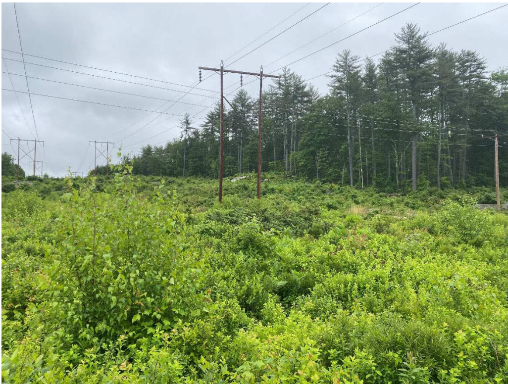
Photograph No. 6: Looking at proposed access and work pad location adjacent to Q171 Structure 136.
