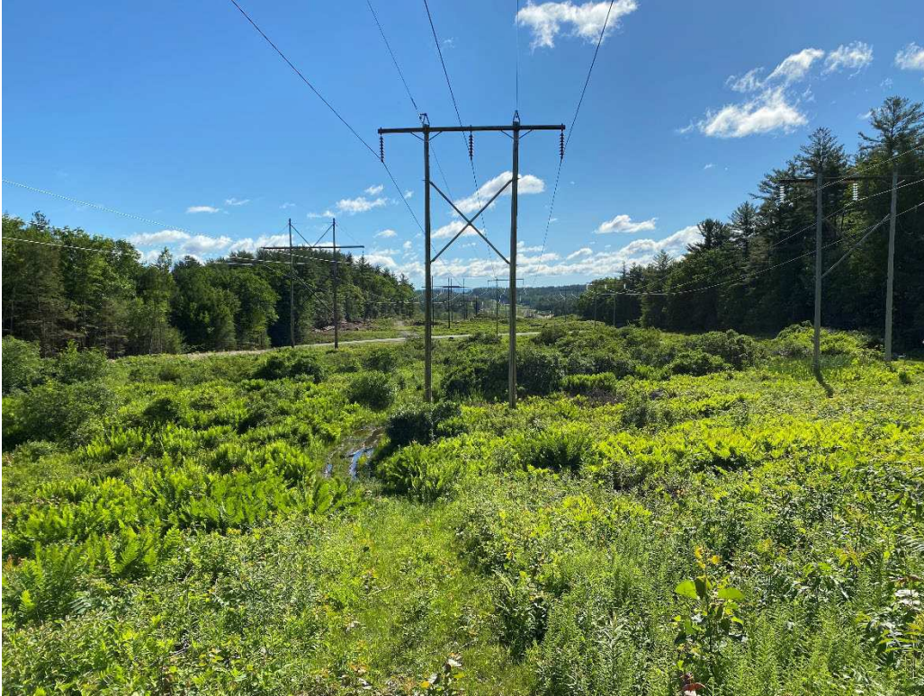
Photograph No. 69: Looking at proposed access and work pad location for C196 Structure 47.
