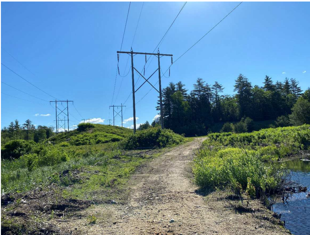
Photograph No. 72: Looking at proposed access and work pad location for Q171 Structure 43.
