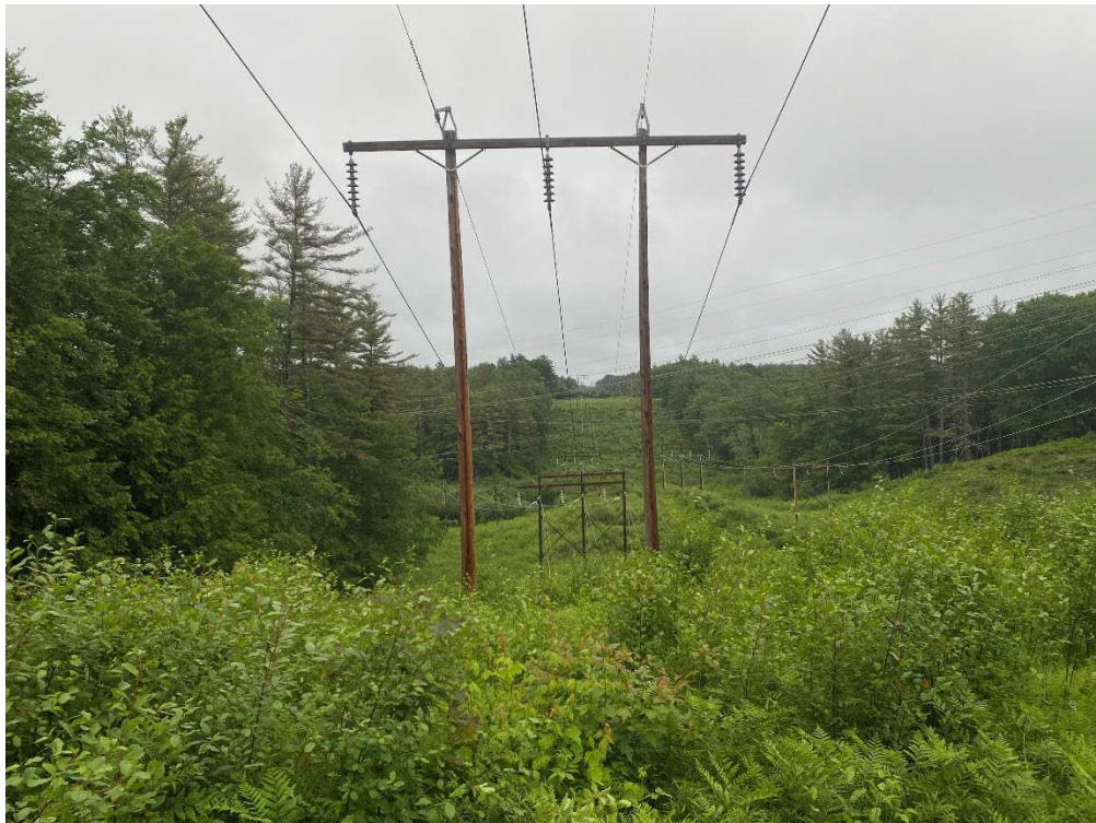
Photograph No. 14: Looking at proposed access and work pad location for C196 Structure 132.
