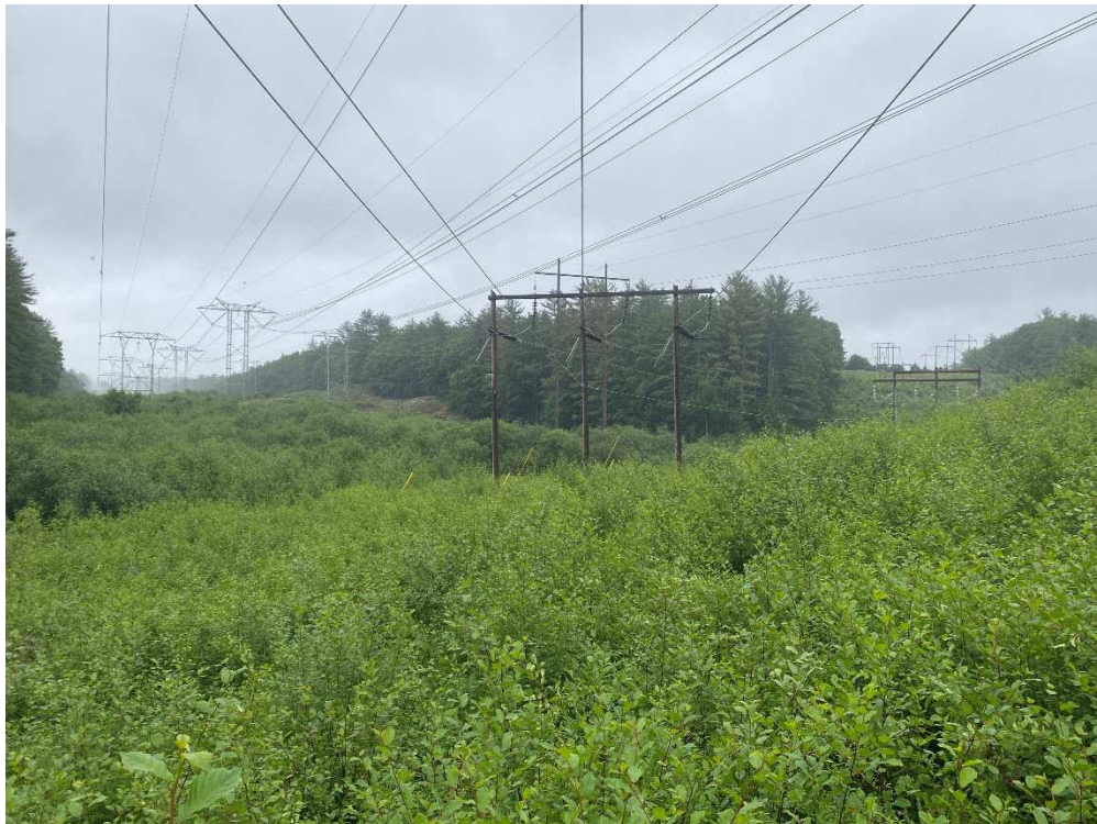
Photograph No. 16: Looking at proposed access and work pad location for C196 Structure 130.
