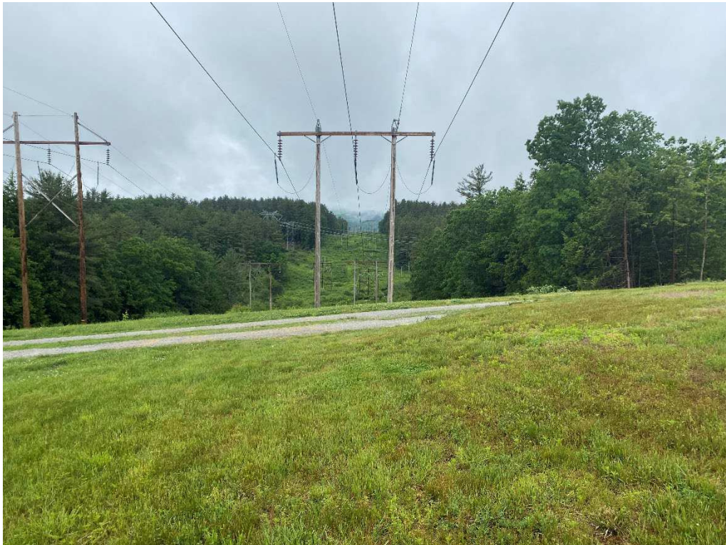
Photograph No. 18: Looking at proposed access and work pad location for C196 Structure 127.
