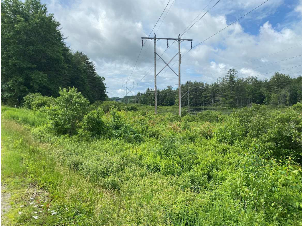
Photograph No. 33: Looking at proposed access from Montelona Road to Q171 Structure 92.
