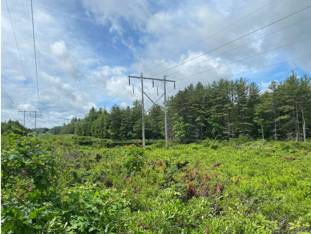
Photograph No. 31: Looking at proposed access and work pad location for C196 Structure 96.
