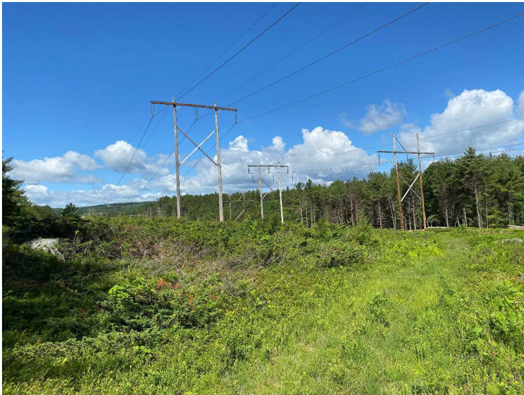
Photograph No. 76: Looking at proposed access and work pad location for Q171 Structure 34.
