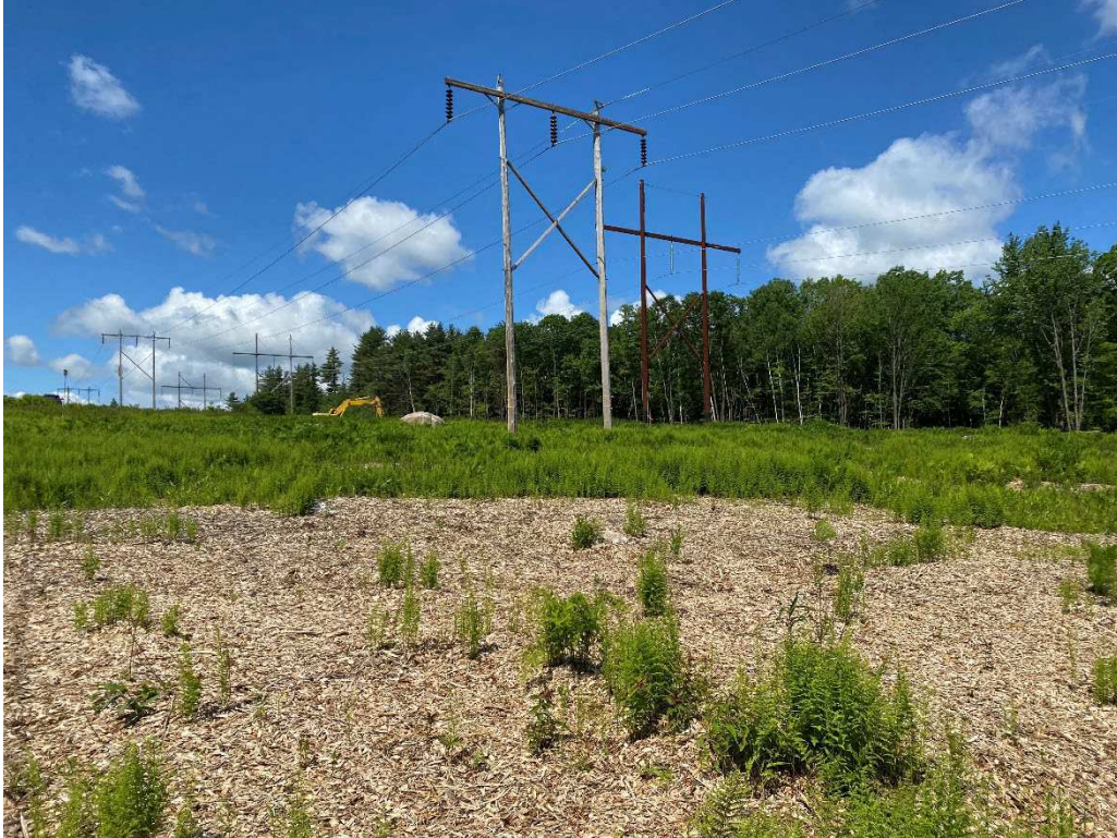
Photograph No. 79: Looking at proposed access and work pad location for C196 Structure 22.
