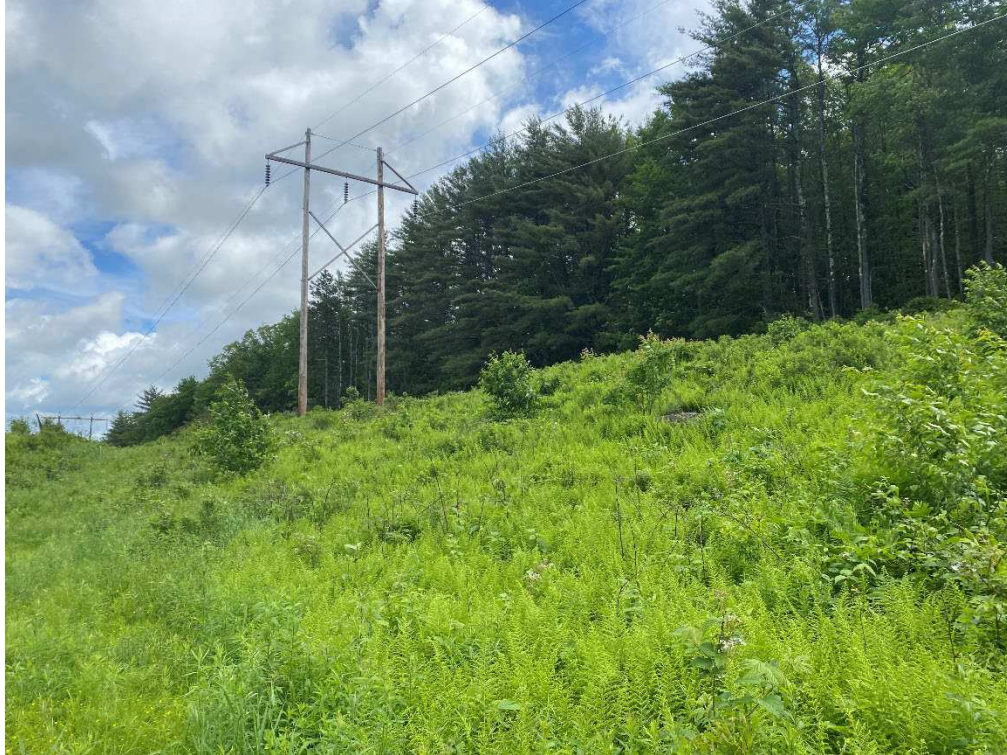
Photograph No. 39: Looking at proposed access and work pad location for Q171 Structure 89.
