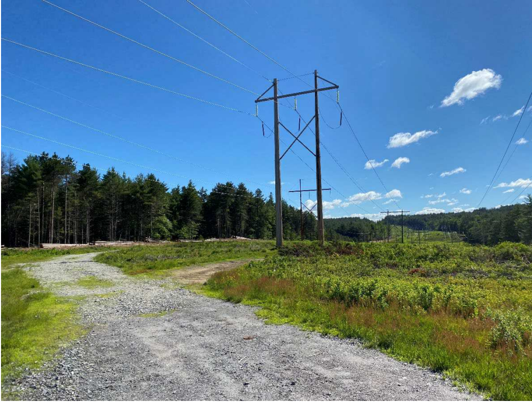
Photograph No. 75: Looking at proposed access and work pad location for C196 Structure 37.
