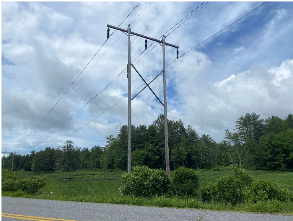
Photograph No. 34: Looking at proposed access and work pad location from Montelona Road for C196 Structure 94.
