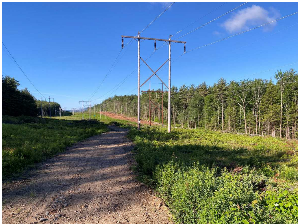
Photograph No. 62: Looking at proposed access and work pad location for C196 Structure 66.
