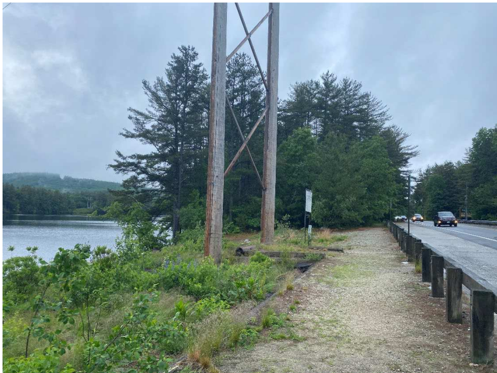
Photograph No. 2: Looking at proposed access and work pad location from Elm Street for C196 Structure 143. 04.0191410.18 GZA GeoEnvironmental, Inc.
