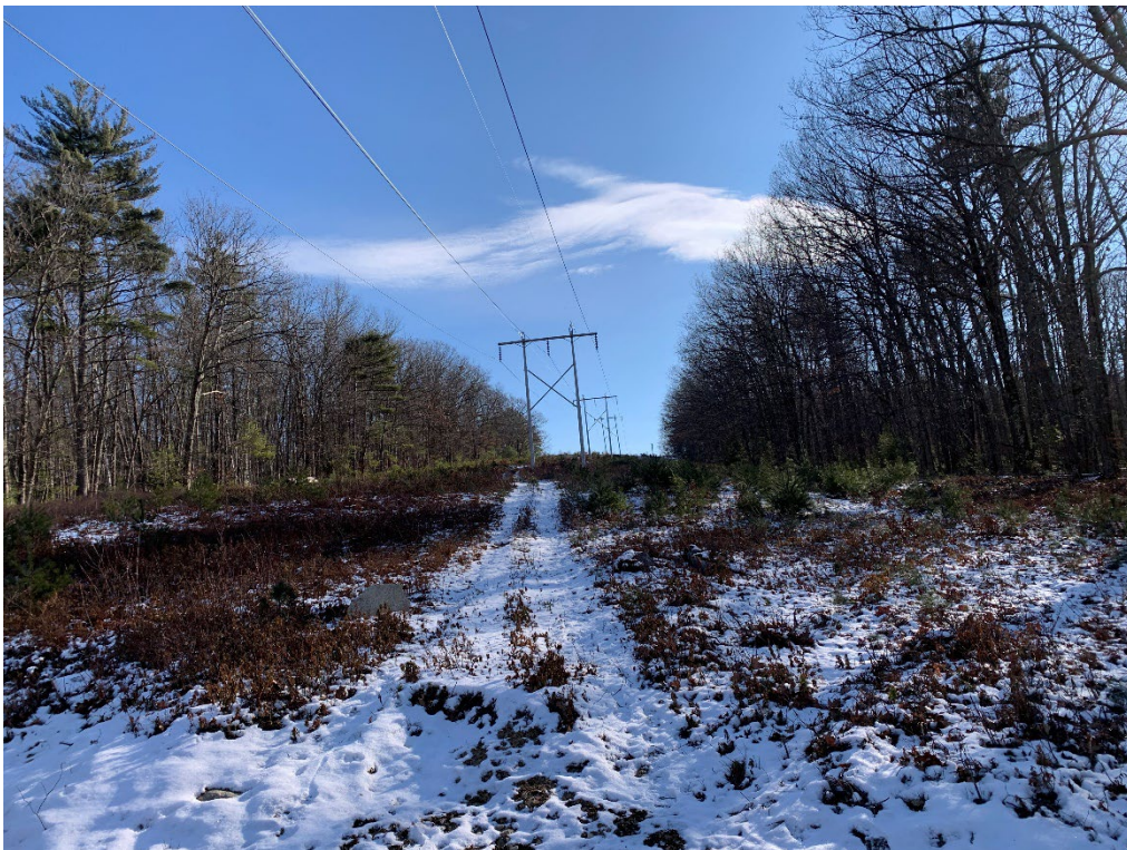
Photograph No. 4: Looking at proposed access and work pad location for Structure 78.
