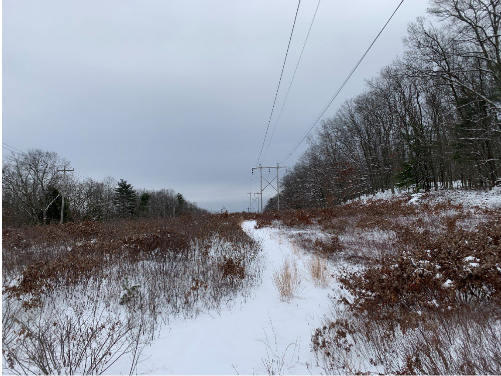
Photograph No. 13: Looking at proposed access and work pad location for Structure 111.
