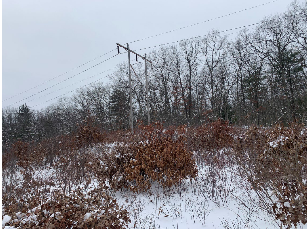
Photograph No. 15: Looking at proposed access and work pad location for Structure 113.
