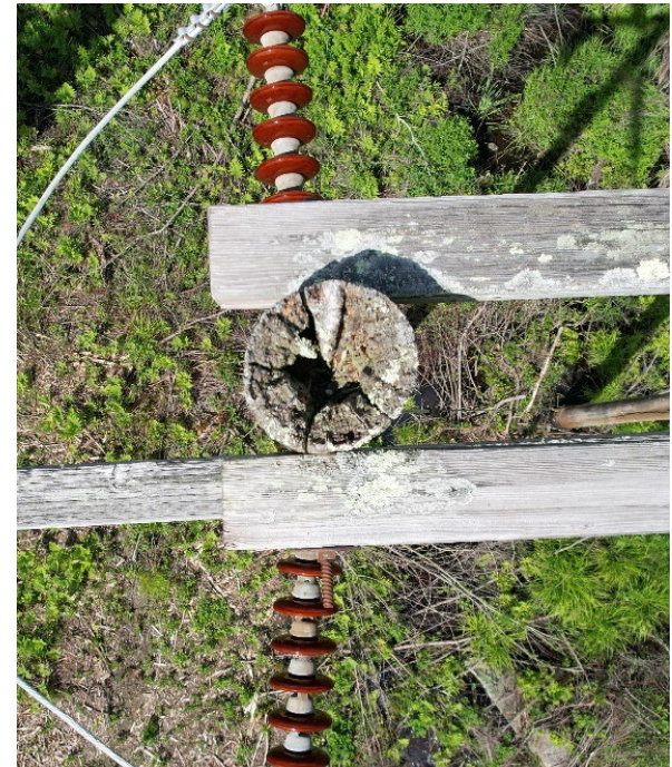
Line M-183 Structure 1 Pole Top Rotted and Split
