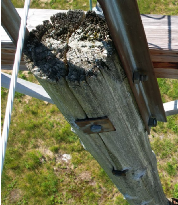
Line F-139 Structure 191 Decay, Woodpecker Damage
