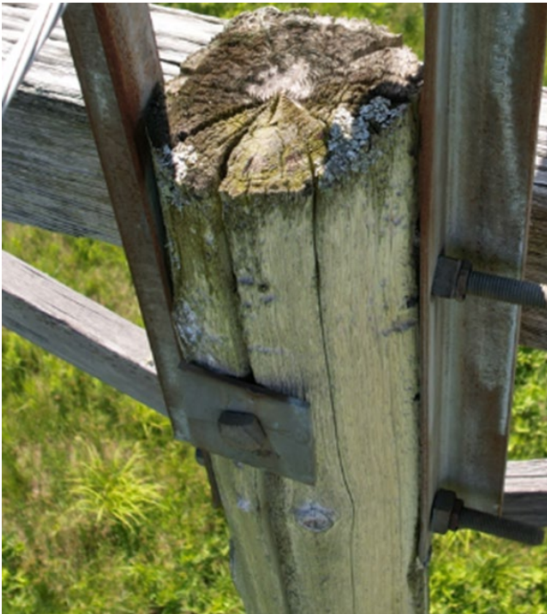
Line F-139 Structure 197 Significant Rot, Split Pole Top
