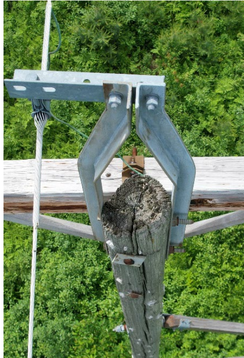
Line M-183 Structure 19 Splitting and Pole Top Rot
