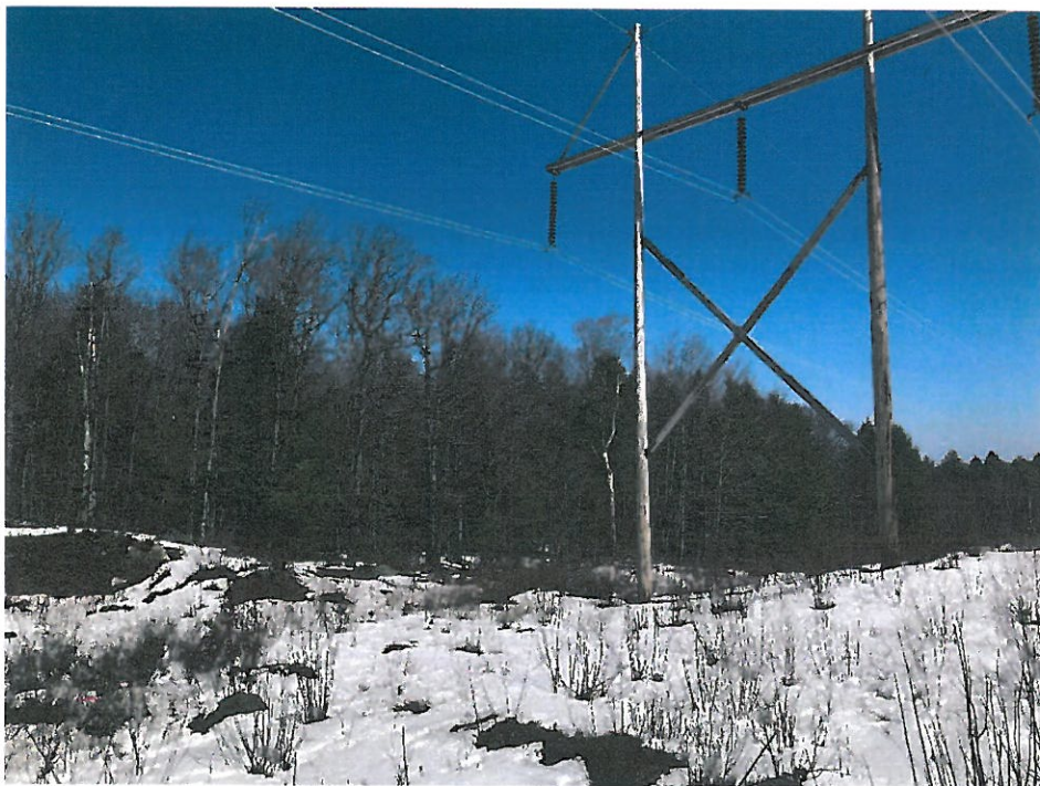
Photograph No. 20: Looking northeasterly at Wetland IW-13.1 (left) and Structure 283 (right) to be replaced.
