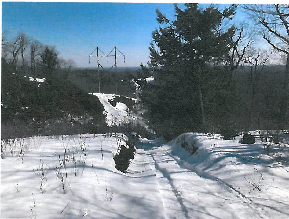
Photograph No. 12: Looking easterly at proposed access route toward Structure 288 to be replaced.
