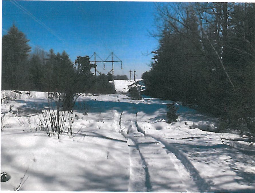
Photograph No. 15: Looking easterly at proposed access route through Wetland IW-18 toward Structure 287 to be replaced. Timber matting will be used through the wetland portion of the access road.
