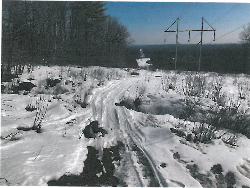
Photograph No 11: Looking easterly at proposed access route through Wetland IW-20 towards Structure 289. Timber matting will be used through the wetland portion of the access road.
