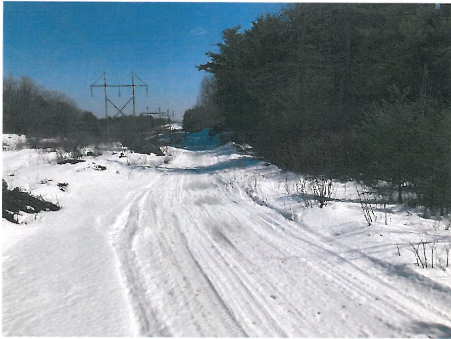
Photograph No. 19: Looking easterly at proposed access route through Wetland IW-14 toward Structure 283 to be replaced. Timber matting will be used through the wetland portion of the access road.
