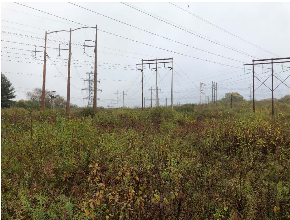
Photograph No. 2: Easterly view of E194 Structure 3 (center) to be replaced within Wetland PW-28.
