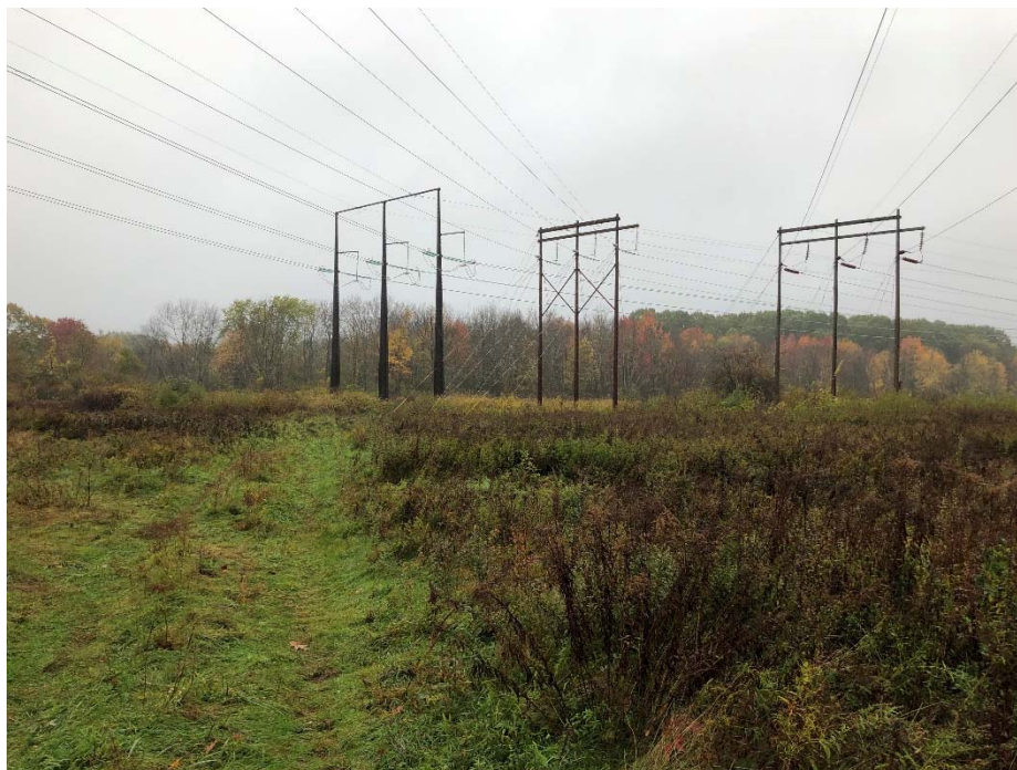
Photograph No. 12: Southeasterly view of proposed access in the 100-foot wetland buffer of Wetland PW-6 for 3135 Structure 105 and 106 to be replaced.
