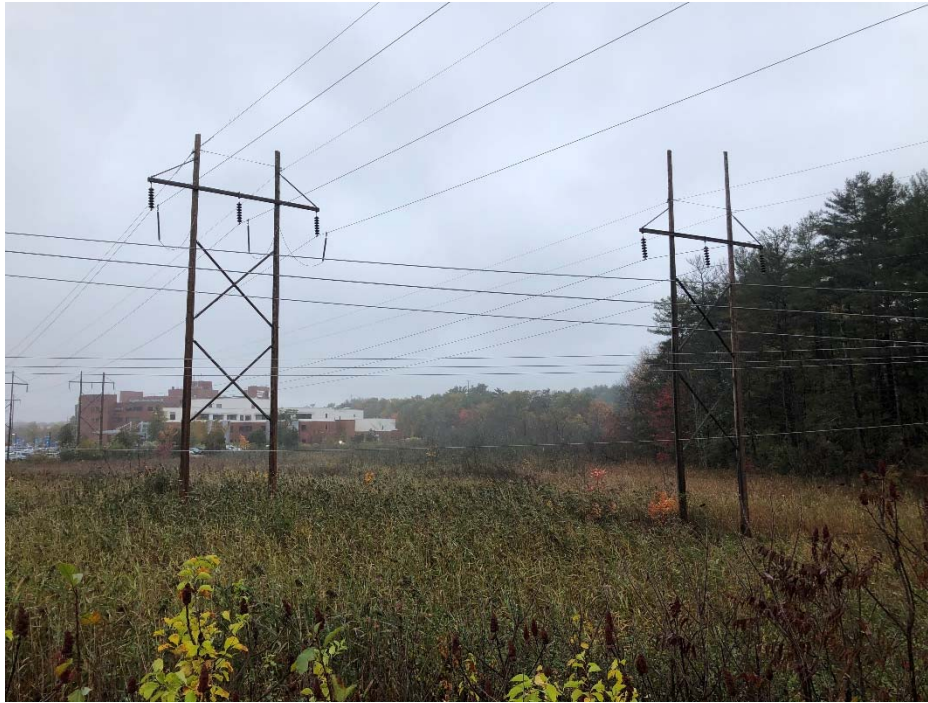
Photograph No. 5: Southwesterly view of E194 Structure 35 (right) and U181 Structure 35 (left) to be replaced within Wetland PW-11.
