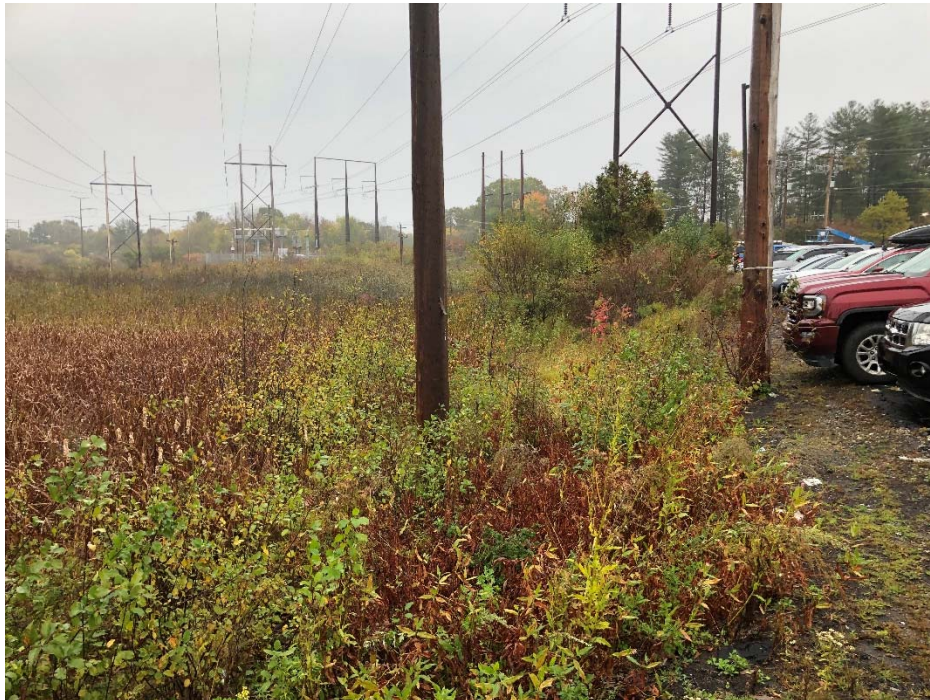
Photograph No. 7: Easterly view of Wetland PW-11 (left) and U181 Structure 36 to be replaced.
