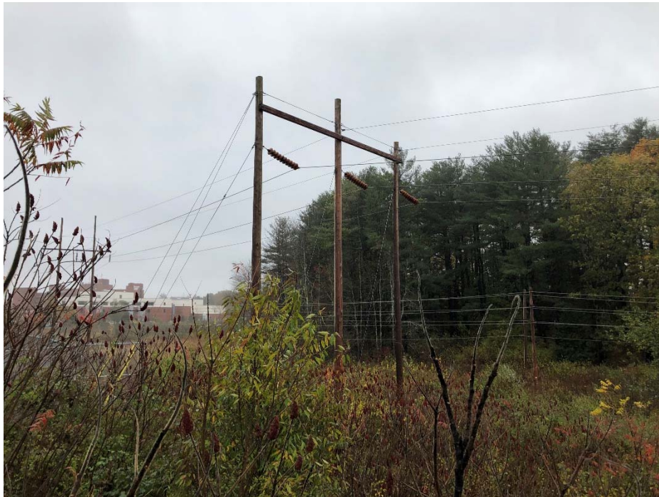
Photograph No. 3: Southwesterly view of proposed access and work area in the 100-foot wetland buffer of Wetland PW-11 for E194 Structure 34 to be replaced.
