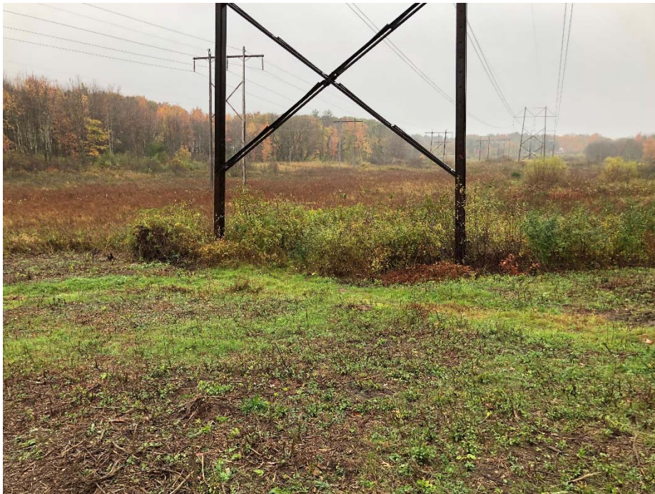
Photograph No. 14: Northeasterly view of 3135 Structure 105 to be replaced within the 100-foot wetland buffer of Wetland PW-6.
