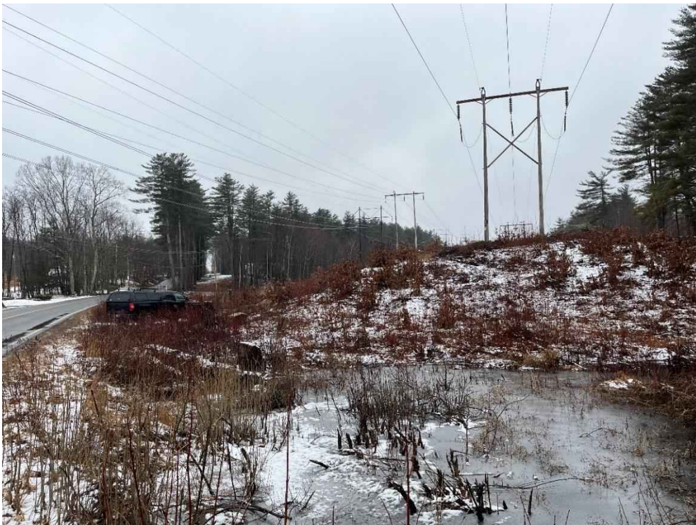
Photograph No. 32: Looking at proposed access and work pad location for H141 Structure 304 (right).
