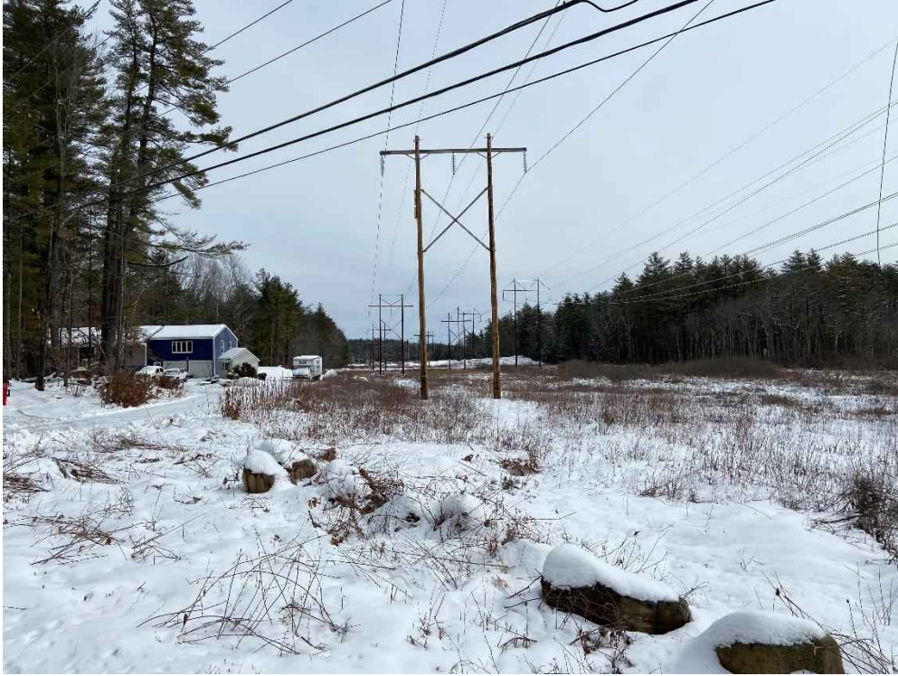
Photograph No. 31: Looking at proposed access and work pad location for R193 Structure 303 (far left), to the east across Fremont Road.
