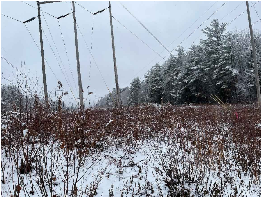
Photograph No. 23: Looking at proposed access and work pad location for H141 Structure 290.
