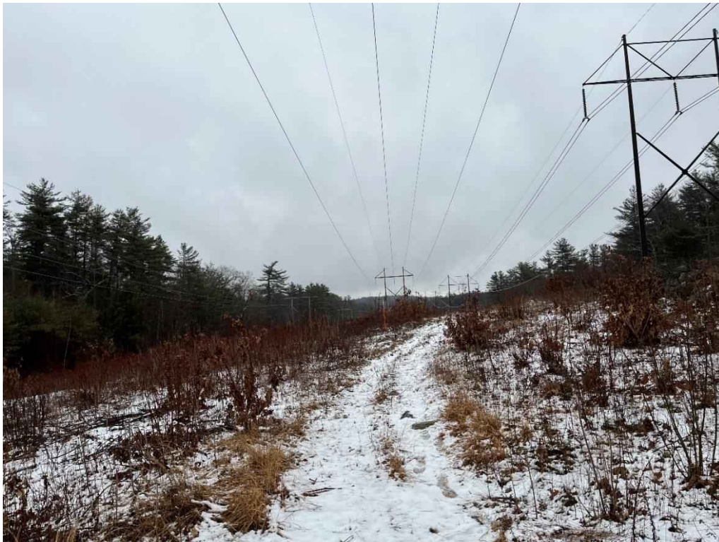
Photograph No. 36: Looking at proposed access to H141 Structure 275 and R193 Structure 307.
