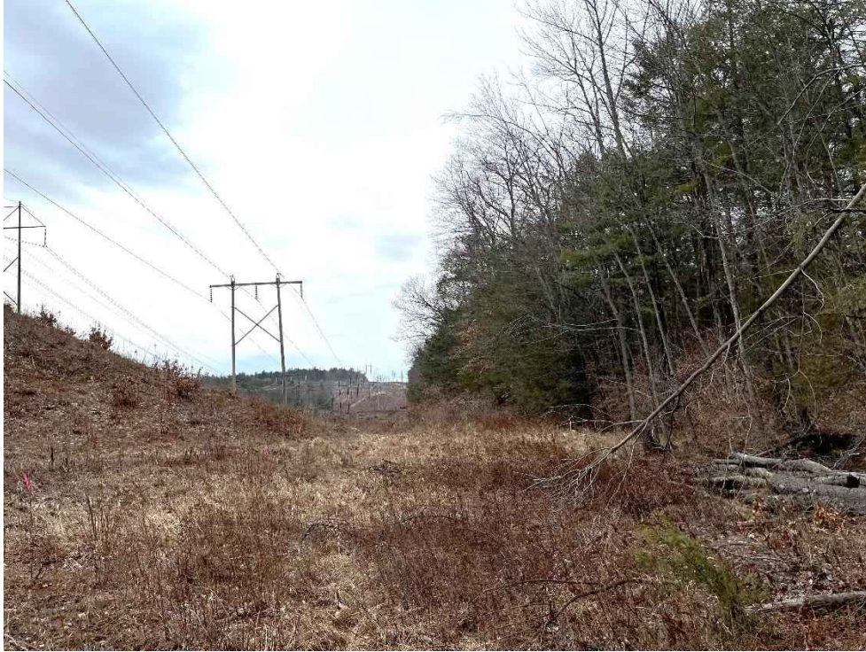
Photograph No. 3: Looking at proposed access and work pad location for R193 Structure 350.
