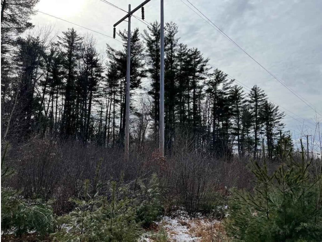
Photograph No. 37: Looking at proposed access and work pad location for H141 Structure 264.
