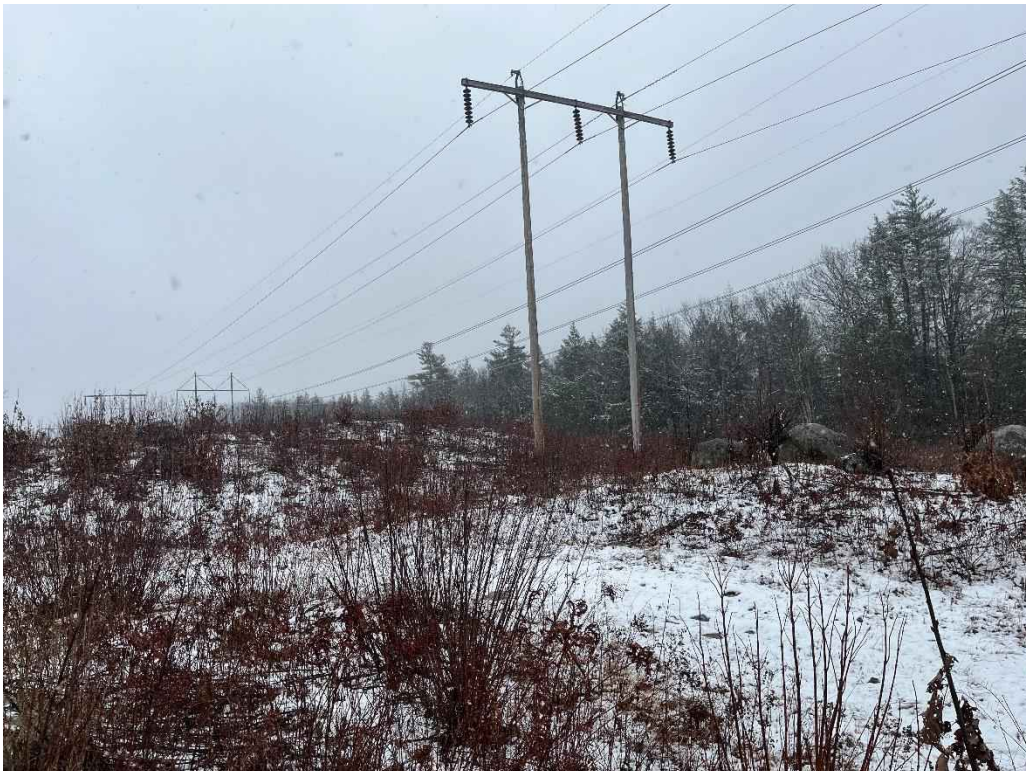
Photograph No. 28: Looking at proposed access and work pad location for H141 Structure 283.
