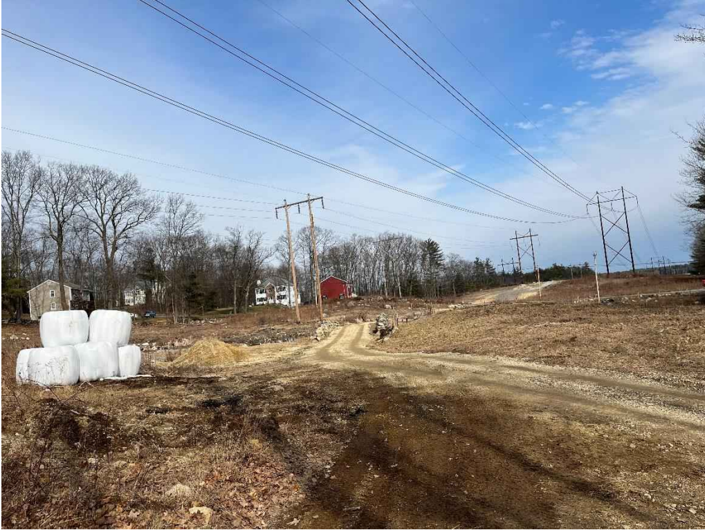
Photograph No. 9: Looking at proposed access and work pad location for H141 Structure 310 (left).
