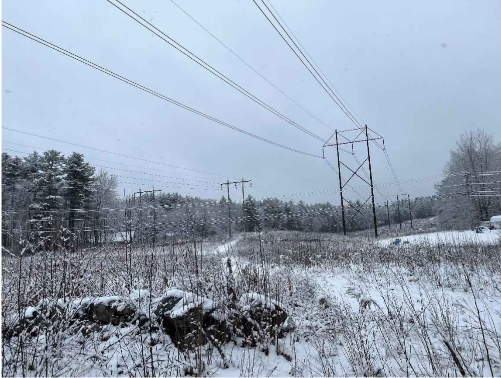
Photograph No. 19: Looking at proposed access and work pad locations for H141 Structure 292 (center) and R193 Structure 325 (left).
