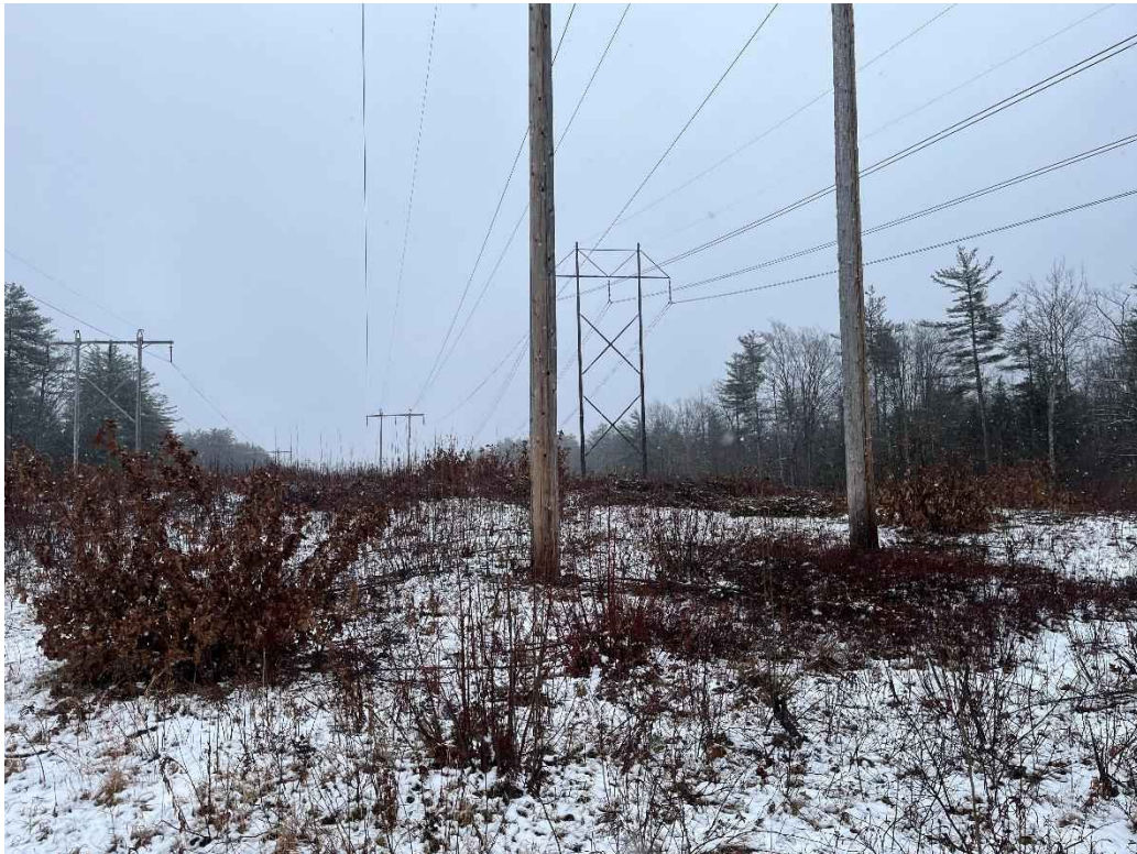
Photograph No. 30: Looking at proposed access and work pad location for H141 Structure 281.
