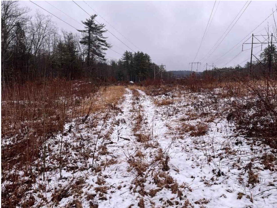
Photograph No. 34: Looking at proposed access and work pad locations for R193 Structure 306 and H141 Structure 274, adjacent to the left and right, respectively.
