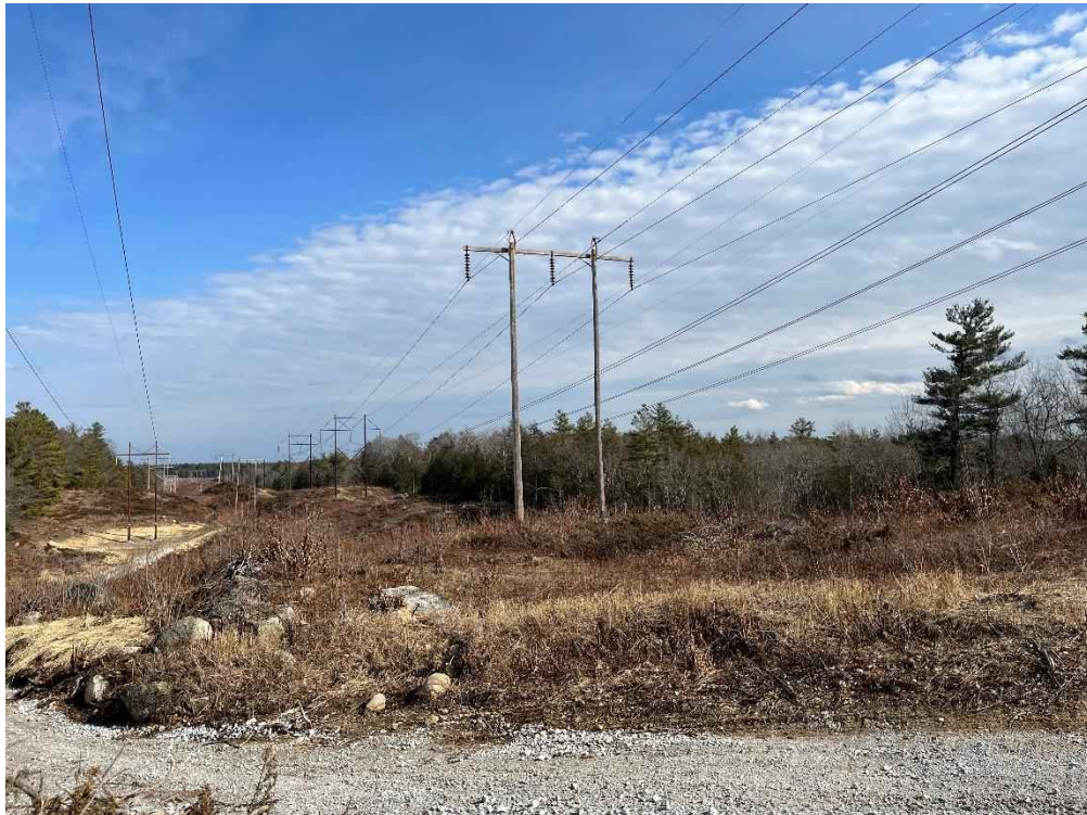
Photograph No. 10: Looking at proposed access and work pad location for H141 Structure 308.
