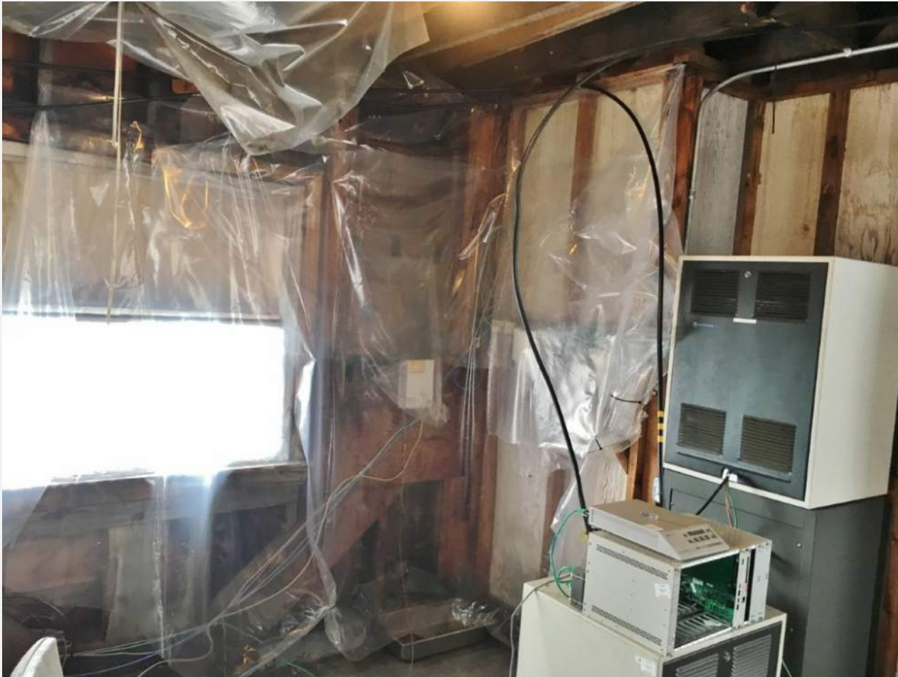
Federal Radios: Plastic Where Roof Leaked
