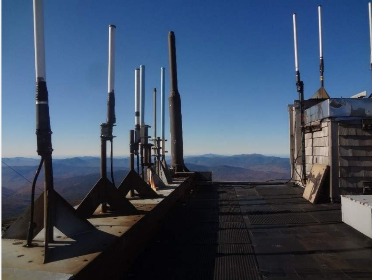
Penthouse Roof Antennas
