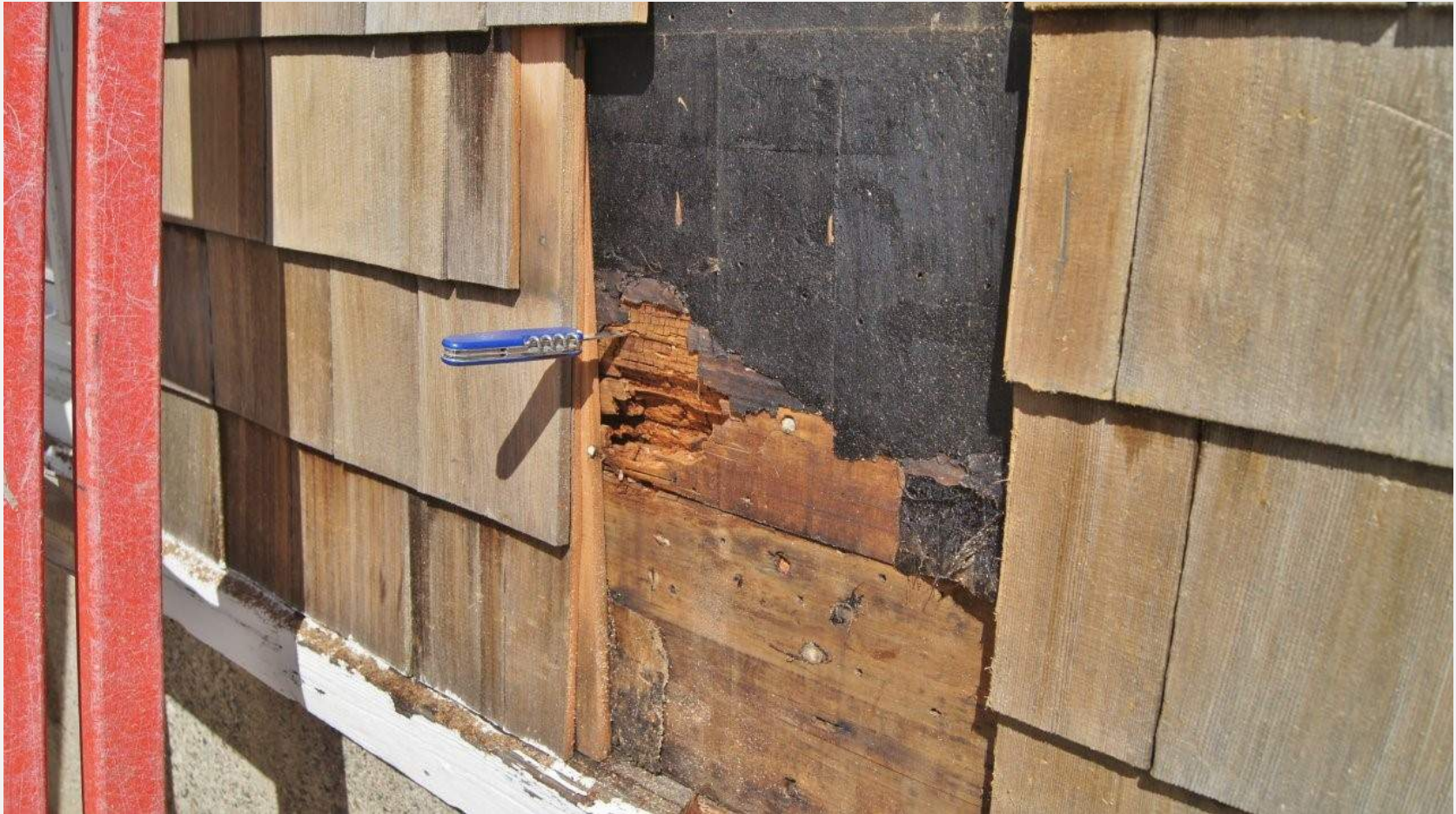
Water Damaged Wall Sheathing
