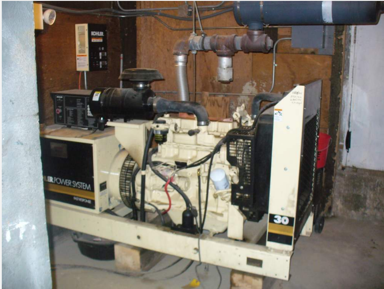
Basement Emergency Generator – Not Used Since After 2003 Fire
