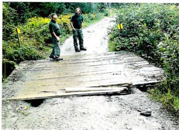
Figure 1, 2 and 3- Shows the broken boards on the bridges and the eroding approaches.
