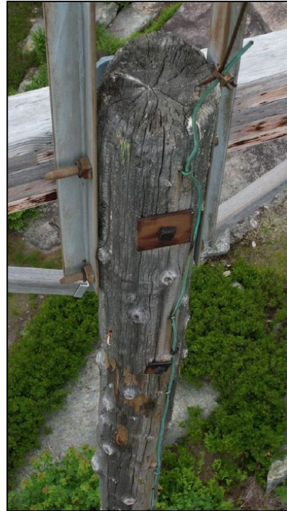
Line D121 Structure 80 – warped pole
