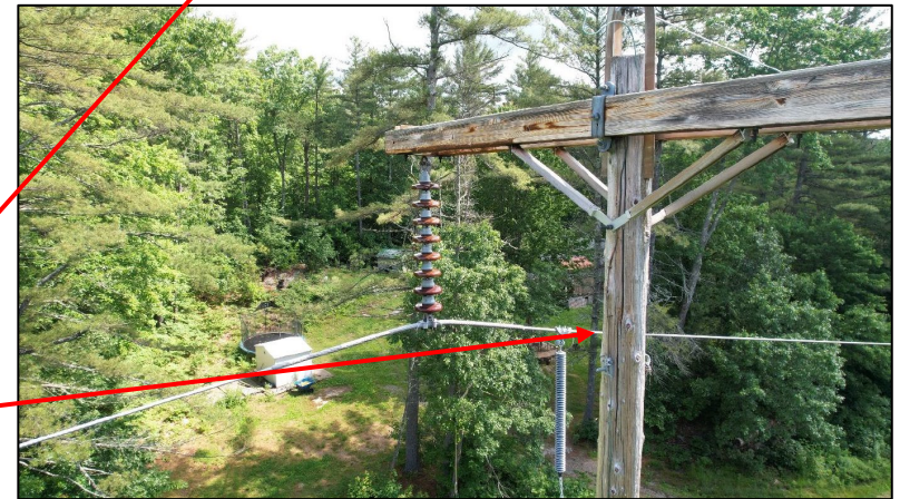
Line J114 Structure 22
