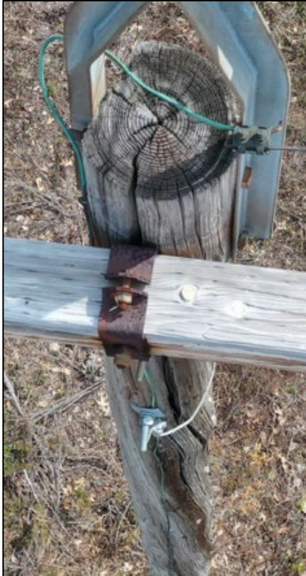
Line A126 Structure 192 – checking down pole affecting hardware
