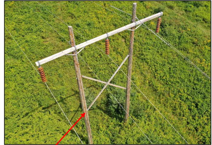
Line U181 Structure 52
