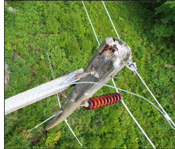
Line J114 Structure 5 – broken pole top, excessive rust on insulators, & splits
