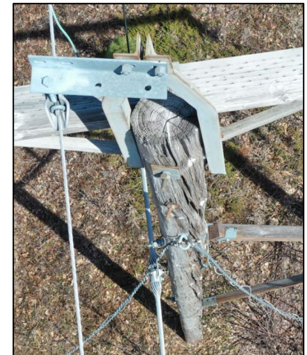
Line R193 Structure 261 – local buckling
