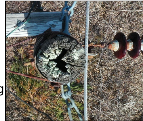
Line H141 Structure 290 Rusty insulator bells, large hole and top rot
