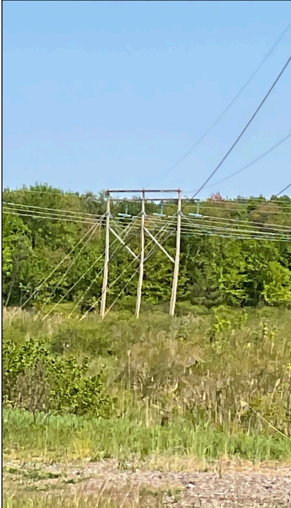
Line I158 Structure 73: Leaning and Bowing
