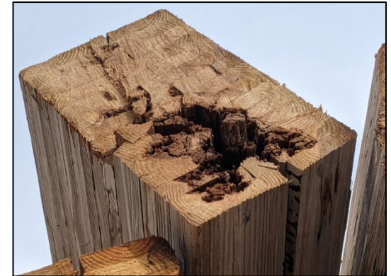
Phase I: Line G128 internal rot & insect damage
