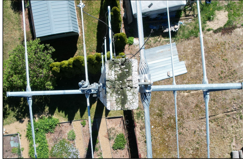
Line F162 Structure 18: Delamination
