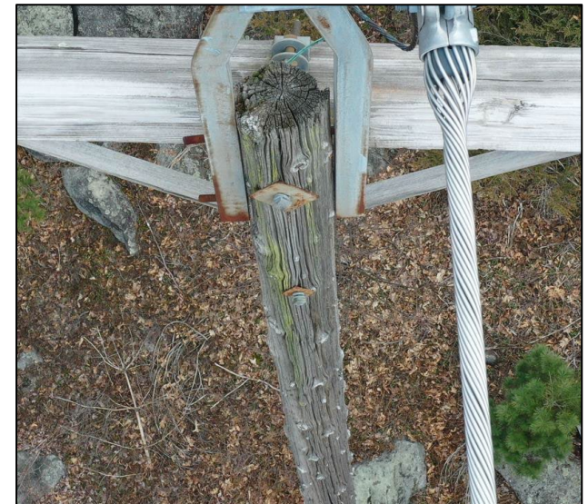
Line H141 Structure 160: Shell Rot on Pole Top Impacting Shieldwire Bracket
