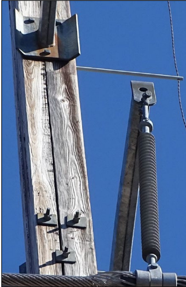
Line F162 Structure 17
