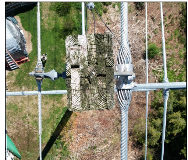
Line F162 Structure 23
