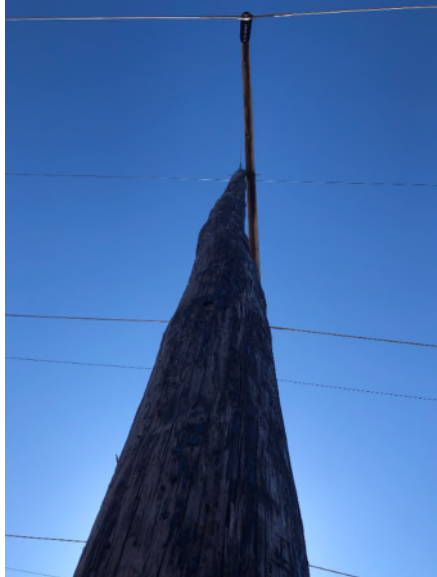
B-202 Structure 230 Wood Pole Crook/Sweep
