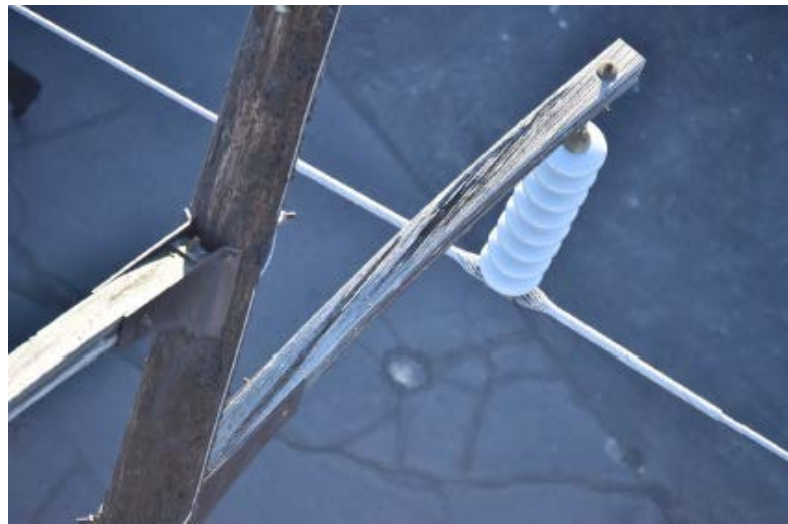
Deteriorated Davit Arm – Line 455-507
