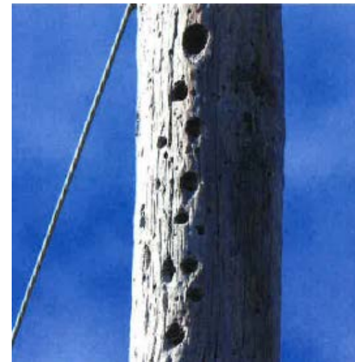
Woodpecker Damage – Line 352
