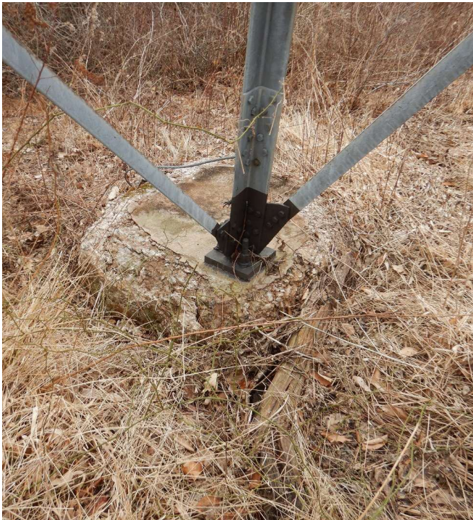
Structure 19095 – Foundation damage
