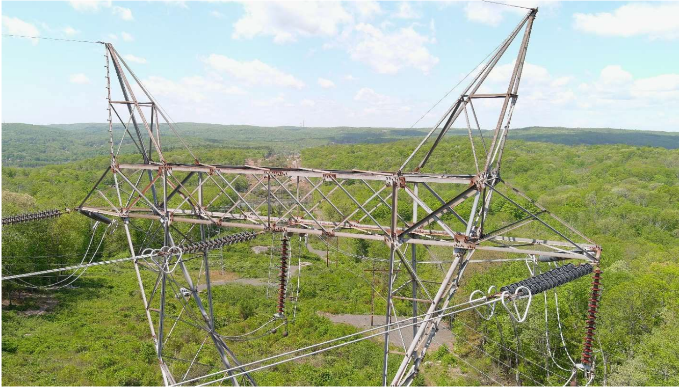
Structure 12054 – Rust on Hardware and Members
