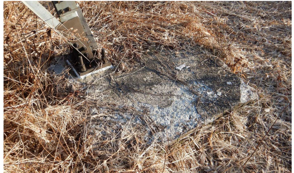
Structure 12066 – Foundation Damage
