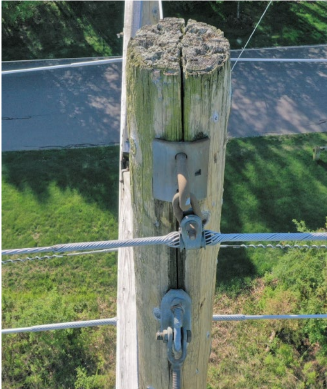
1208 Line – Pole Splitting and Woodpecker Damage
