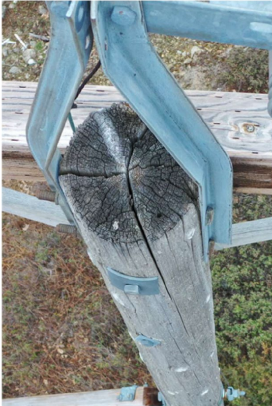
C196 Line – Top Rot and Splitting
