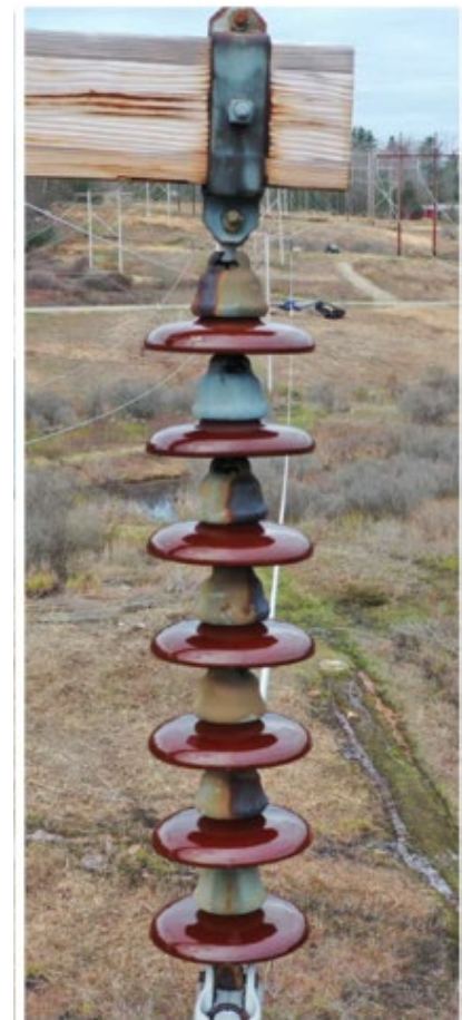
C196 Line – Damaged and Rusted Insulator 9
