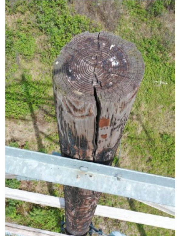
389 Line – Top Pole Splitting
