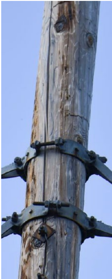
Line 389 – Pole Splitting and Breaking
