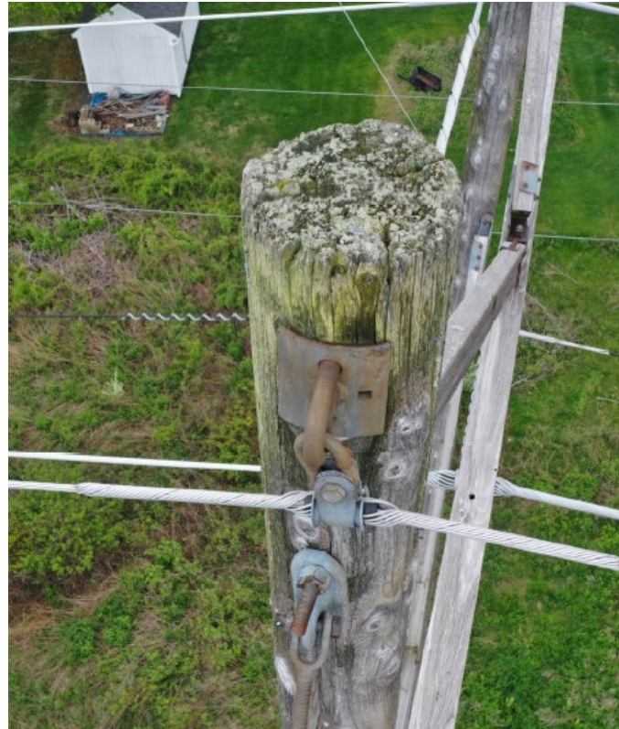
1208 Line – Top Rot and Cracking
