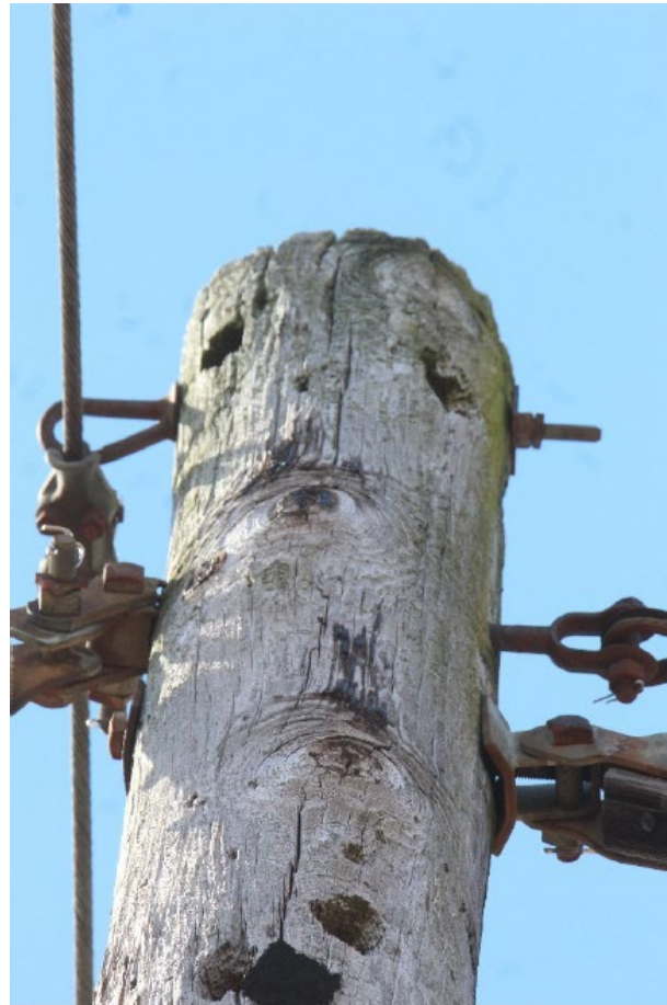
Line 1280 – Woodpecker Damage and Top Rot
