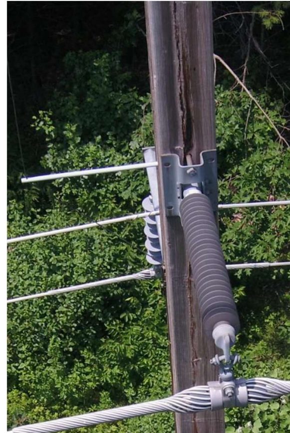
Side Crack – V191 Line, Structure #13
