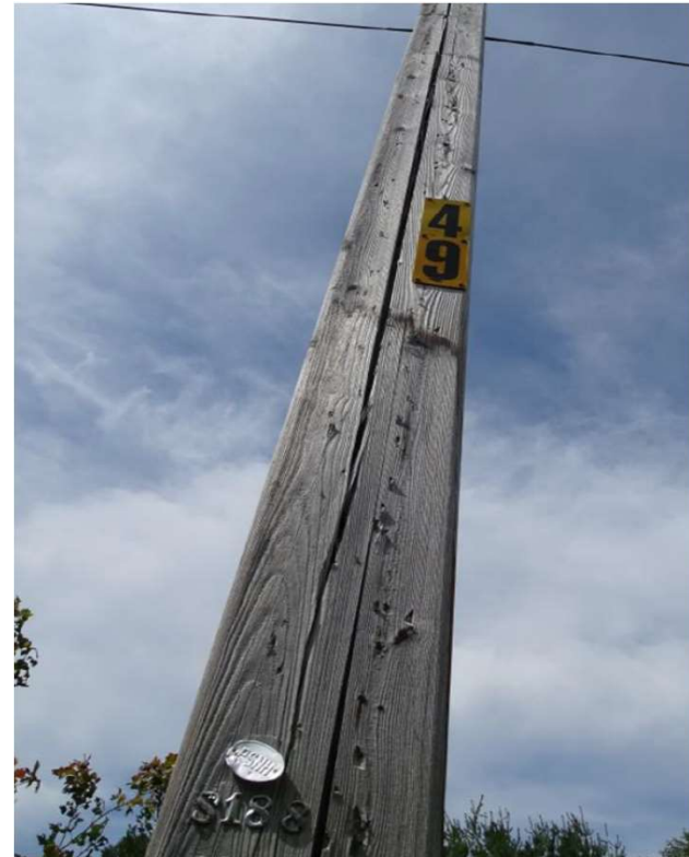
Side Crack – S188 Line, Structure #49
