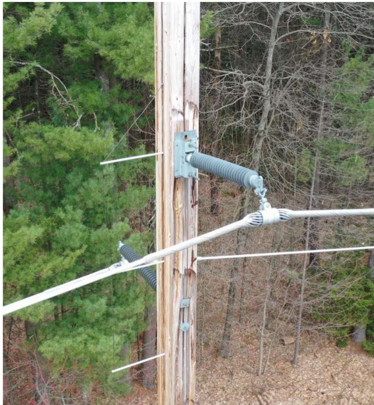
Cracking Laminate Structure – V191 Line, Structure #47
