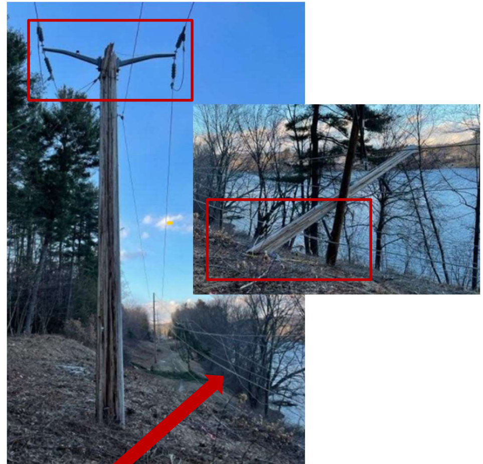
V191 Line Structure 47 – 115-kV Wires on the Ground due to Laminated Wood Structure Failure
