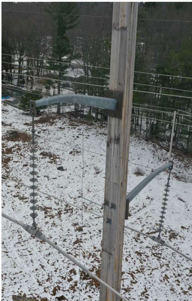
Side Cracks – R187 Line, Structure #21
