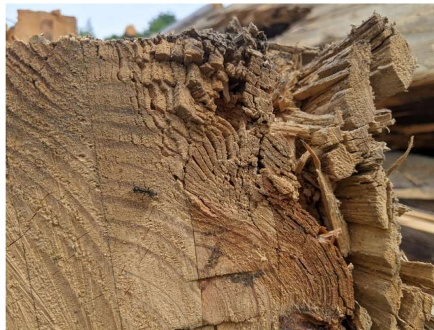
L175 Line – Degraded Laminated Wood Structures, Internal Rot, Side Cracking, Insect Damage
