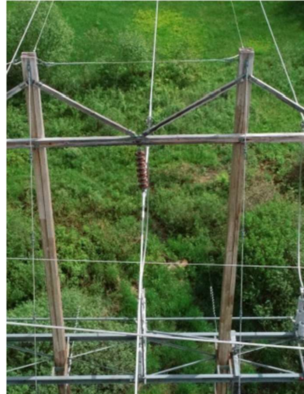
Cracking Laminate Structure – A152 Line, Structure #70
