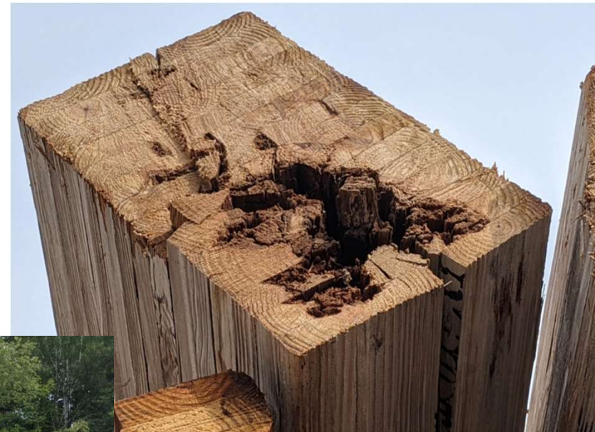
Above: G128 Line – Slide Cracking, Rot and Insect Damage
