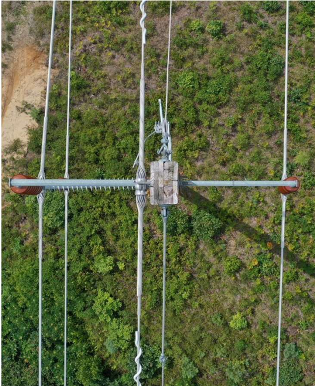
Pole Top Cracking – A152 Line, Structure #46
