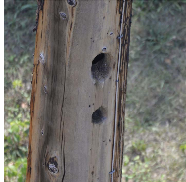
Structure 34209: Woodpecker Damage (medium)
