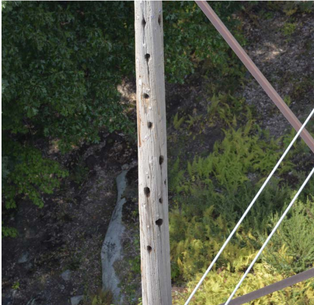
Structure 34005: Woodpecker Damage
