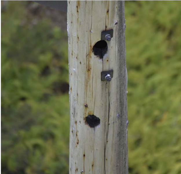
Structure 34038: Woodpecker Damage (heavy)
