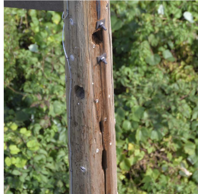
Structure 34156: Woodpecker Damage
