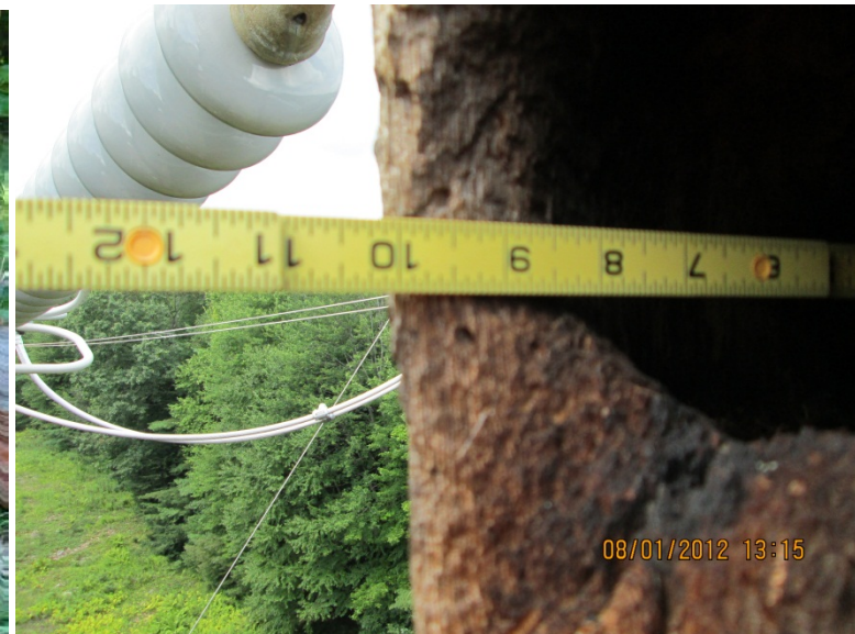
Depth of Woodpecker Damage
