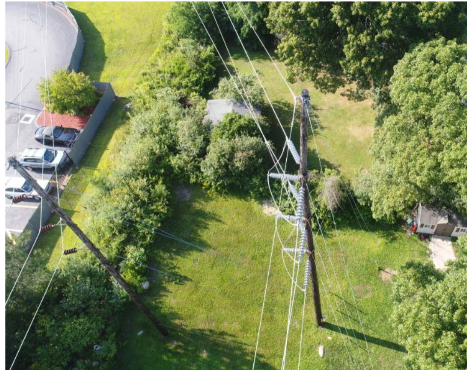
Typical Wood Structure on Line 455-507
