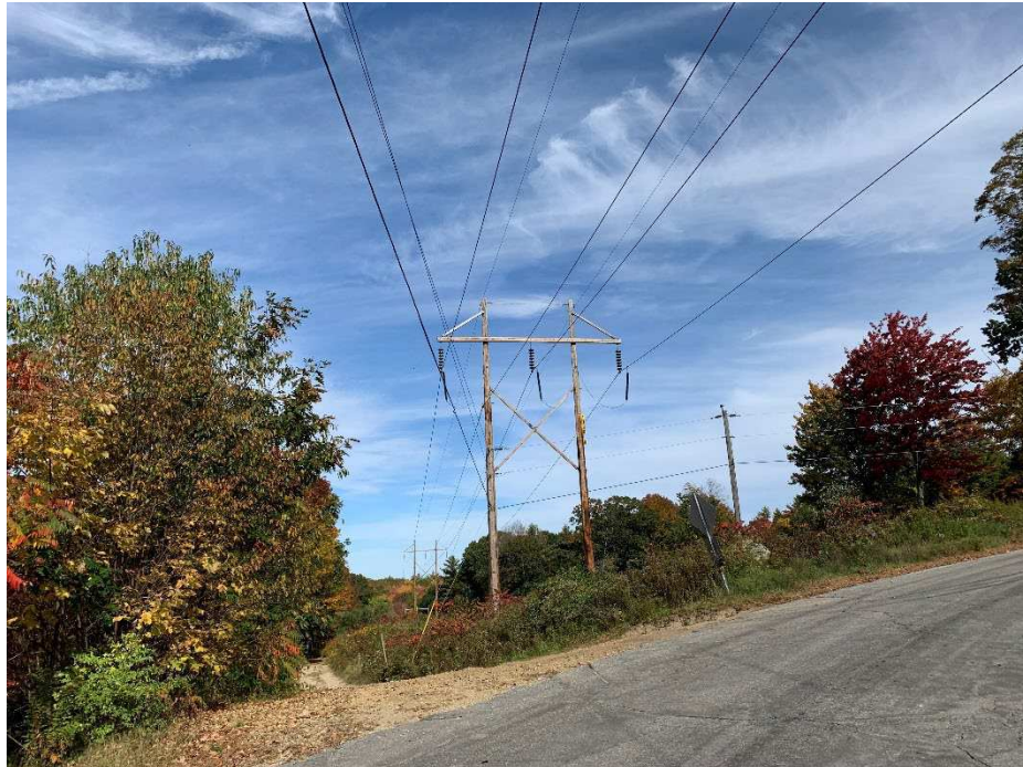
Photograph No. 24: Northwesterly view of entrance into the right-of-way and Structure 8 from Bigelow Hill Road.
