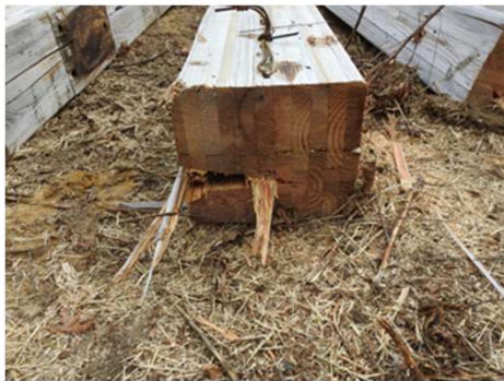
Large Crack – X116 Line, Structure #133
