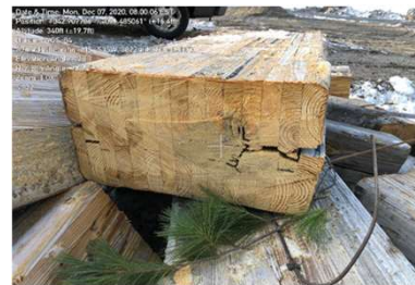
Rot and Splitting at Joints – K105 Line, Structure #32
