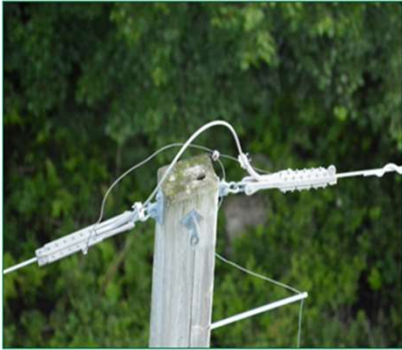
Rotten Pole Top – K105 Line, Structure #20
