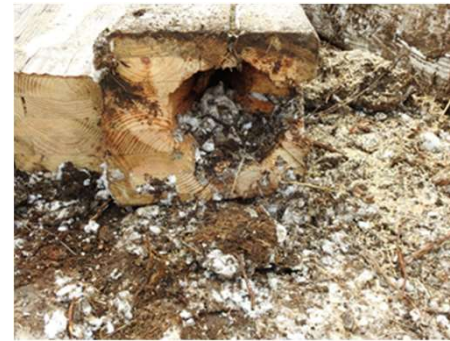
Extensive Rot – Z119 Line, Structure #137
