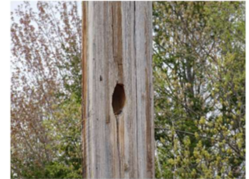
Crack Through Woodpecker Hole – L175 Line, Structure #139
