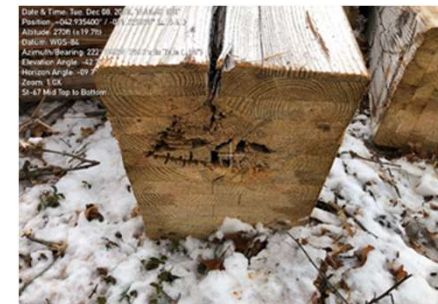
Extensive Rot – K105 Line, Structure #67
