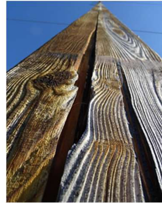
Side Crack – L175 Line, Structure #122
