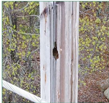
Woodpecker Damage – G128 Line, Structure #57
