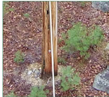
Woodpecker Damage – G128 Line, Structure #63
