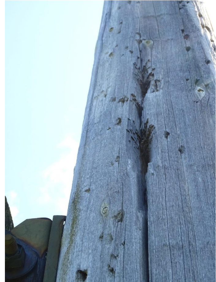
379 Line – Pole Splitting and Woodpecker Damage
