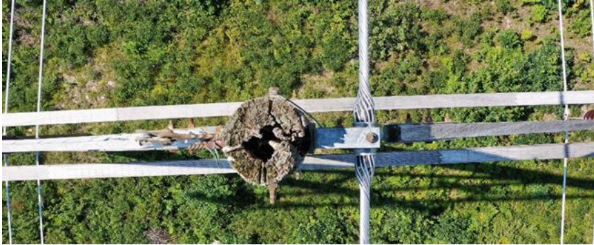
373 Line – Top Rot and Splitting
