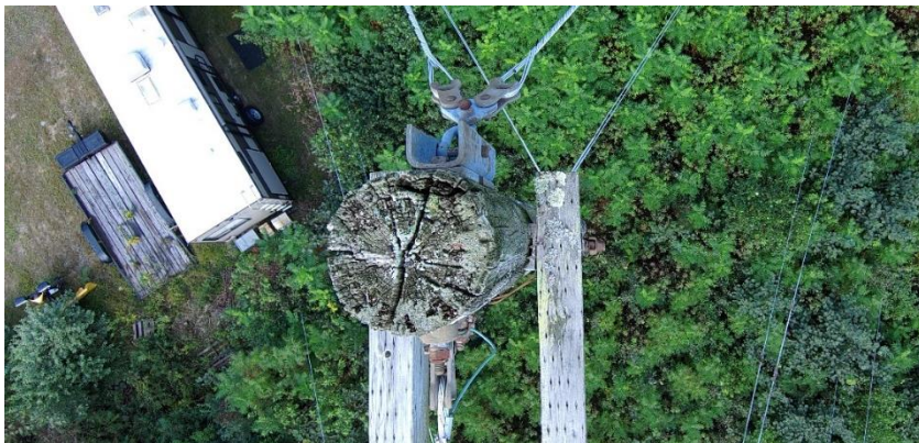
326 Line – Top Splitting and Cracking
