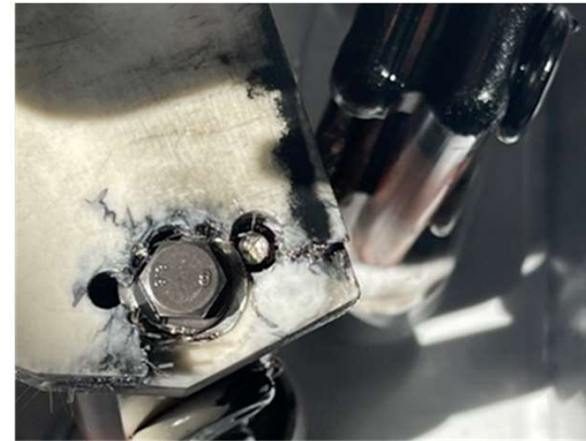
TB154 - Evidence of arcing within LTC cabinet
