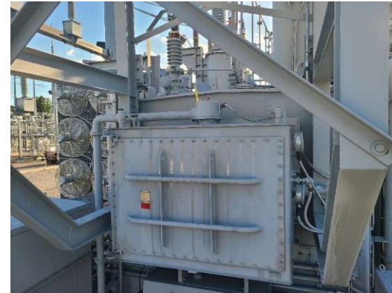
TB154 - Evidence of active oil leak on LTC door
