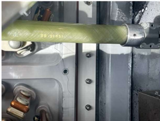
TB154 – Barrier board comprised and cracked
