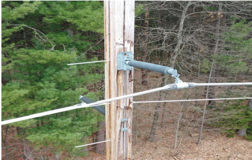
Cracking Laminate Structure – V191 Line, Structure #47
