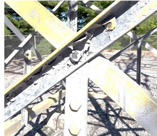
Steel member deterioration
