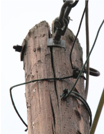
1751, Structure #3-331 Split Pole Top, Cracks, Decay
