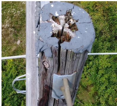
240-510, Structure #197 Pole Top Rot
