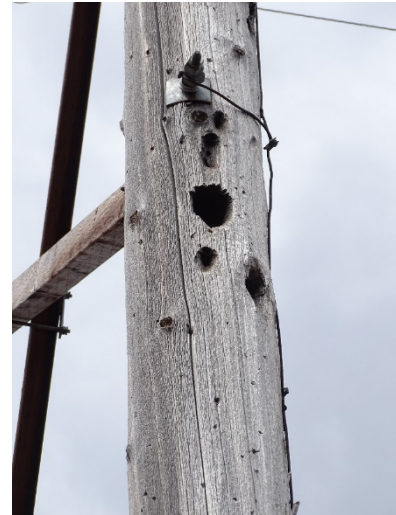
D121, Structure #46 Woodpecker Damage
