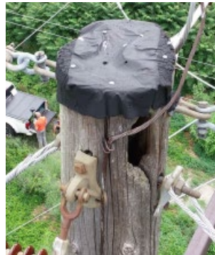
342-603, Structure #101 Woodpecker Damage
