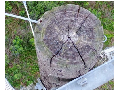
456-522, Structure #2 Pole Top Split
