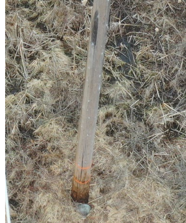
Q171 Structure 34 cracking, decay, structure leaning
