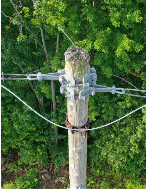
1783 Structure 16073 Split pole top, woodpecker damage
