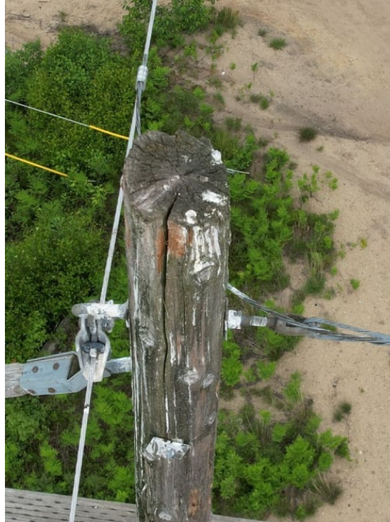
P106 Structure 56 Pole top rot, chunk missing out of pole top
