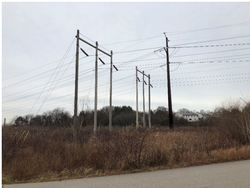
Photograph No. 4: View of Structures U181-20 & E194-20 to be replaced within Wetland PW-23. Timber matting will be used to minimize and prevent rutting in the wetland.
