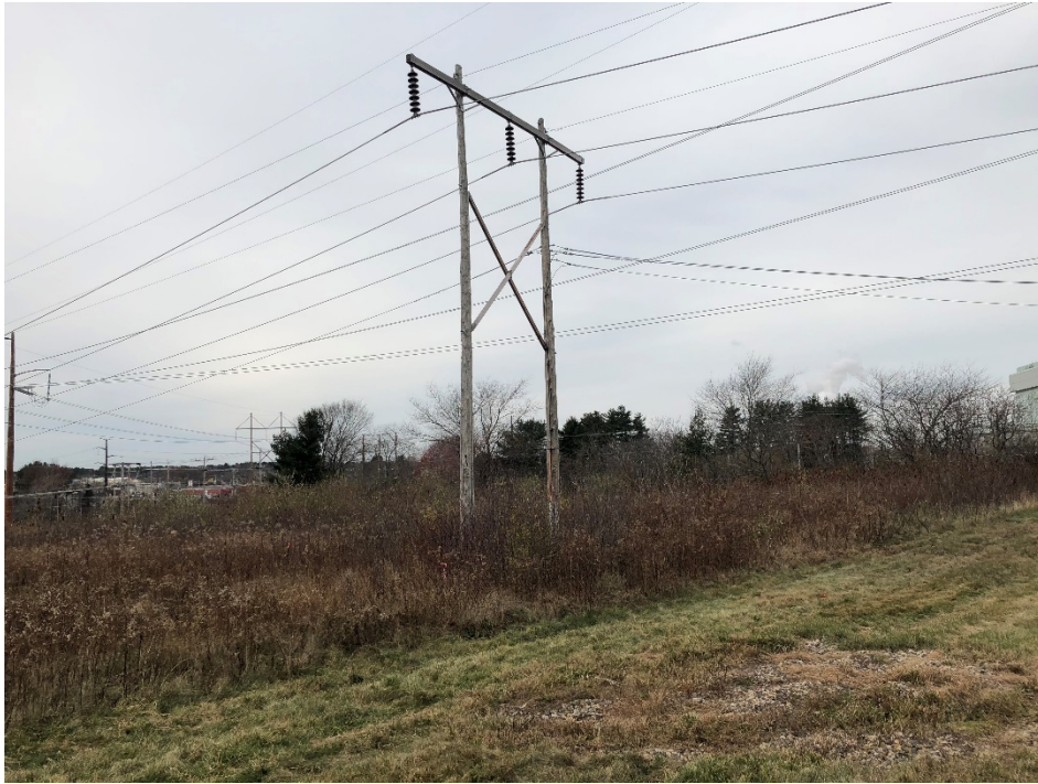
Photograph No. 13: View of Structure U181-2 to be replaced off Gosling Road.
