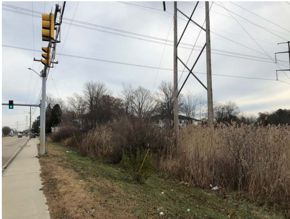
Photograph No. 10: View of Structure U181-12 to be replaced within Wetland PW-27 off Gosling Road. Timber matting will be used to minimize and prevent rutting in the wetland.
