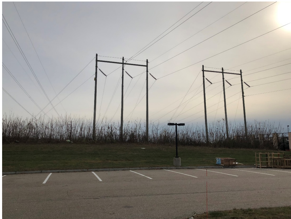
Photograph No. 6: View of Structures U181-17 & E194-17 off Echo Avenue to be replaced.
