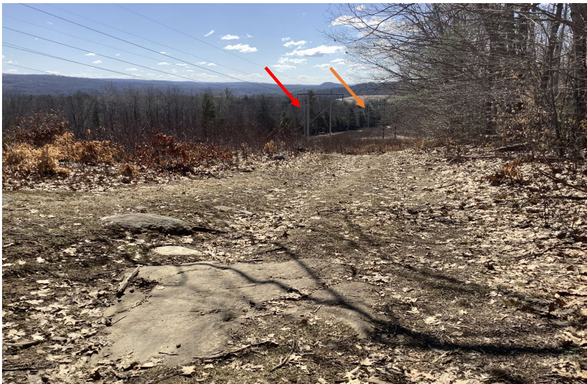
Photo 8: Representative view southeast of the utility ROW with V182 Line Structures 247 (red arrow) and 246 (orange arrow) in the background in Franklin.
