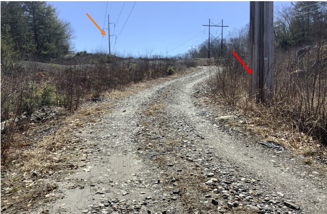
Photo 2: View south of the existing access road at the base of Structure 253 (red arrow) with Structure 252 in the background (orange arrow) in Franklin.
