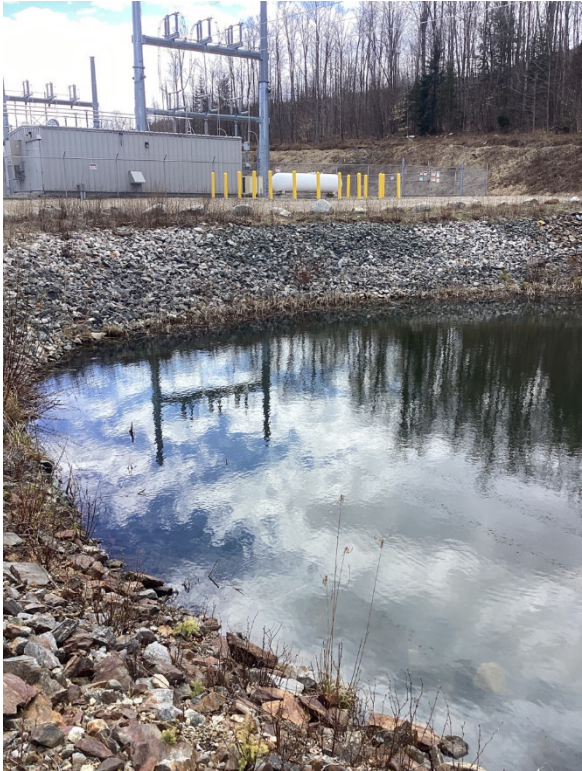
Photo 16. View of Paris Substation and existing stormwater basin. Stantec, May 5, 2022.
