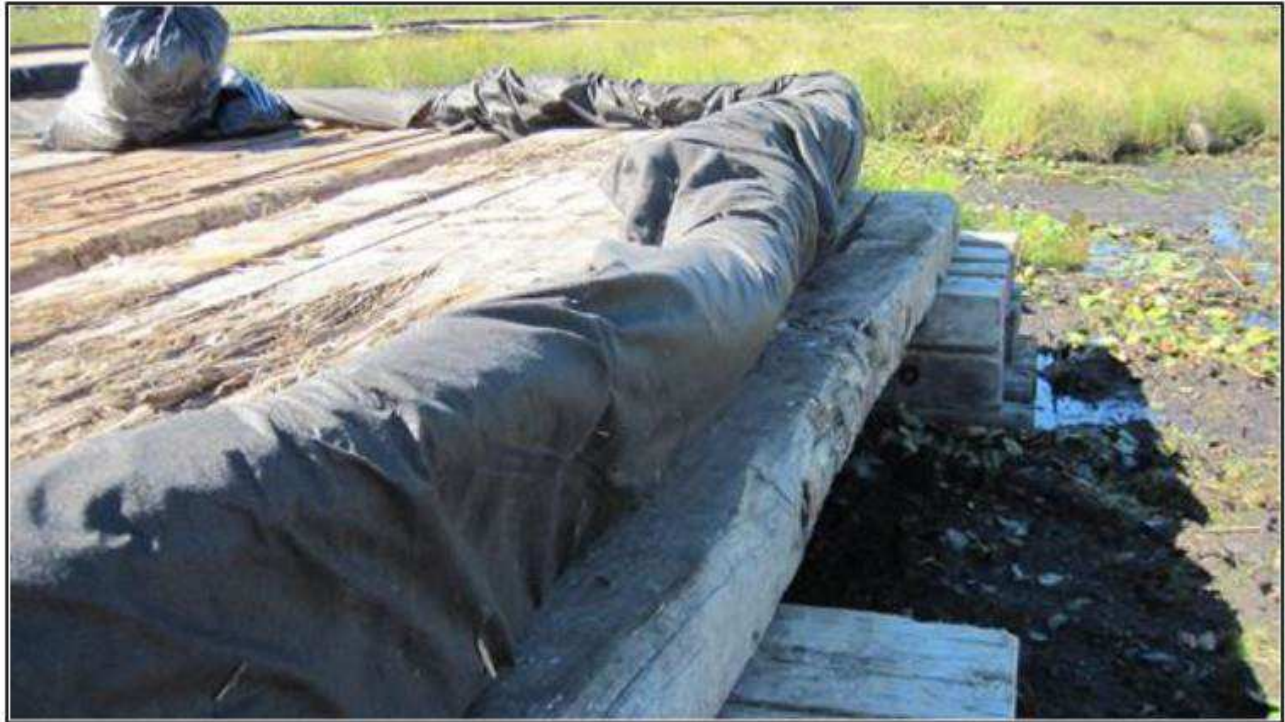
Constructing a swamp mat bridge span reduces direct impacts to the wetland surface and maintains aquatic organism passage through the construction area. The number of necessary swamp mats may be reduced using this method.
